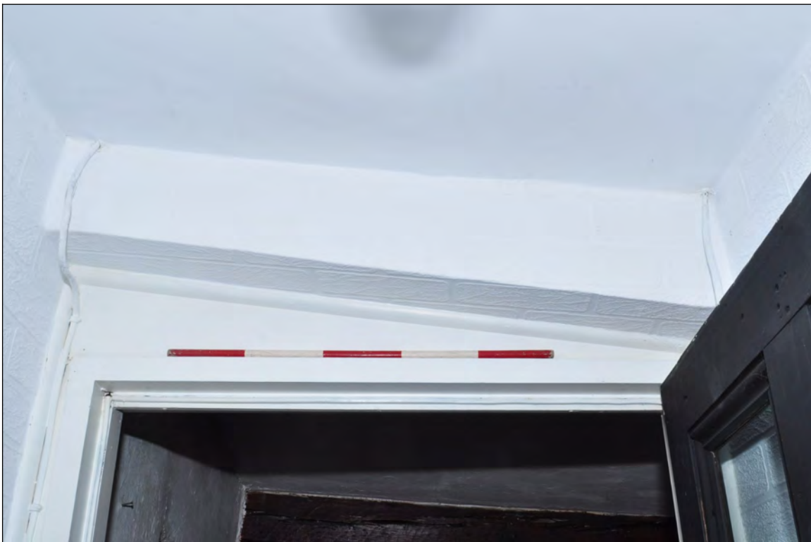
Photo 4: Beam 1 (firehood bressumer?), boxed in over doorway from shop (before work). Looking north-east.
