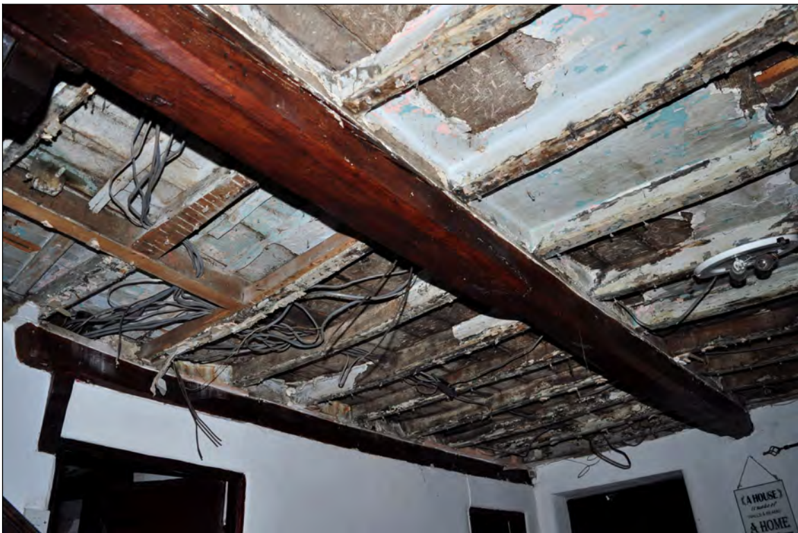
Photo 20: Underside of joists and boards either side of beam 2 (exposed for repairs). Looking south-east.
