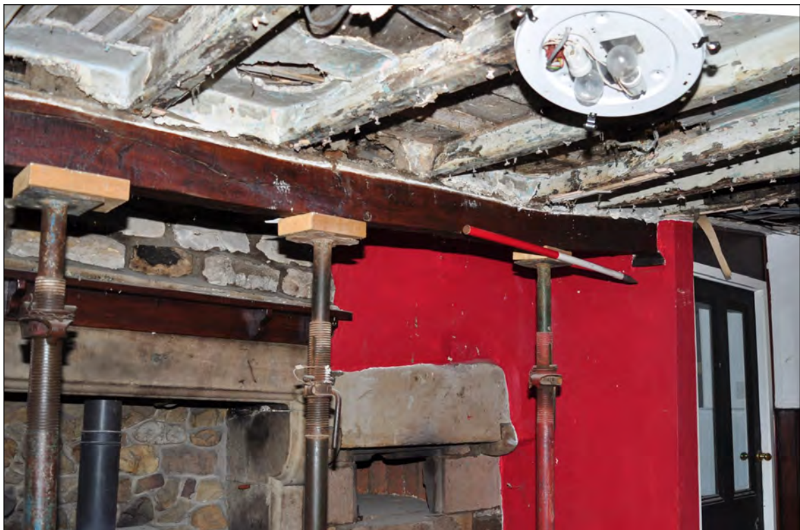
Photo 6: Beam 1 (firehood bressumer?), adjacent to fireplace in lounge/living room (exposed for repairs). Looking west.
