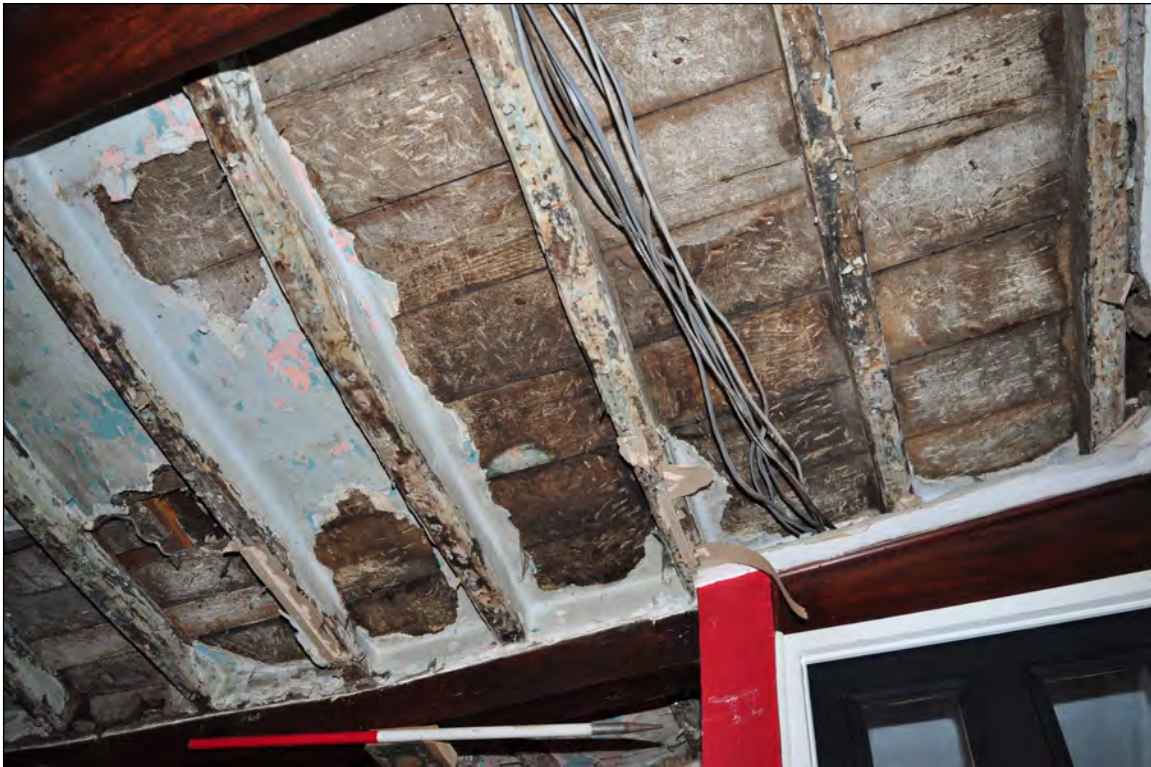
Photo 17: Underside of joists and boards between Beams 1 & 2 (exposed for repairs). Looking south-west.
