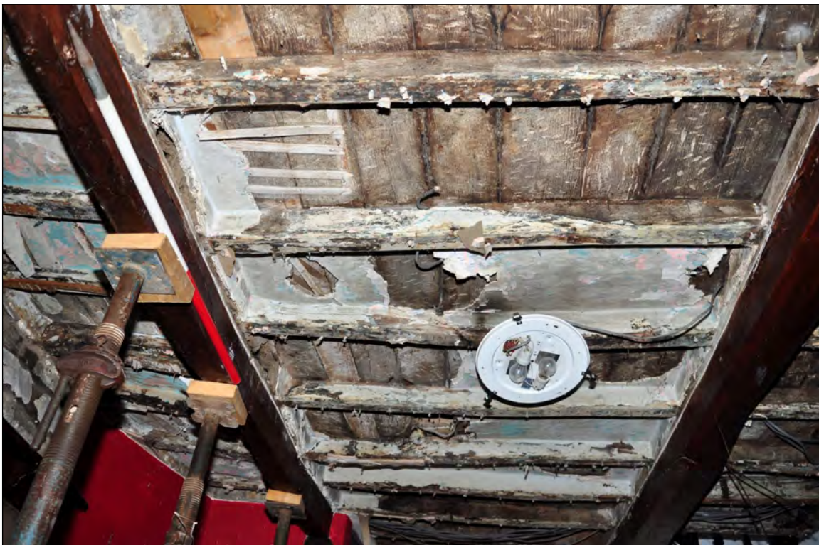
Photo 18: Underside of joists and boards between beams 1 & 2 (exposed for repairs). Looking north-west.
