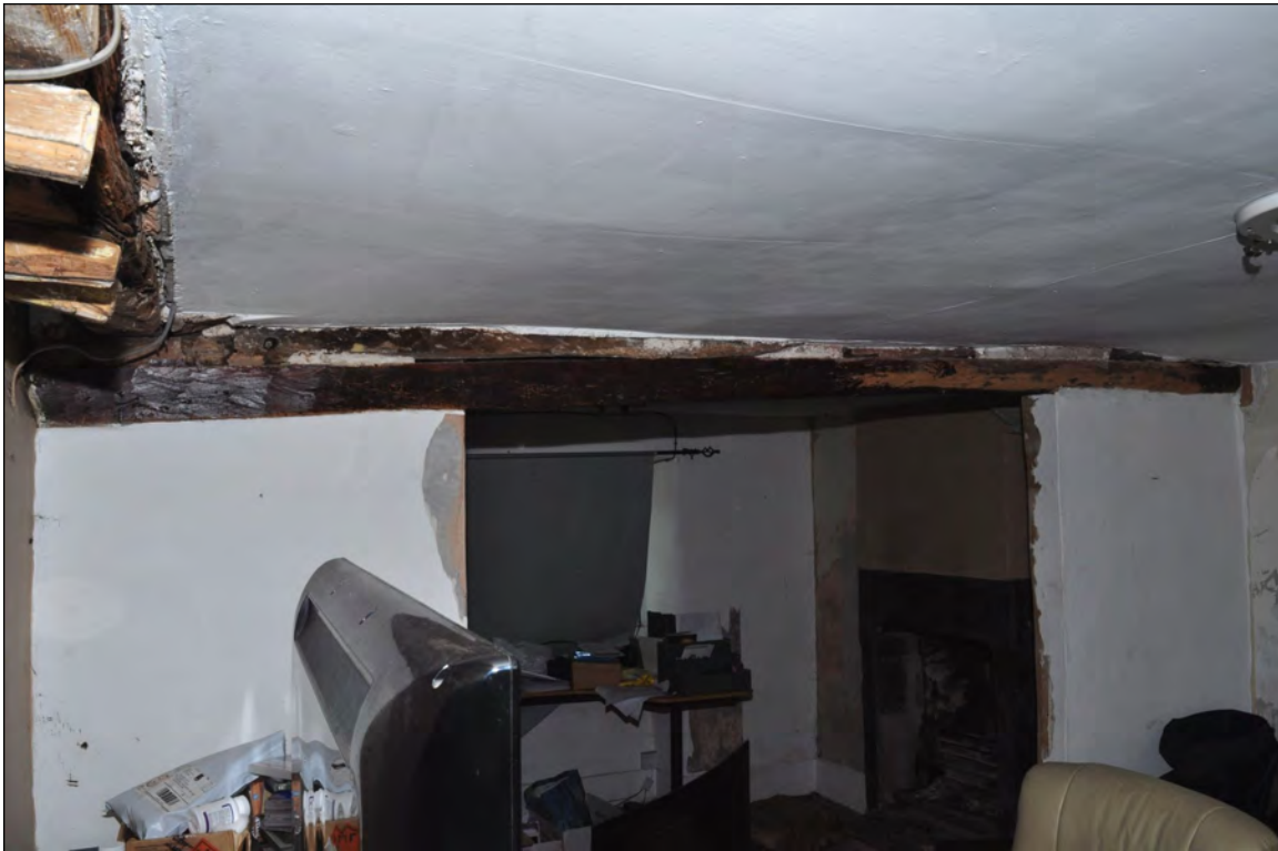
Photo 31: Beam 5, over partition between dining room and study (before work). Looking north.
