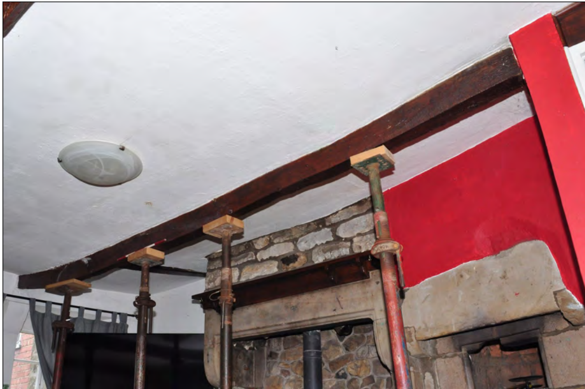
Photo 1: Beam 1 (firehood bressumer?), adjacent to fireplace in lounge/living room (before work). Looking south.
