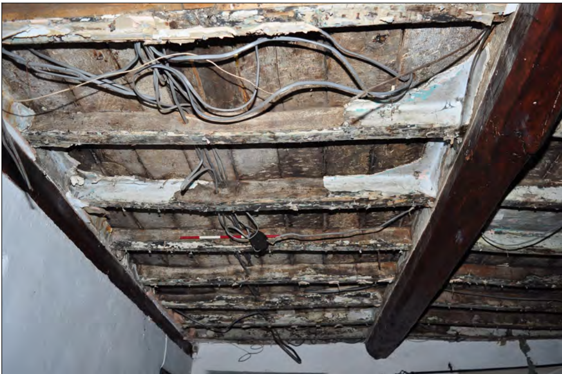
Photo 26: Underside of joists and boards, between beams 2 and 3 (exposed for repairs). Looking south-east.
