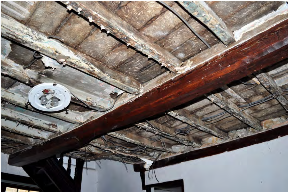
Photo 21: Underside of joists and boards to either side of beam 2 (exposed for repairs). Looking north.
