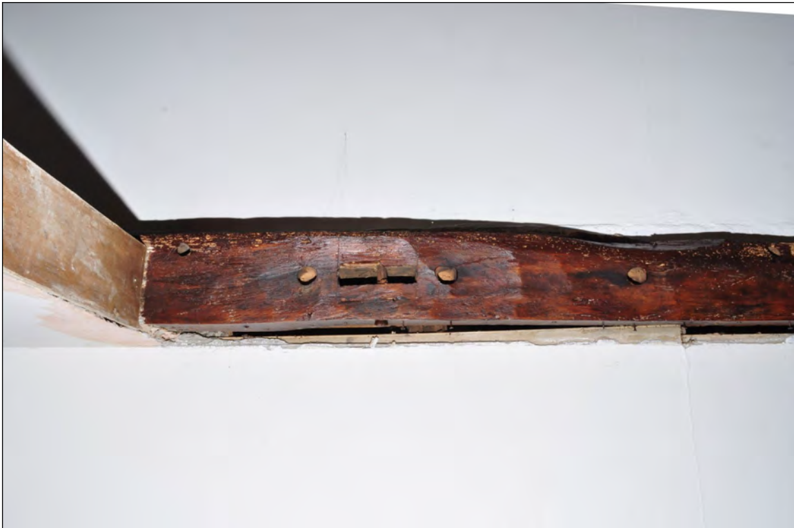
Photo 33: Beam 5, over partition between dining room and study (before work) South-west end.
