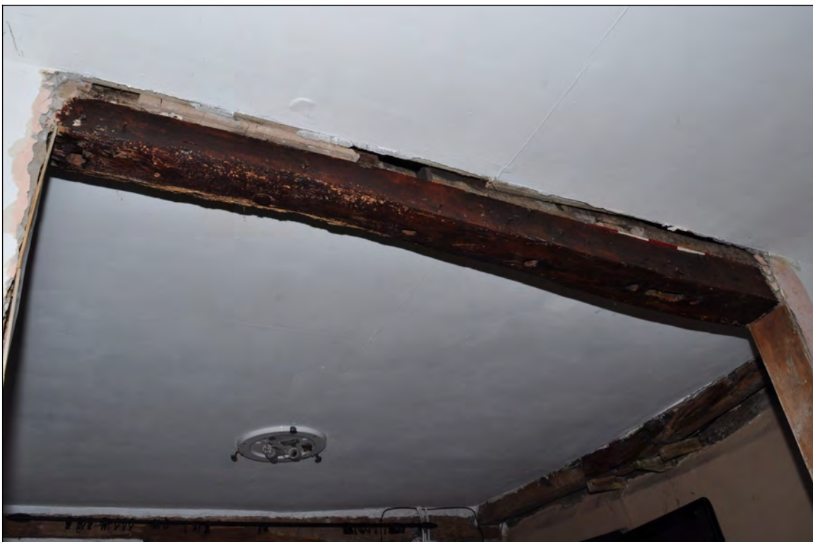
Photo 32: Beam 5 over partition between dining room and study (before work). Looking south.
