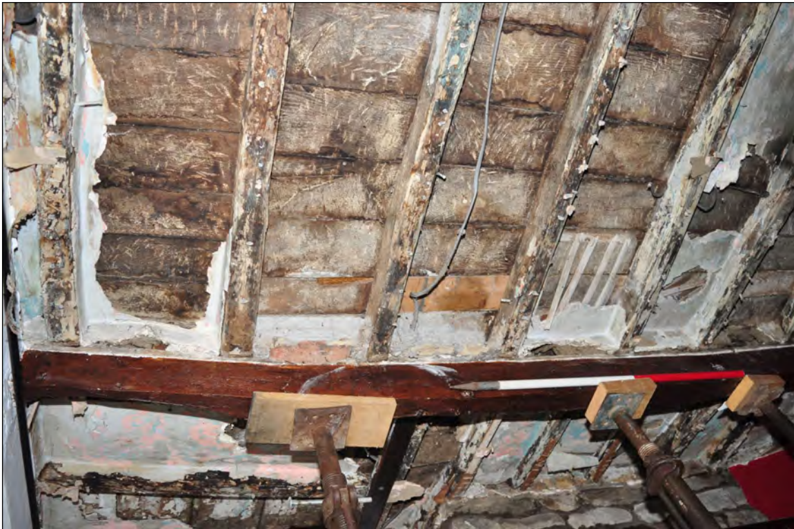
Photo 19: Underside of joists and boards between Beams 1 & 2 (exposed for repairs). Looking south-west.
