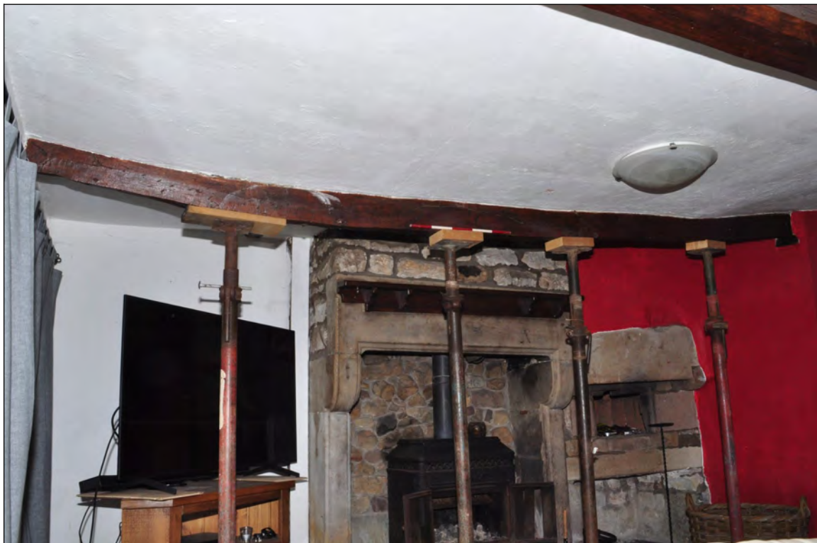
Photo 2: Beam 1 (firehood bressumer?), adjacent to fireplace in lounge/living room (before work). Looking south-west.
