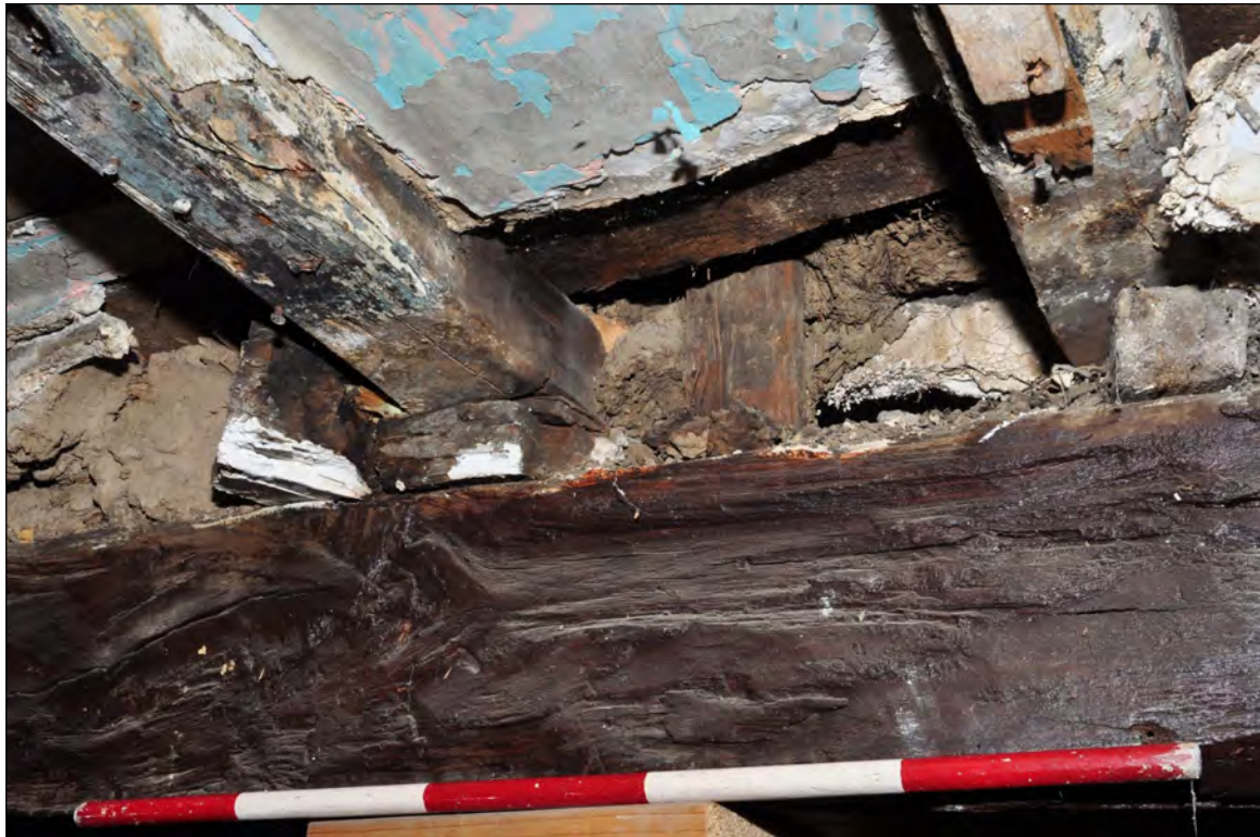
Photo 7: Detail of beam 1, looking east. Note oak joists resting on packing, suggesting that they are secondary, and foot of riven stud to first floor partition, with daub infill – perhaps part of firehood (exposed for repairs)
