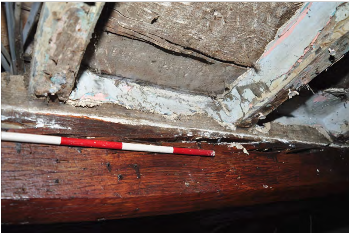
Photo 22: Detail of beam 2 and joists on south-west side (exposed for repairs). Looking north.
