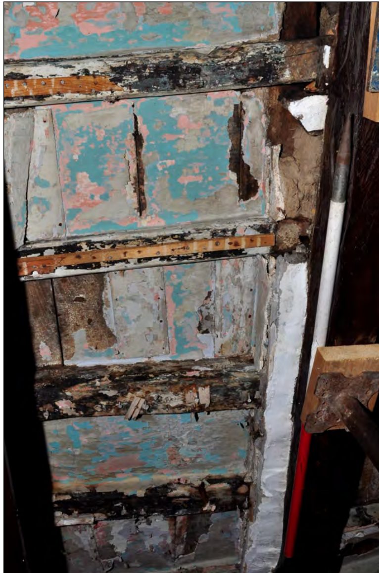
Photo 8: Underside of joists and boards between Beam 1 and fireplace (exposed for repairs). Paint and limewash indicate ceiling was not always underdrawn. This may be infill within former firehood. Looking north-west.
