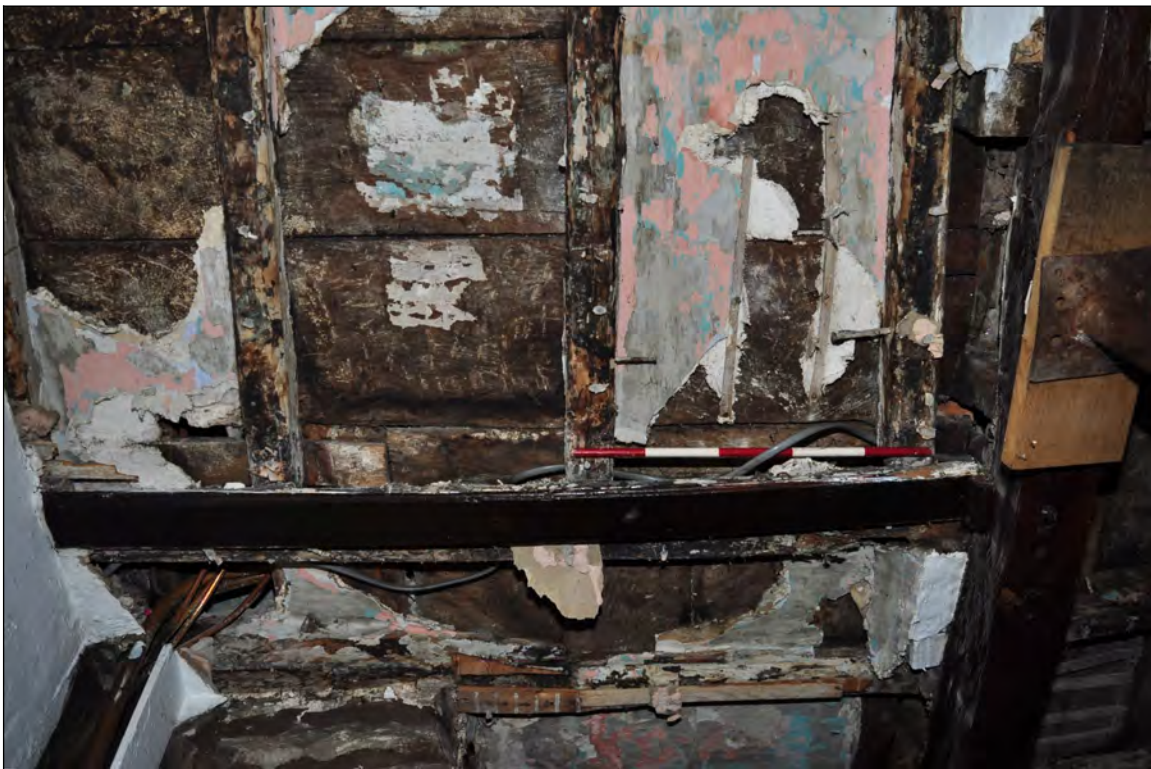
Photo 10: Underside of short cross-beam and floor in south corner of living room (exposed for repairs). Note different orientation of joists, perhaps indicating this part of the first floor lay outside the firehood. Looking north-west.
