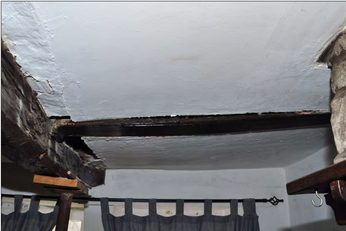
Photo 9: Short cross-beam, spanning between Beam 1 and end wall, by fireplace (before work). Looking south-east.
