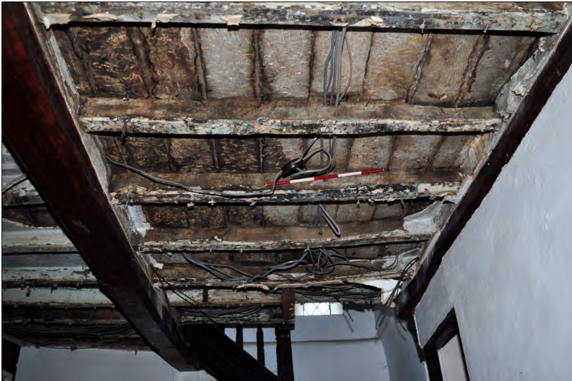
Photo 25: Underside of joists and boards, between beams 2 and 3 (exposed for repairs). Looking north-west.
