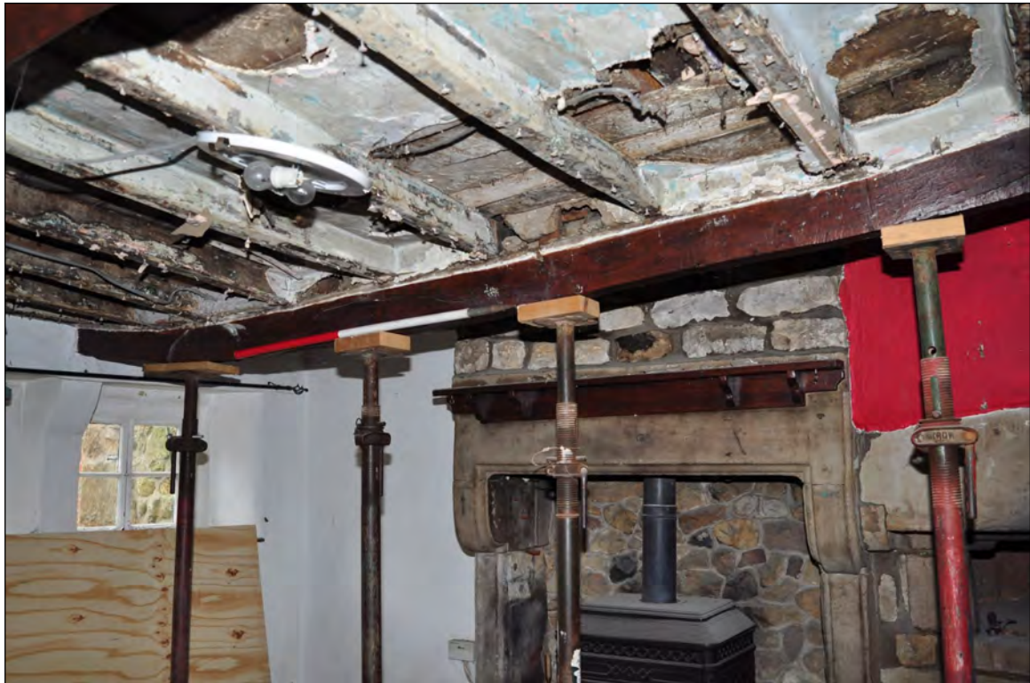
Photo 5: Beam 1 (firehood bressumer?), adjacent to fireplace in lounge/living room (exposed for repairs). Looking south.
