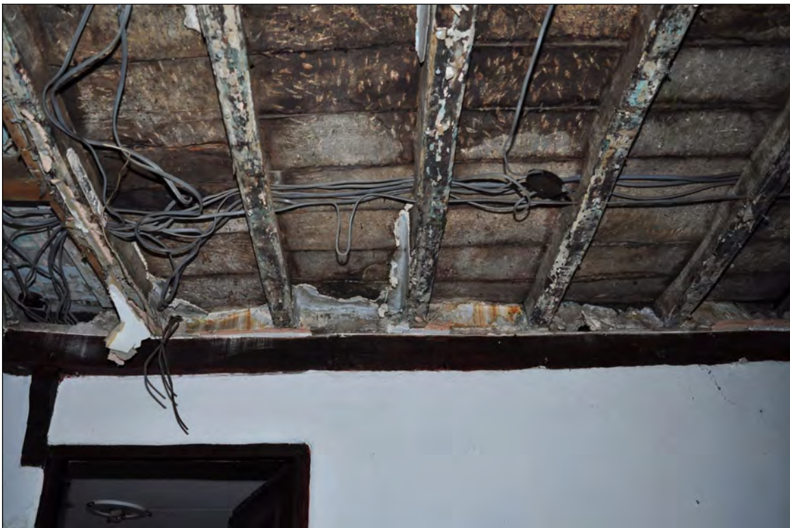
Photo 24: Underside of joists and boards, next to beam 3 (exposed for repairs). Looking north-east.
