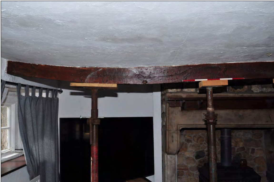
Photo 3: Beam 1 (firehood bressumer?), adjacent to fireplace in lounge/living room (before work). Looking south-west.
