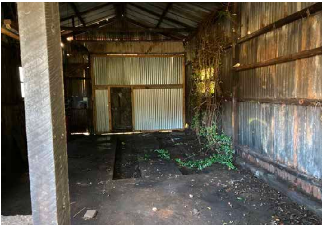
Photo 8: Interior of dilapidated corrugated iron shed.
