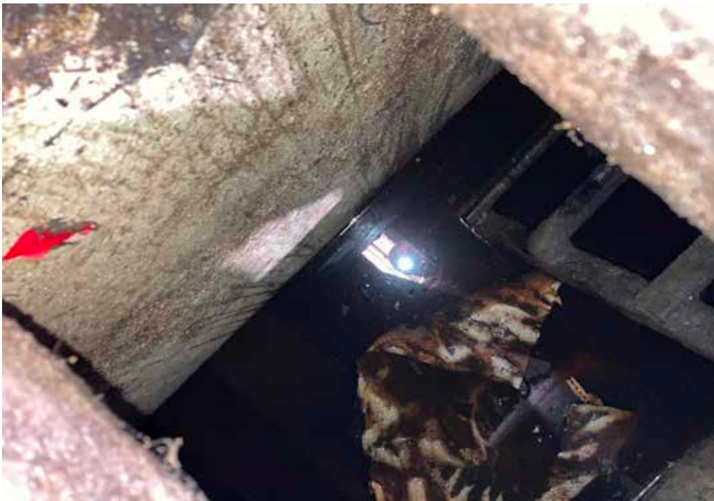
Photo 10: Interior of vehicle inspection pit showing cement render side walls, steel access ladder, standing water, and some discarded fabric.
