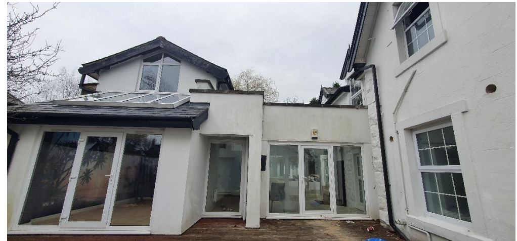
B1 – newer section linked with the main structure via a flat roof section.
