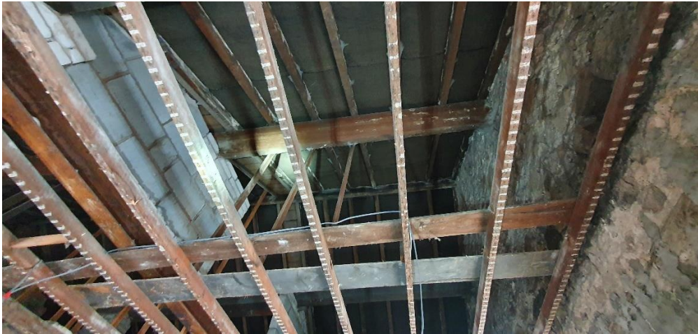
B1 – internal roof structure showing the lack of loft space (pictured above).
