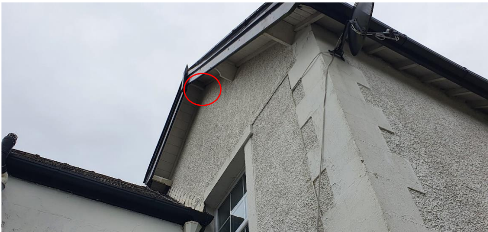
B1 – possible bat access point as pre the previous ecological survey present along the western elevation (pictured above).
