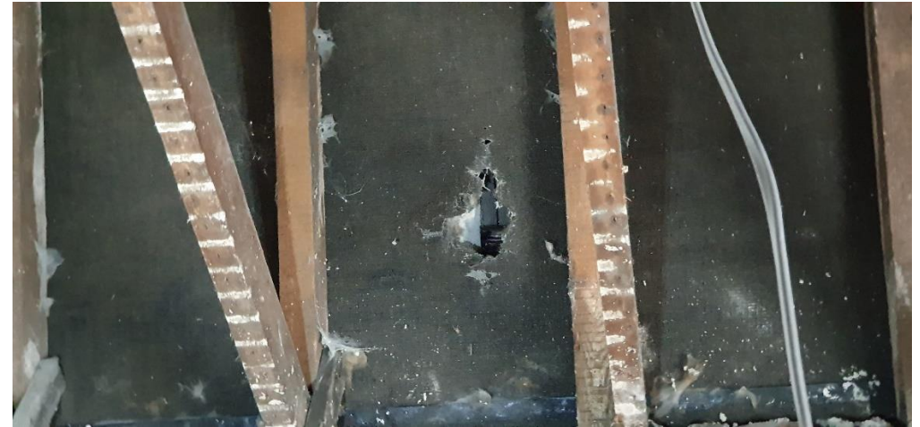
B1 – example of a rip in the roof lining as per the previous ecological survey (pictured above).
