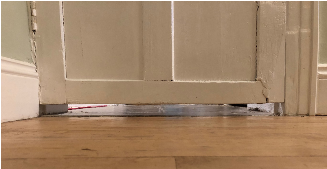
Fig. 1 – photograph showing damage to the base on an existing door, caused by past alterations to the bottom rail.
