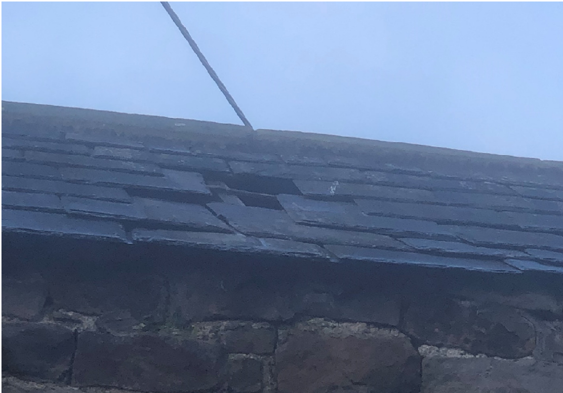
Fig. 2 – damage to the roof of the outbuilding caused by recent storms.
