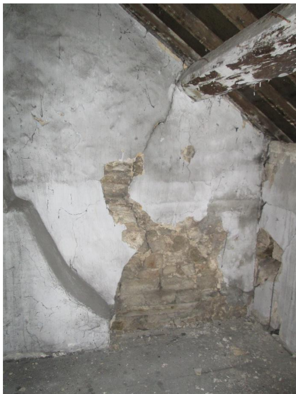
Photo 10 – Crack in left hand gable wall
