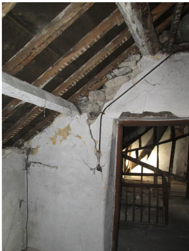
Photo 11 – Crack in internal dividing wall
