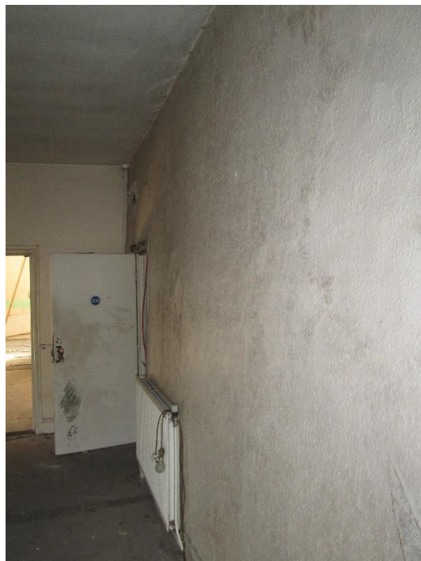
Photo 16 – Leaning wall in rear right-hand room
