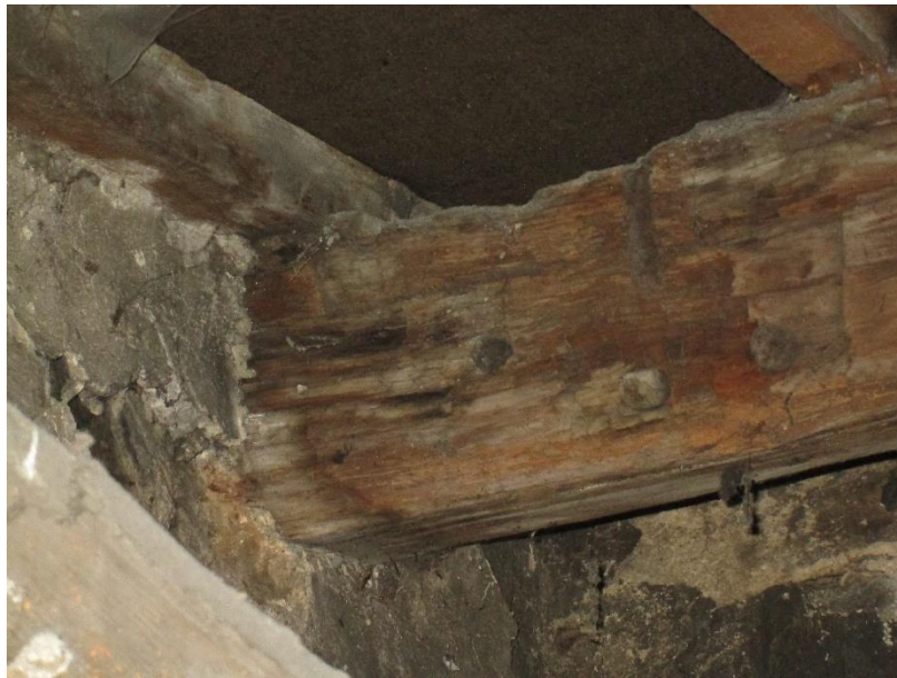
Photo 7 – Decay to timber purlin at wall bearing
