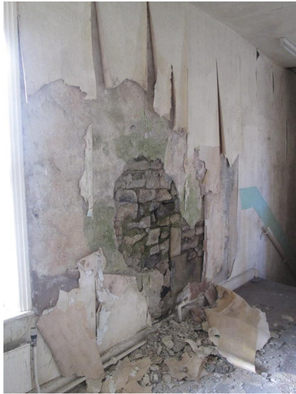
Photo 17 – Damaged and detached plaster
