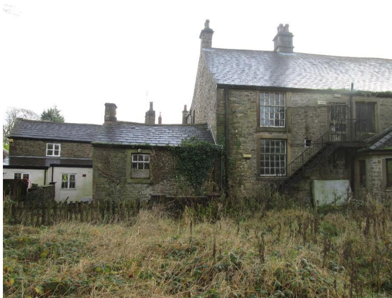
Photo 23 – Sag in kitchen ridge
