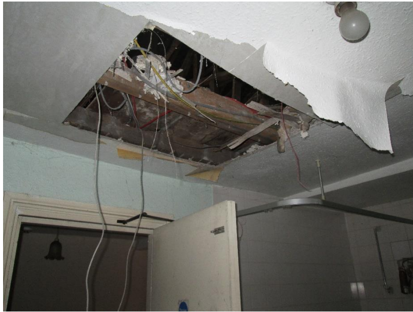
Photo 15 – Collapsed ceiling in bathroom
