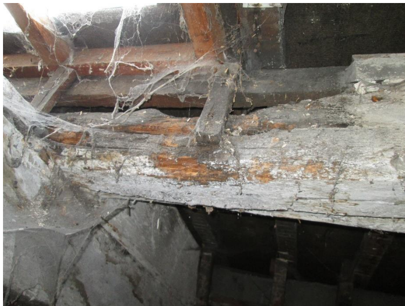
Photo 8 – Decay to timber purlin at skylight
