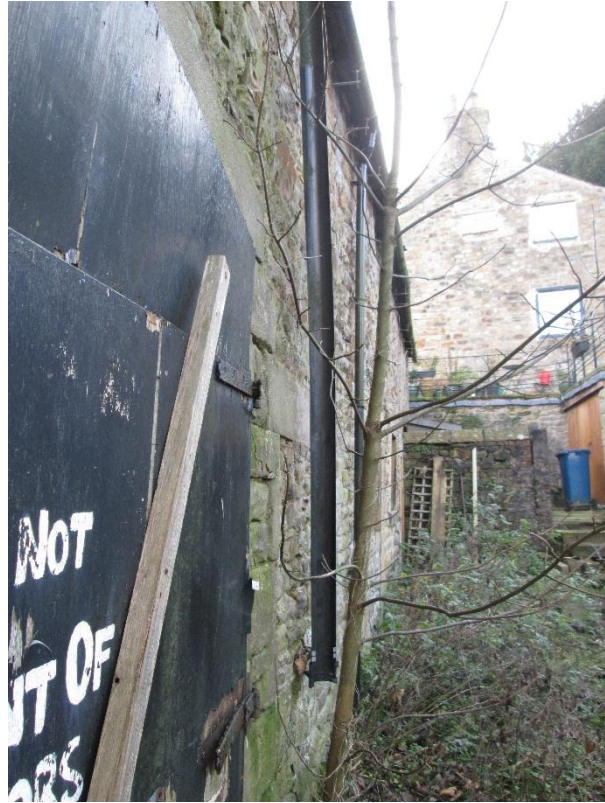
Photo 33 – Distorted rear wall
