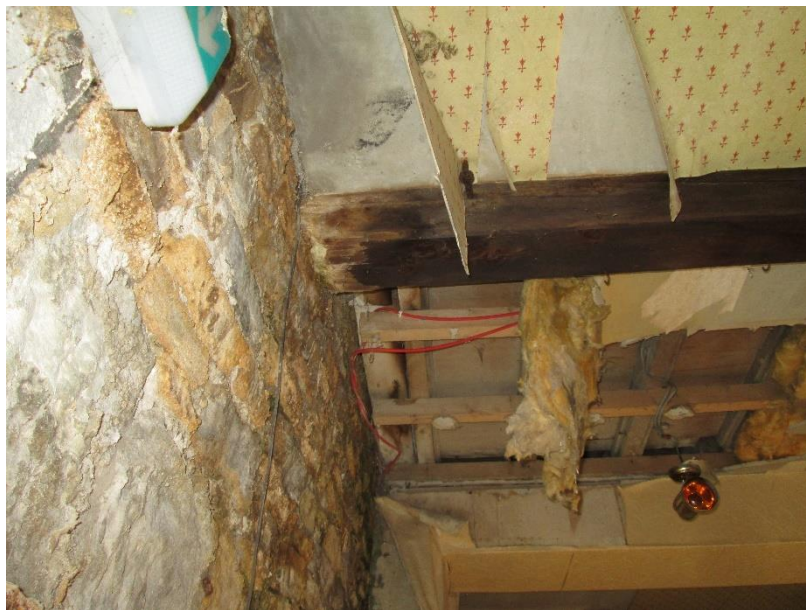
Photo 18 – Decayed timber and damp staining
