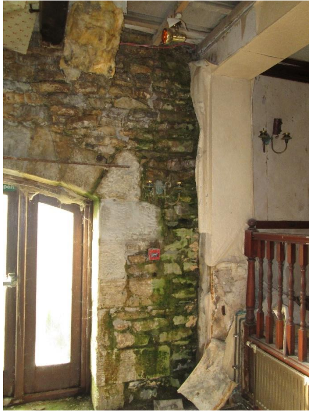
Photo 19 – Water ingress in front right-hand lounge
