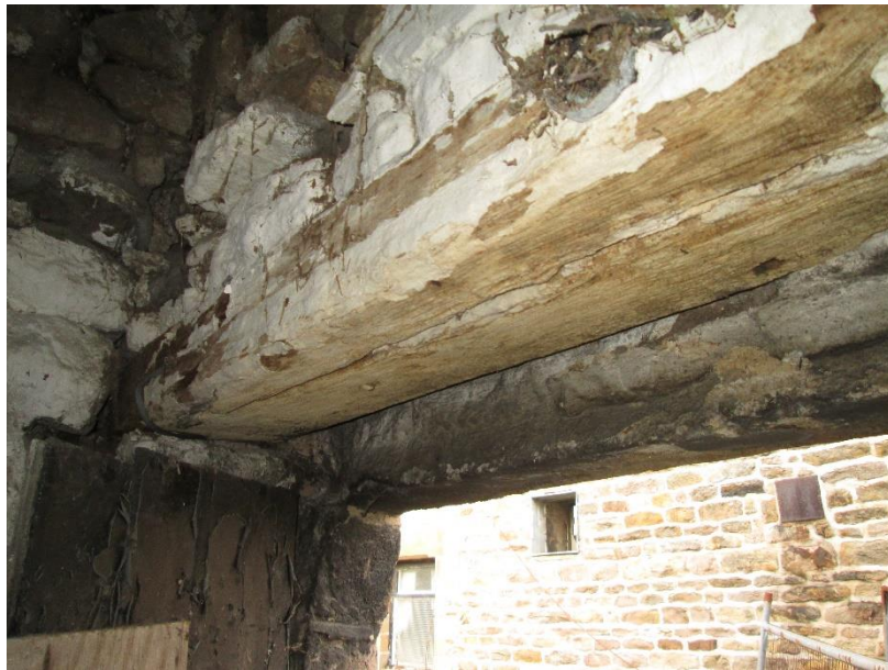
Photo 29 – Decayed timber lintels
