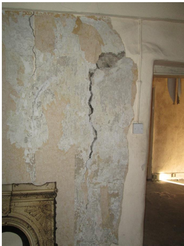
Photo 14 – Crack in wall of rear left-hand bedroom
