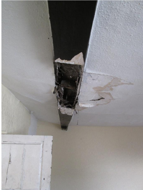
Photo 13 – Exposed truss tie beam showing signs of decay
