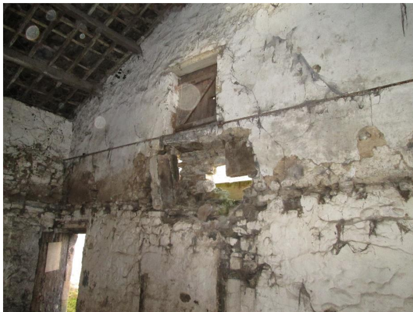
Photo 28 – Hole in right-hand gable wall
