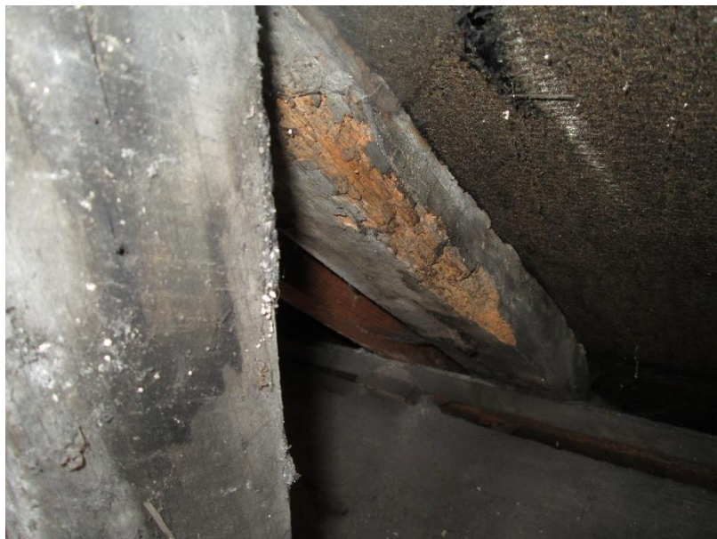
Photo 6 – Decay to original timber rafters
