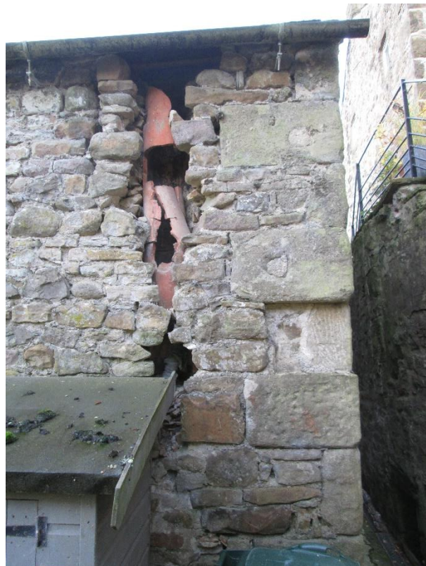
Photo 34 – Damaged stone and exposed flue
