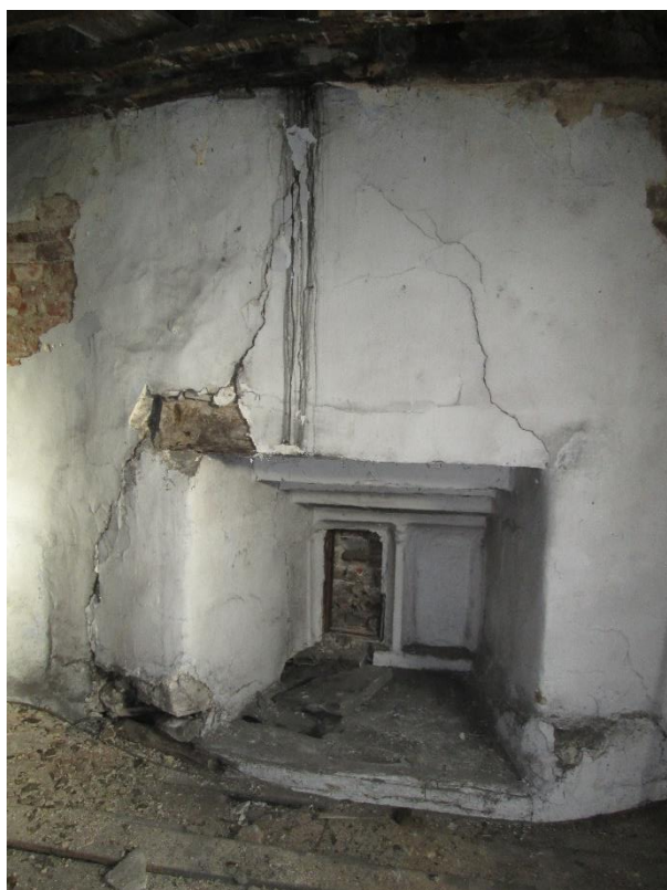
Photo 12 – Cracking to chimney breast
