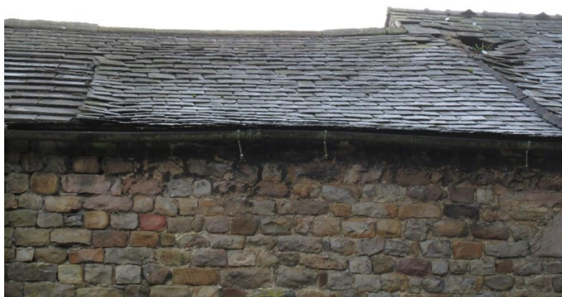
Photo 30 – Partially collapsed slates
