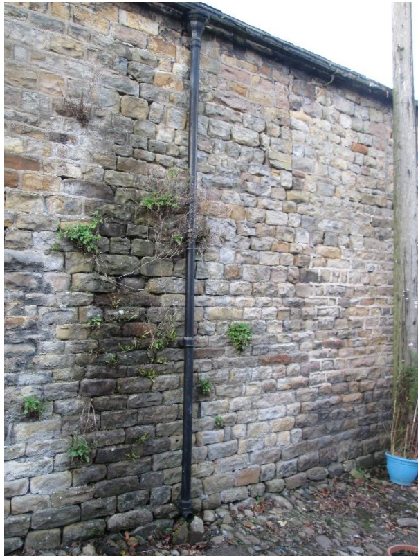
Photo 31 – Water staining and vegetation growth
