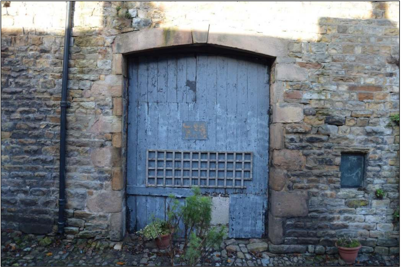
PL75: View of the former crat entry to the front south east elevation of the barn.
