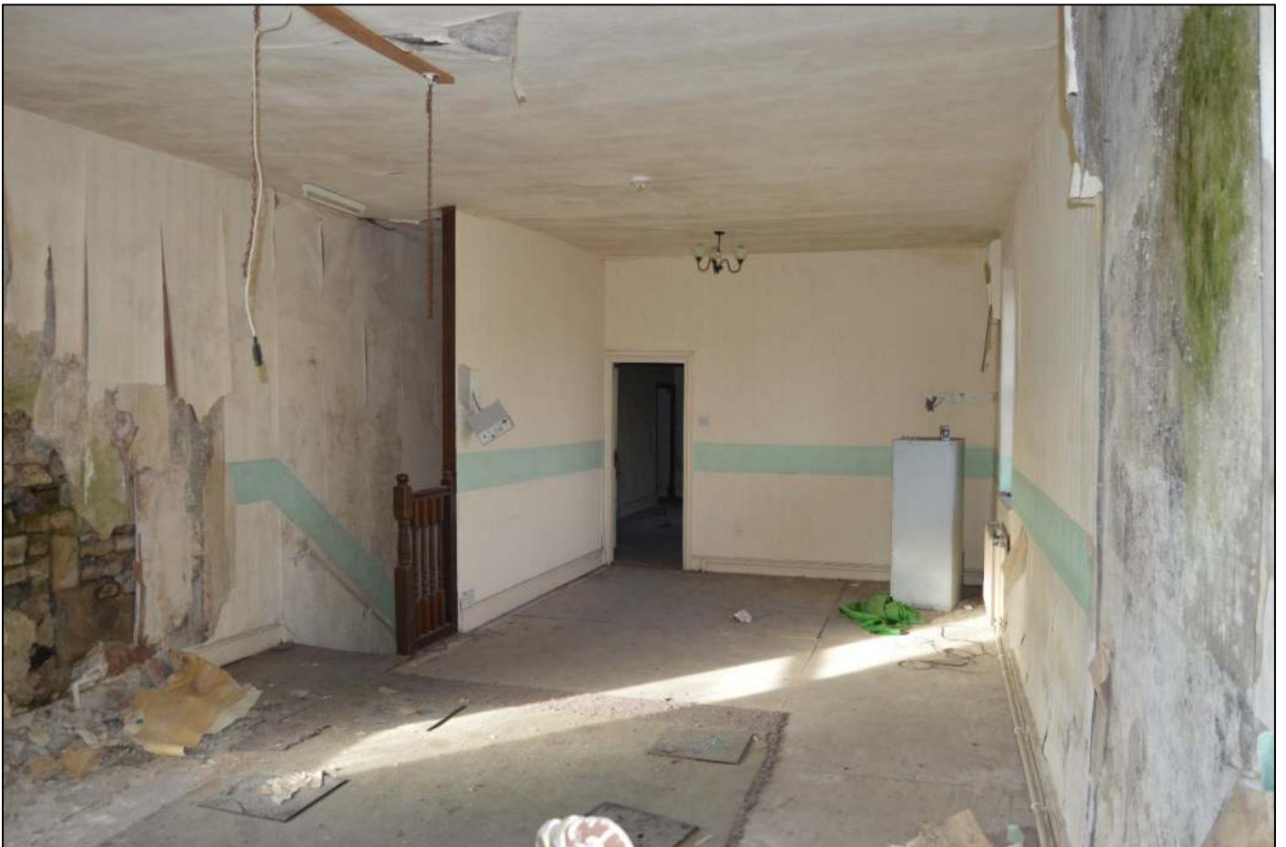
PL38: View north west within the front first floor unit of the coach house addition.
