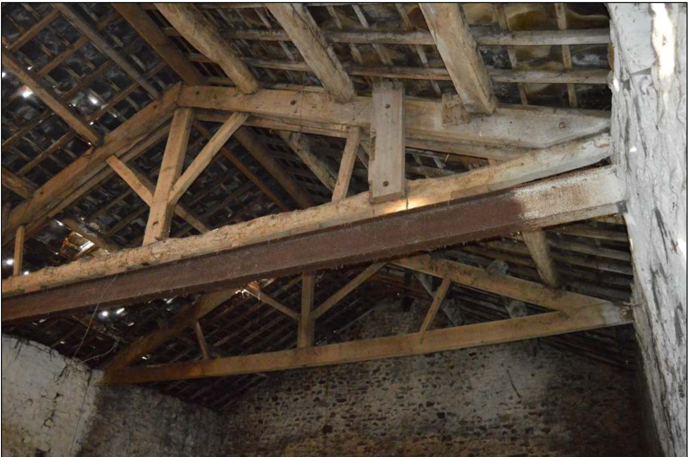
PL84: View of the 2no timber king post roof trusses to the south end of the barn.
