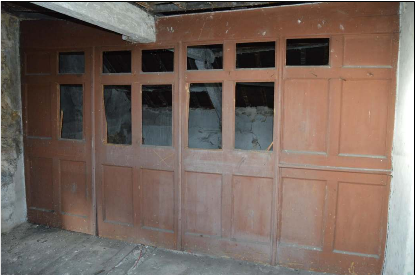
PL68: View of the timber partition within the south unit of the attic.
