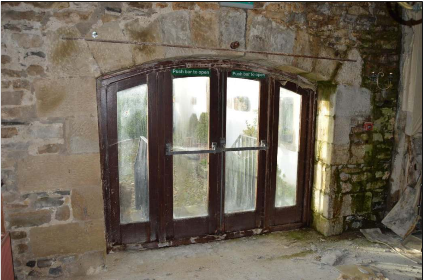
PL36: View of the former coach entry to the to the ground floor south east unit of the coach house addition.
