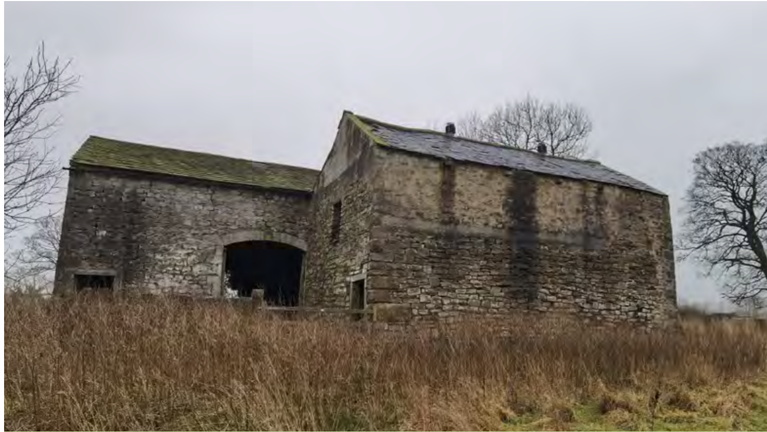
The existing ruined bothy house at the heart of Phase 6 has suffered considerable structural degradation
