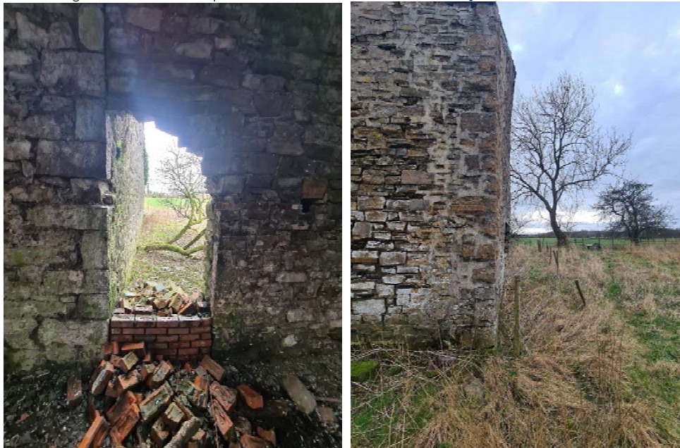
Image 8 showing collapse of previous masonry infill at the junction of the western and eastern sections. Image 9 side elevation shows the extent of distortion in the stone panel with it believed that the movement is largely recent because of poor remedial works and new roof.
