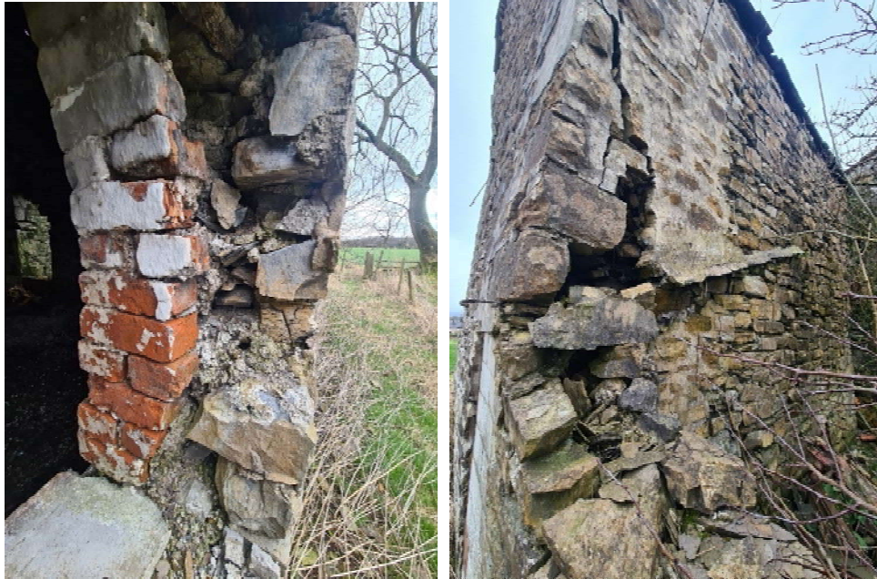
Image 6 showing circa 140mm bow of a remedial masonry support that highlights recent movement. Image 7 indicates a significant and severe separation of the wall at blockwork infill and junction of elevations.
