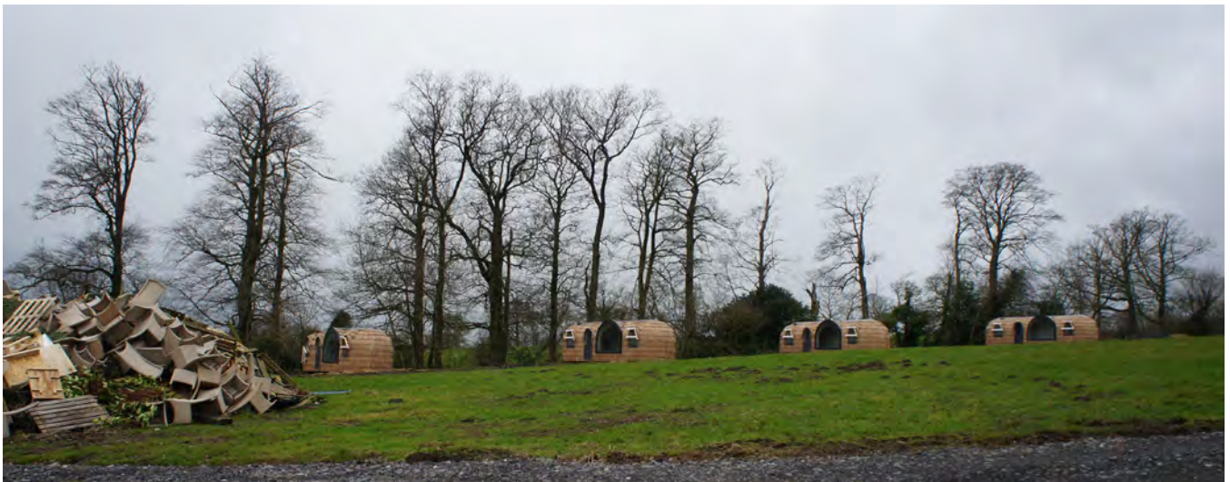
View from the centre of the development site looking west, showing the already installed eco-lodges
