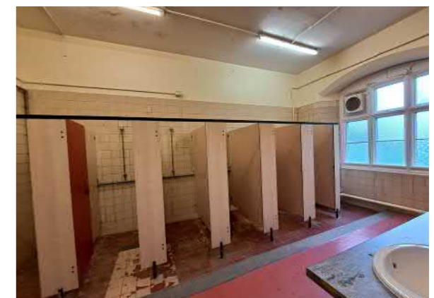
Existing shower/ changing space is detrimental to the historic fabric
