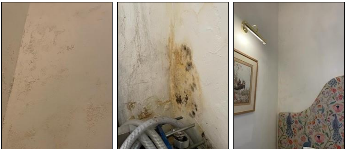
Fig. 1 illustrating internal damp issues.
