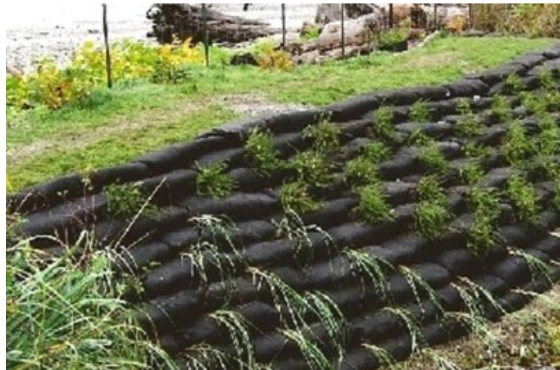
Type C - Green Wall formed with Sand Bags (prior to growth of green wall)
