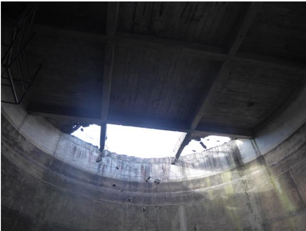
Photo 2: Water Tower missing roof
