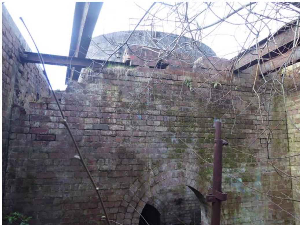
Photo 10: Valve House interior and Missing Roof
