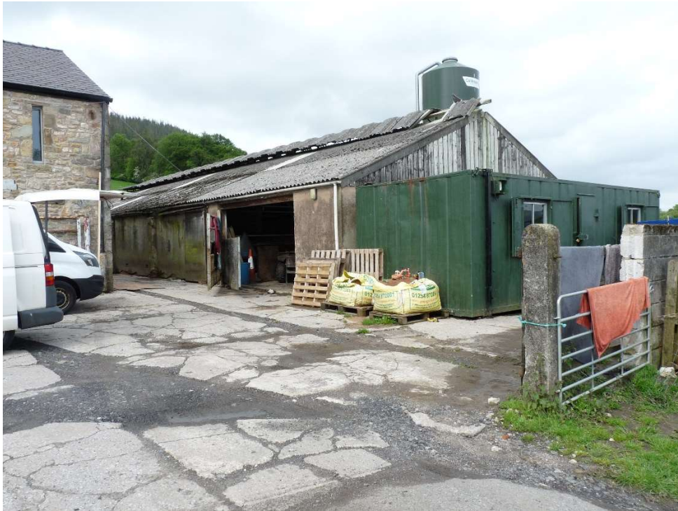
Entering site office and wall to be removed, note storm damage to roof
