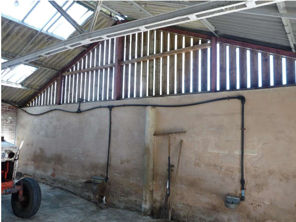
Internal wall finish machine storage not secure
