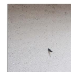
Photo 7: Single bat dropping on inside of east elevation wall.
