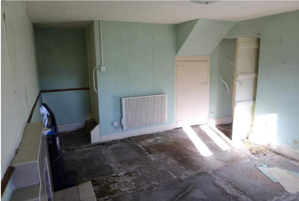
Plate 11: Living room facing towards the boxed-in staircase , facing north-east towards the property
