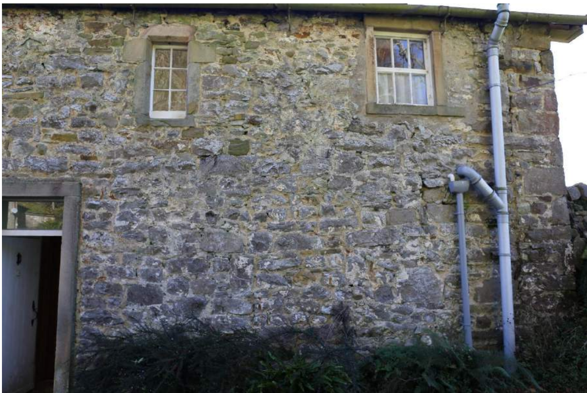
Plate 22: Re-used mullion window to front elevation, note also wide sill to right indicating re-modelling of window. Note also possible blocked doorway in centre of frame defined by two vertical joints.
