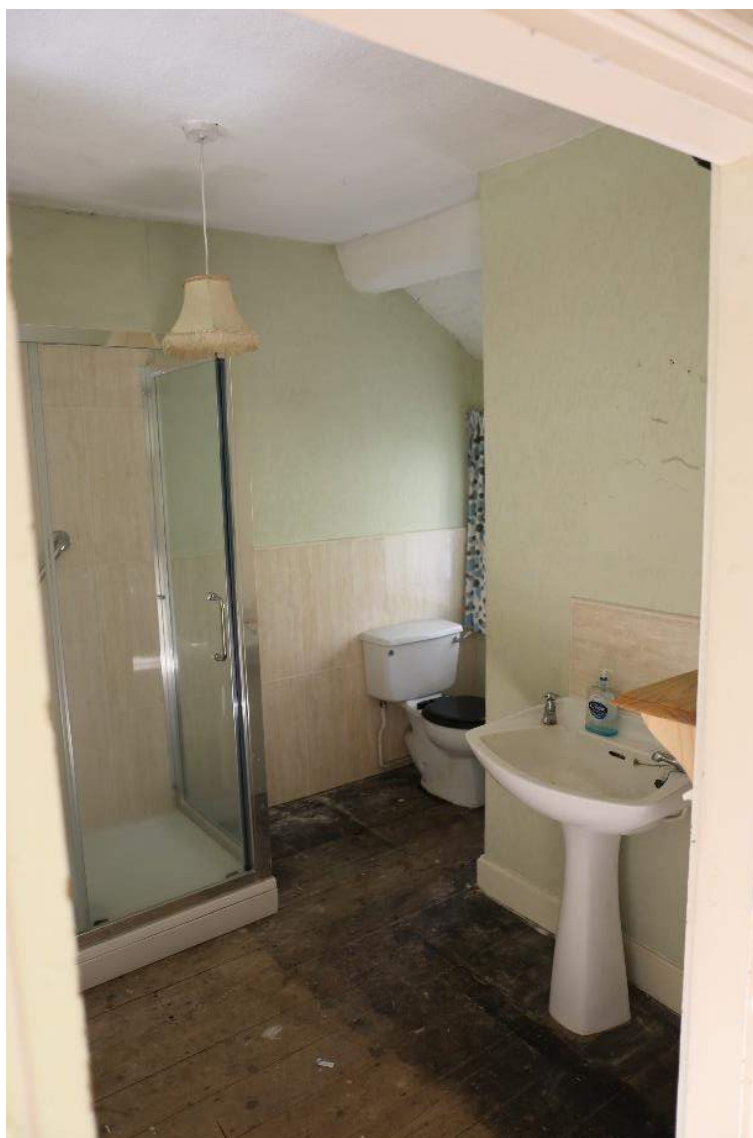
Plate 14: Shower room on first floor and discoloured flooring, facing west
