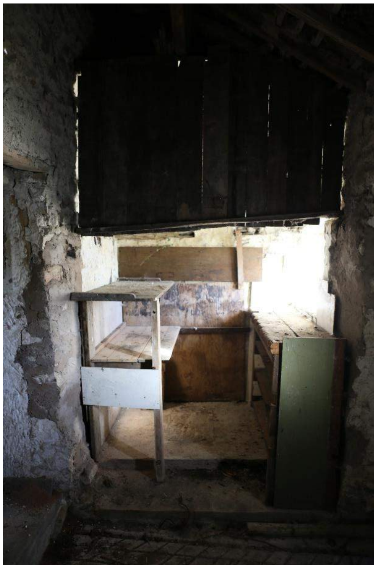
Plate 29: Residual timber hayloft structure over workbench, note grooves in dung channel to front of frame
