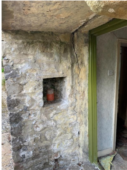
Minor Cracking between stairs and rear wall
