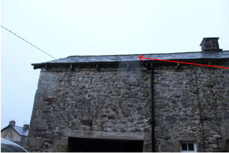
Slipped slates on the roof
