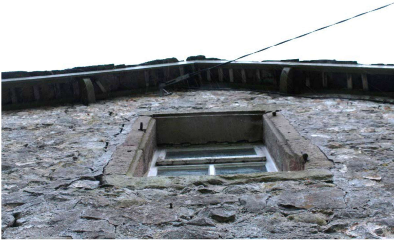
Gaps along the roof verges
