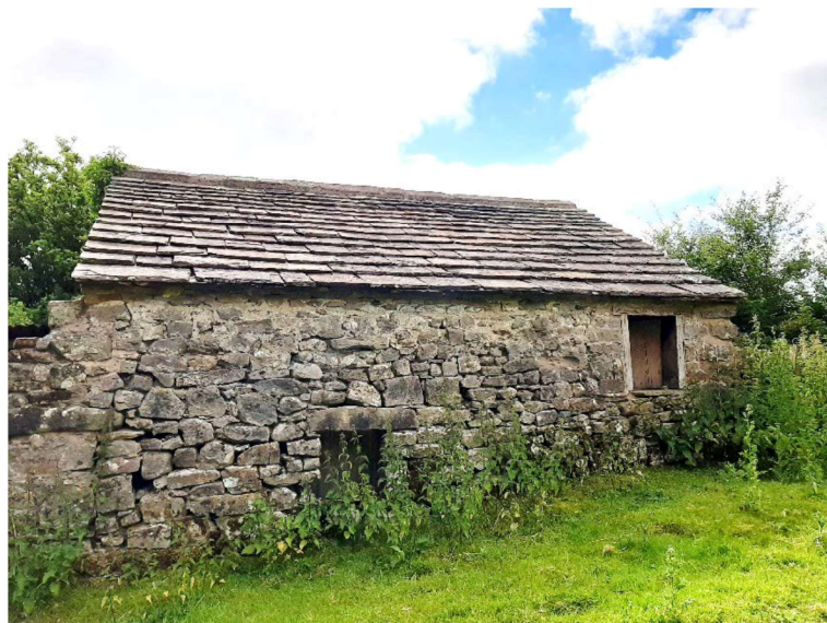
The store has well sealed walls and a stone slate roof. It is a small building which could be fully inspected during the daytime surveys
