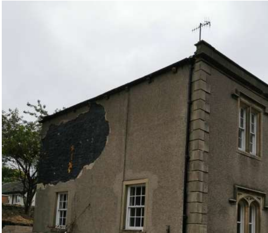
FIGURE 5: IMAGE OF THE SIDE ELEVATION WITH MISSING/DAMAGED RENDER
