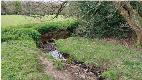
Photograph 7: Vertical cut banks along the stream. No evidence of burrowing from either kingfisher or water vole.
