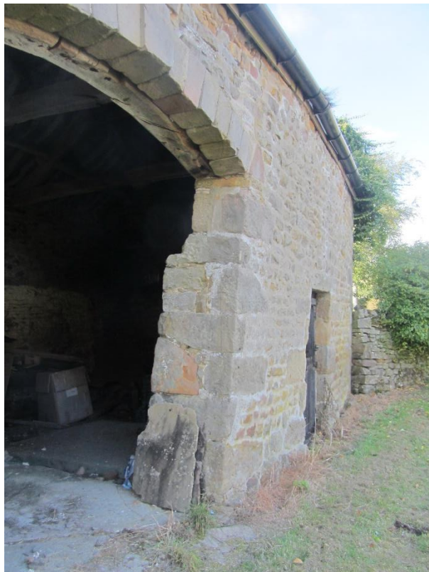
Photo 10 – Extreme lean of eastern wall to northern space
