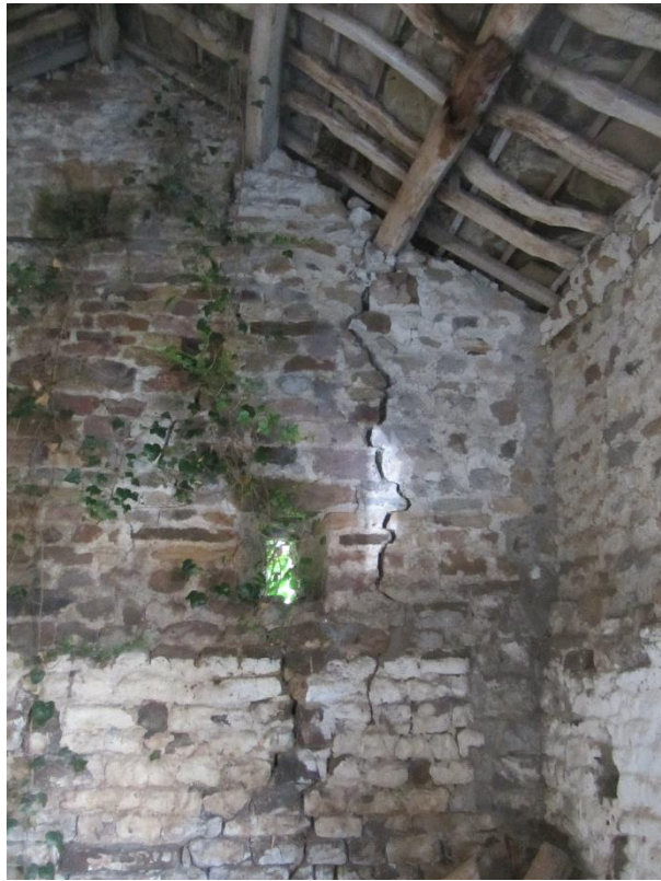
Photo 5 –Vertical crack on north gable wall
