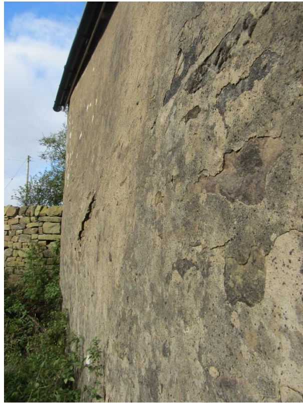
Photo 11 – Significant bulging of western wall to northern space
