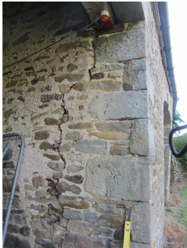
Photo 8 – Vertical crack in wall between northern and southern spaces
