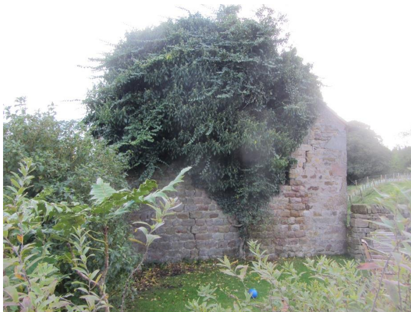
Photo 12 – Vertical crack in northern gable wall
