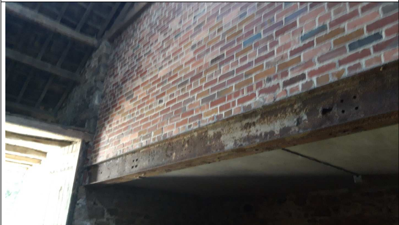
Corroding Beam Supporting 1 st Floor and Wall in North West Barn
