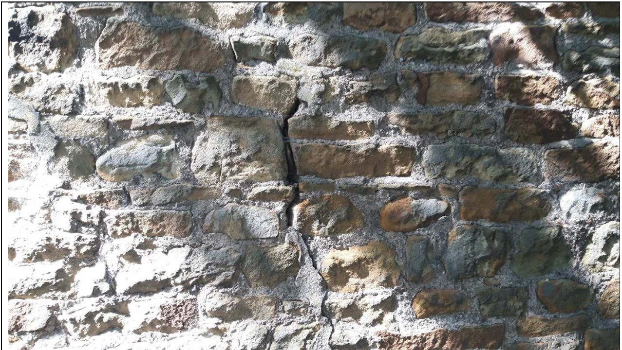
Crack to Mid-Point of South Wall to South East Barn
