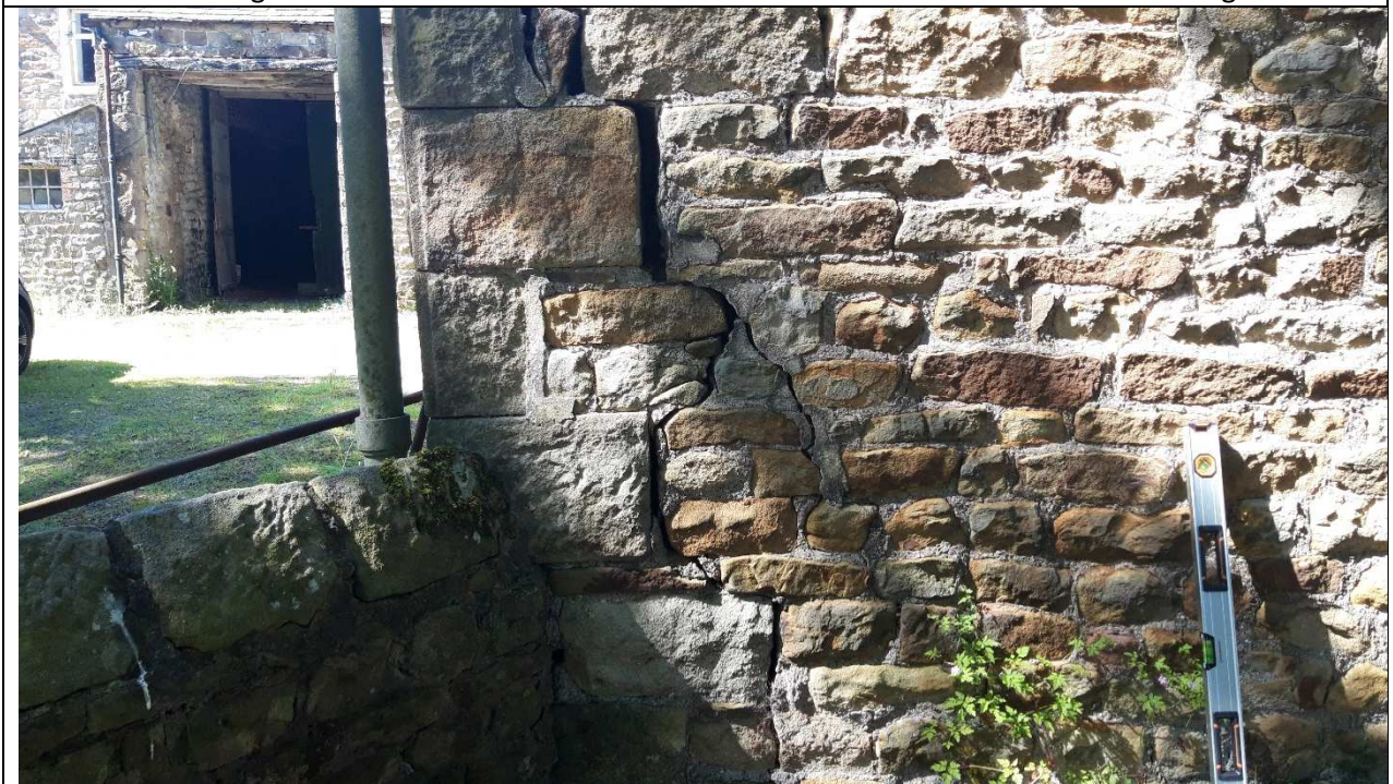
Cracking to Left End of South Elevation Wall of South East Barn at Base of Wall
