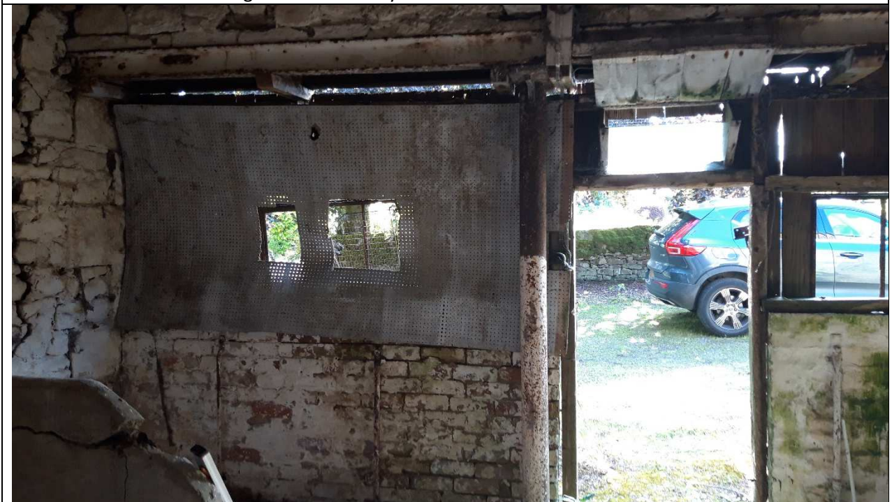
Corroding Frame to South East Barn
