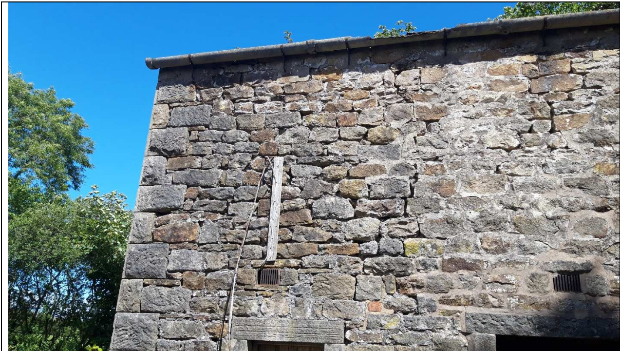
Cracking to Front Wall of South East Barn
