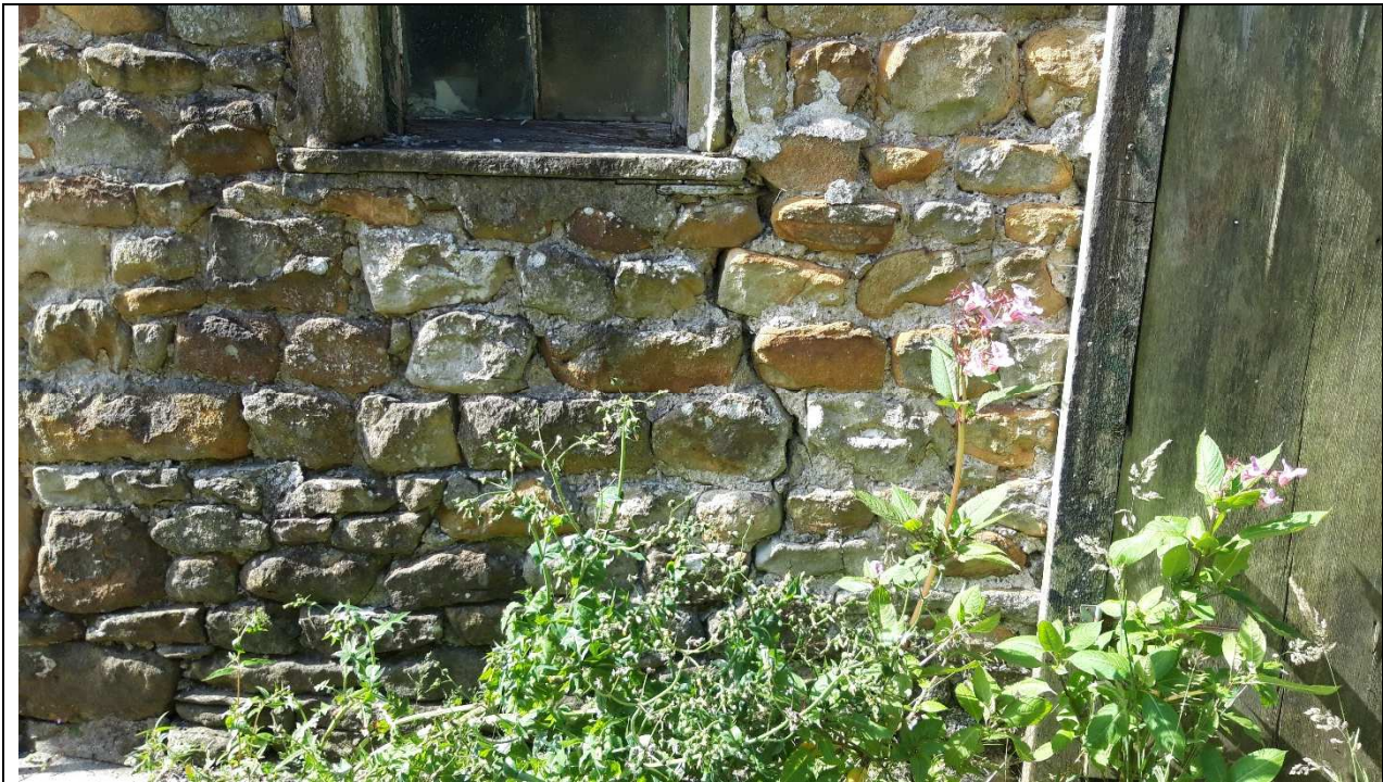
Crack Below Front Wall (South) to North West Barn
