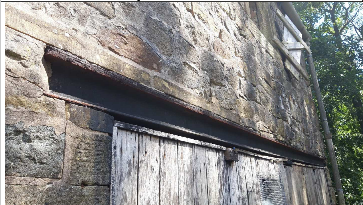
Corroding Beam Over Opening to Front Wall of South East Barn
