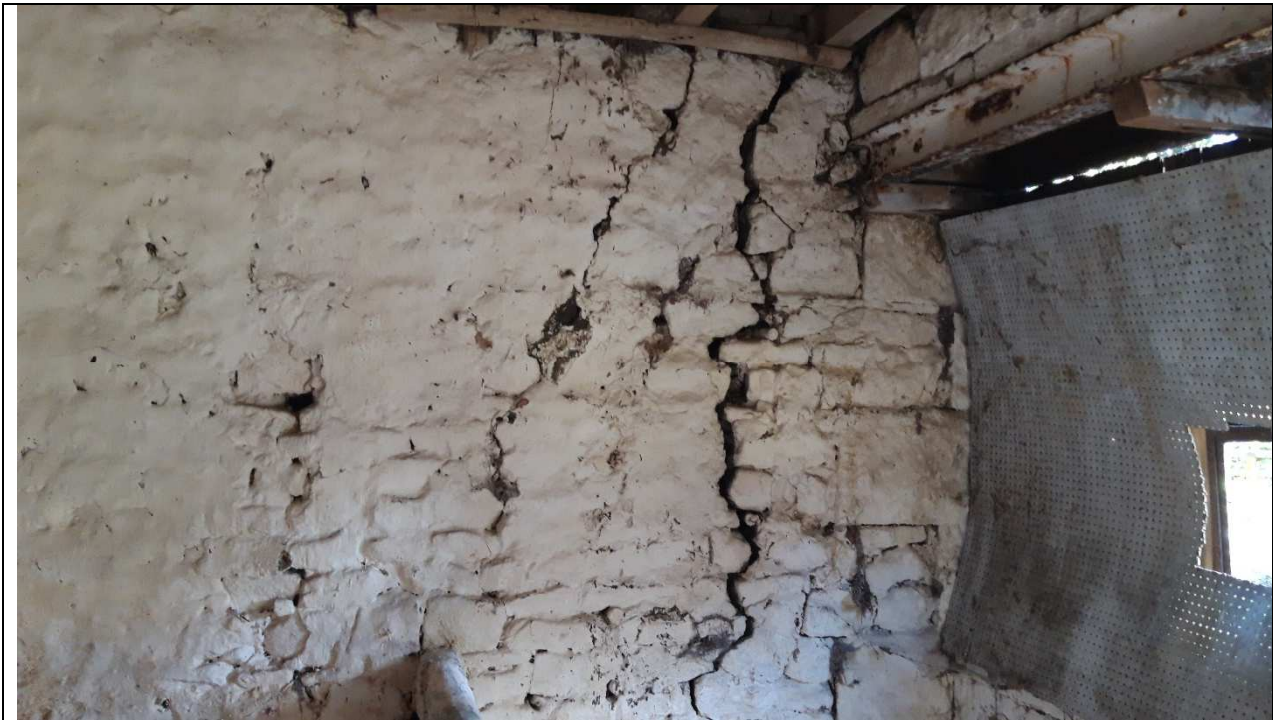
Large Crack Internally to South Wall of South East Barn
