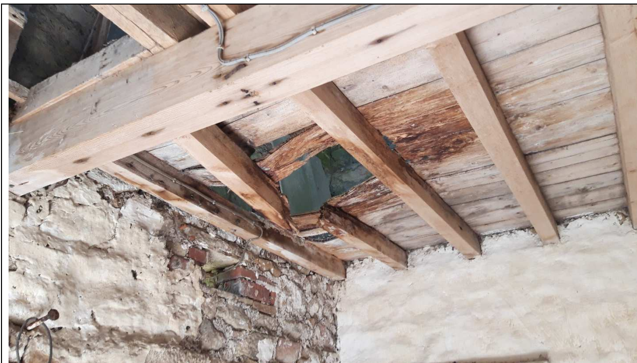
Damaged 1 st Floor to South East Barn
