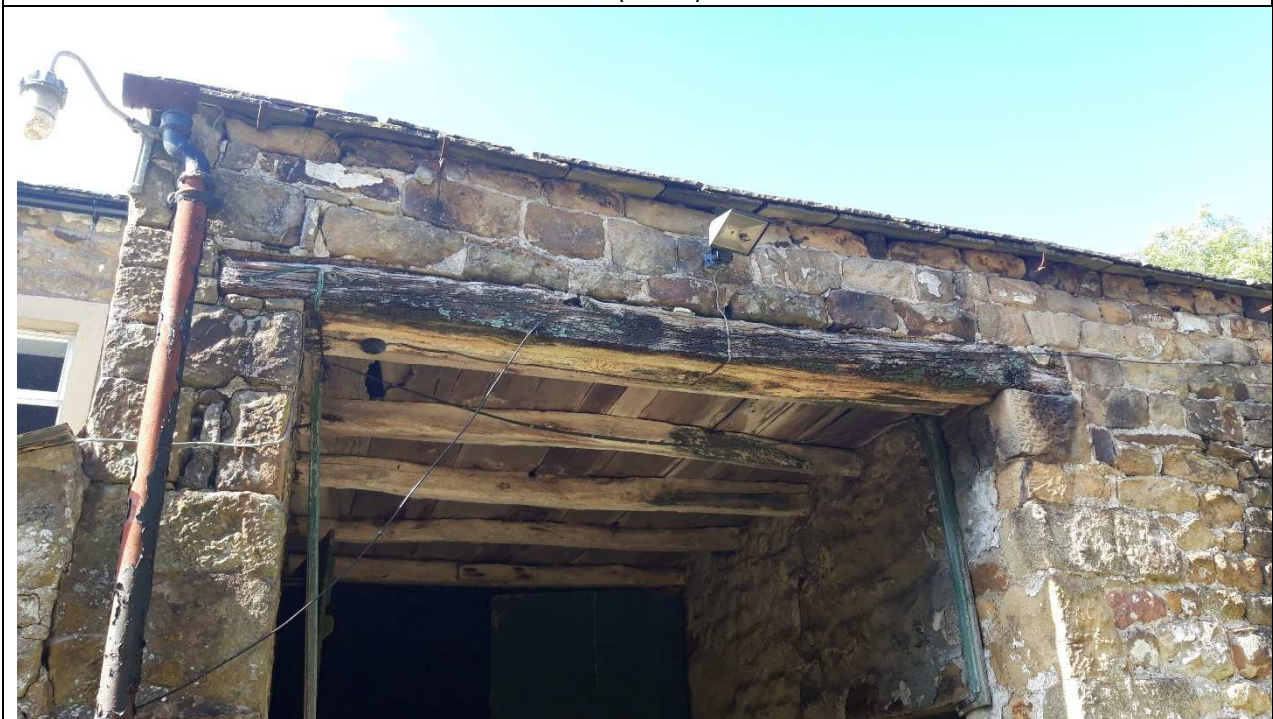
Lintel in Poor Condition to Main Door Over North West Barn Opening
