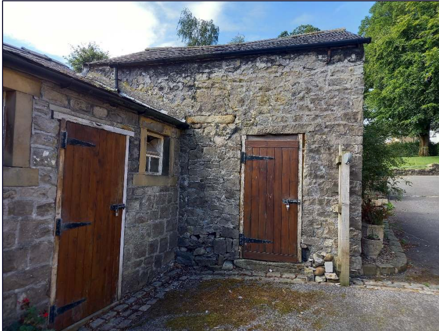
Plate 19: North-east elevation of Building B, with Building A to left of photograph
