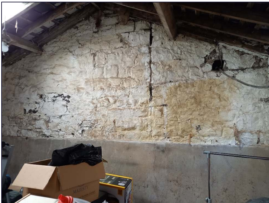
Plate 18: South-west internal wall of Building A showing the vertical construction break where Building A has been constructed against part of Building B
