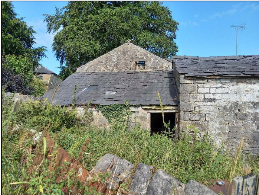
Plate 25: South-east gable of Building B largely obscured by the roof of Building C
