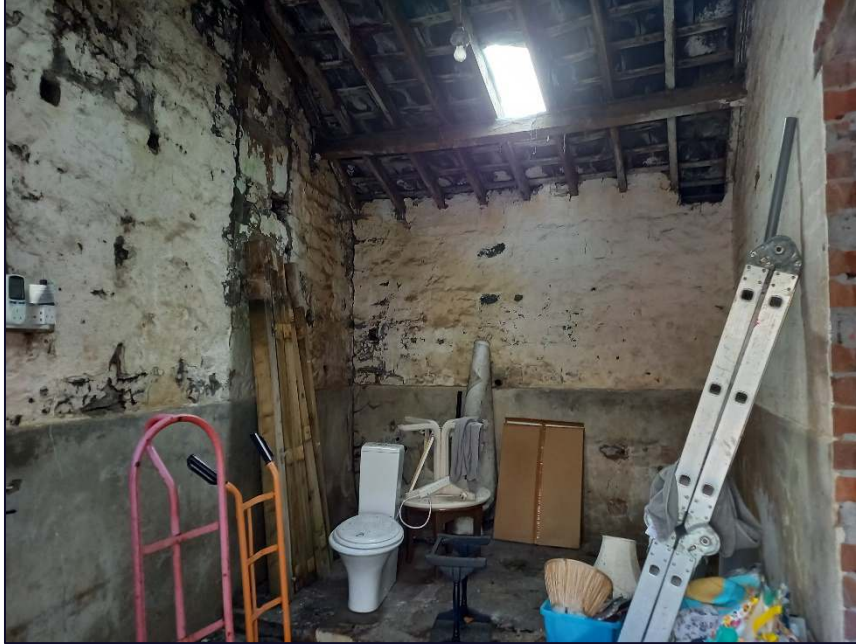
Plate 13: Interior of Building A showing plastered and white-washed walls and concrete floor
