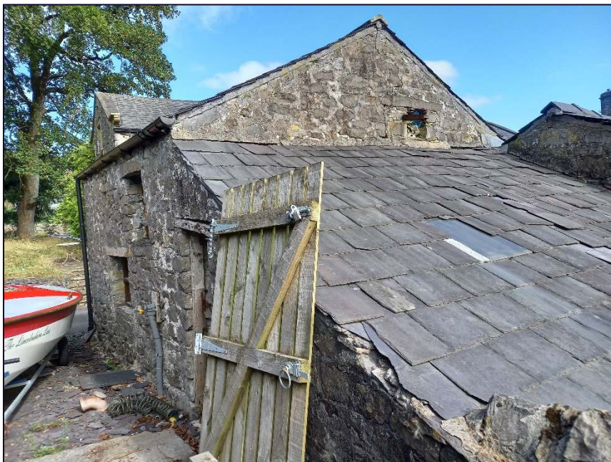
Plate 28: View looking north showing Building B with the roof of Building C to right of photograph
