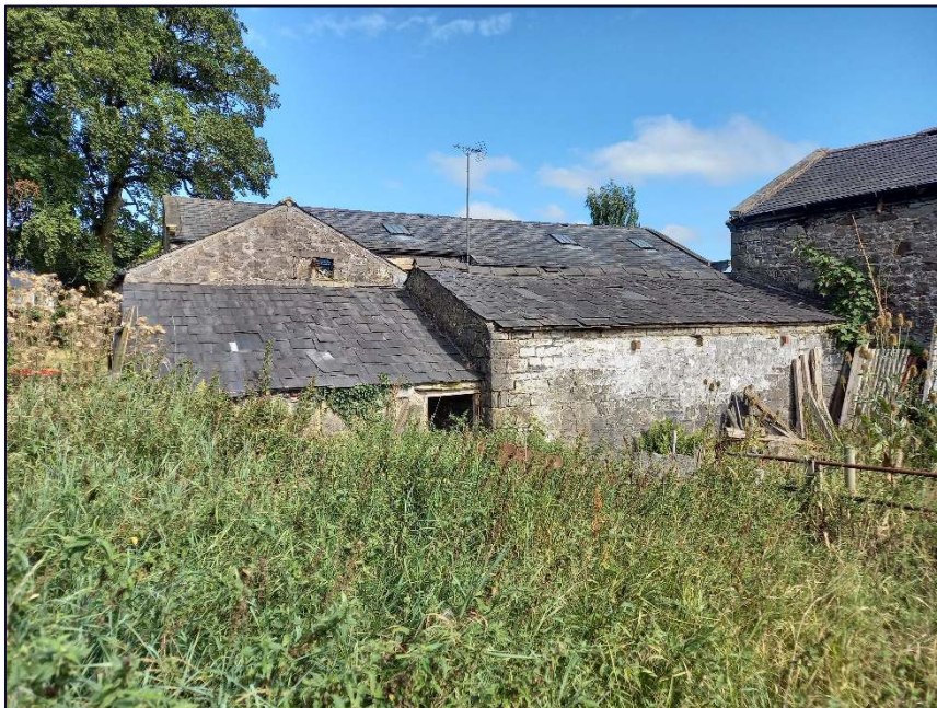
Plate 12: View looking north showing the south-east (rear) elevations of the buildings proposed for conversion
