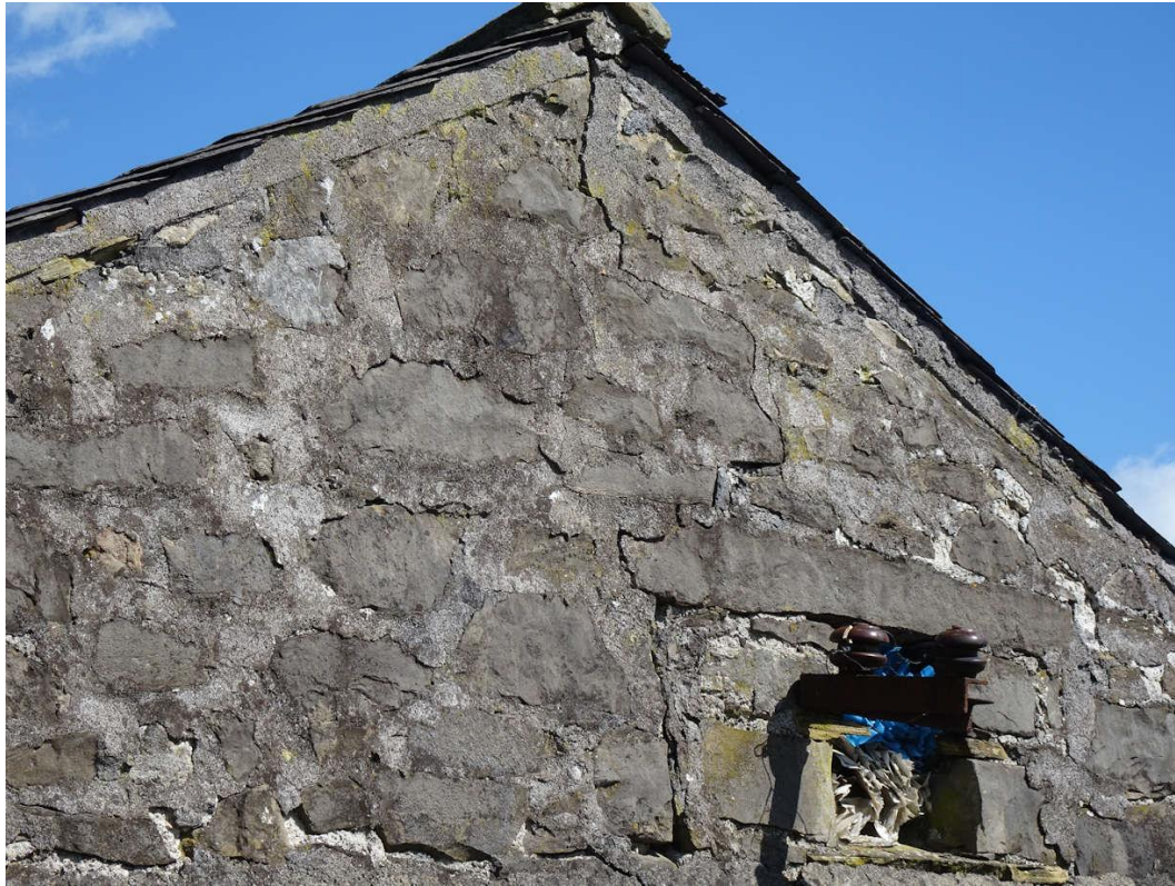
Photograph 7: Cracking In Bedroom Rear Elevation
