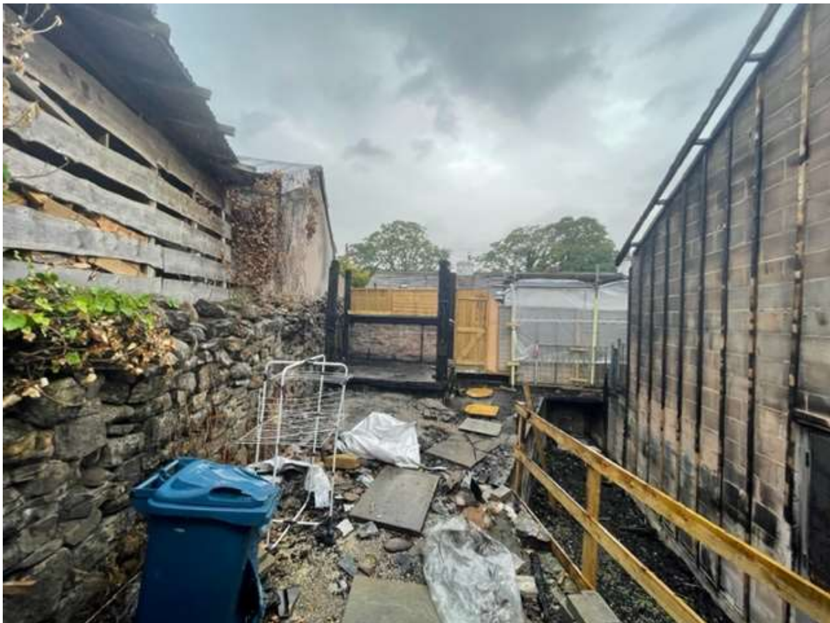
View of the application site from the south (fire damage evident)
