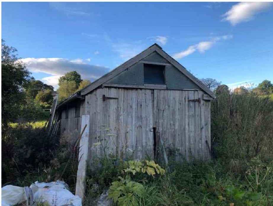
Existing dilapidated timber building in need of repair
