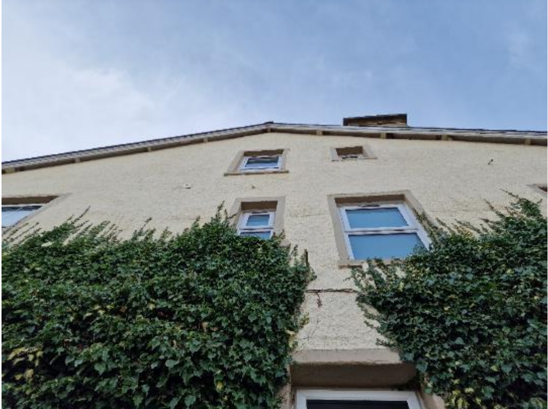
Plate 6 – General character of the northern gable; note the ivy which was used by house sparrow
