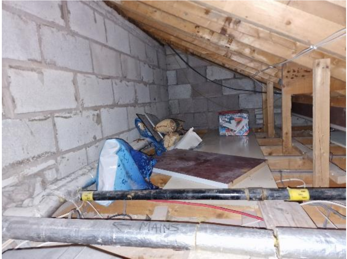
Plate 10 – Additional image showing the internal character of the void in Section 2.
