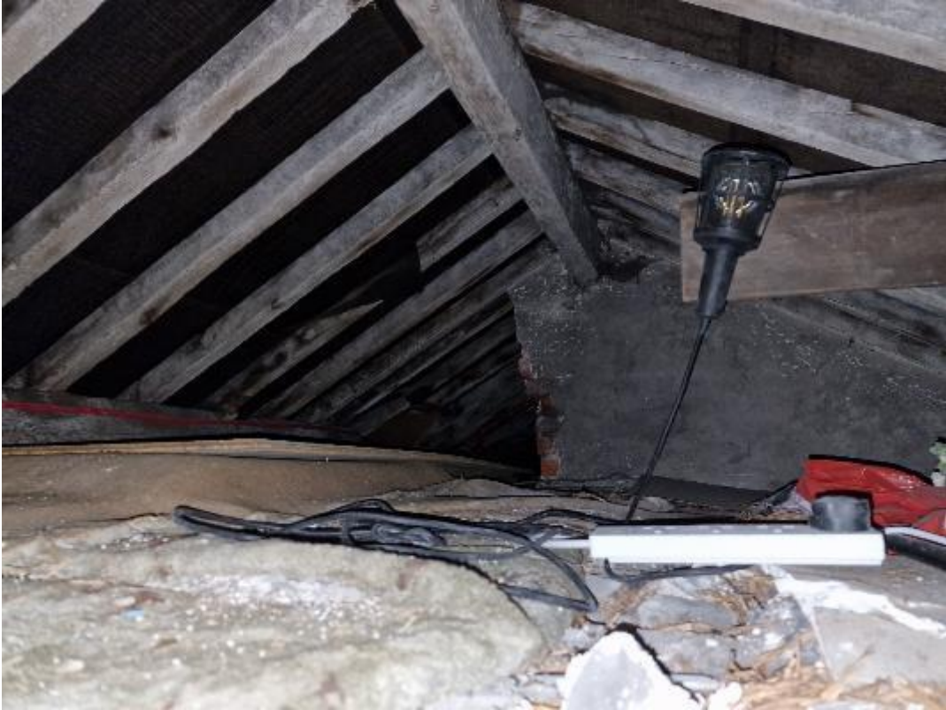
Plate 7 – General character of the internal void within Section 1
