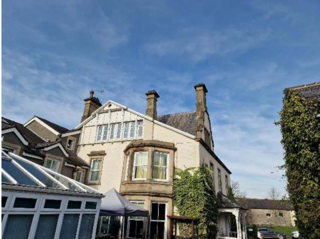
Plate 3 – General character of Section 3; see hang tiles are present and ivy growth
