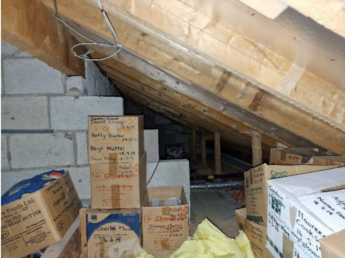
Plate 9 – The general character of the second void, used for storage, within Section 2.
