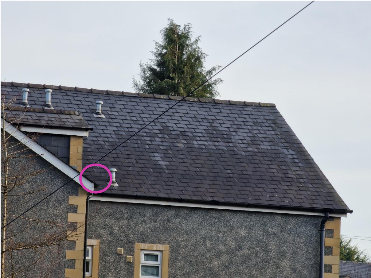
Figure 5.4 – Emergence Point 1 identified on the southwest elevation of the Manor Care Home
