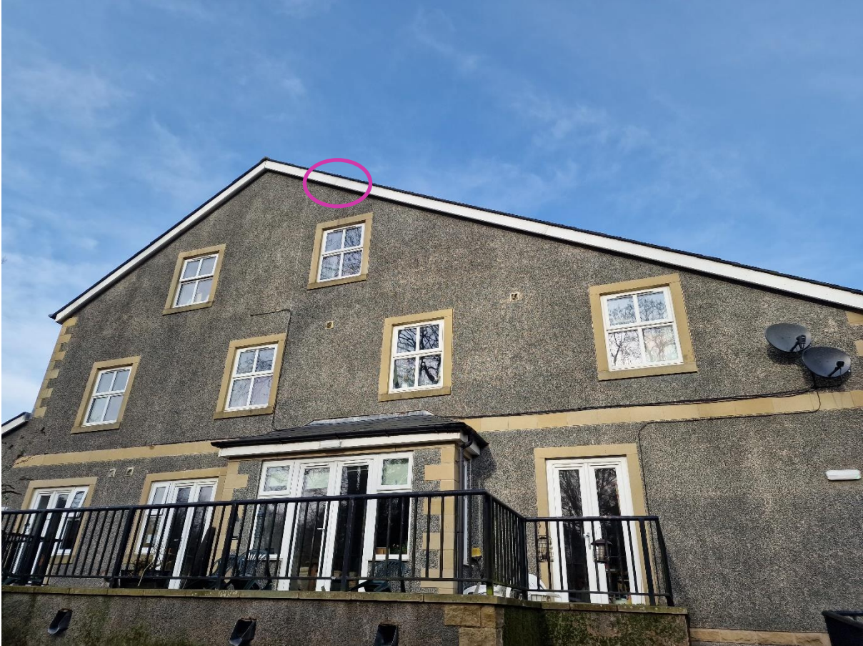
Figure 5.5 – Emergence Point 2 identified on the southern elevation of the Manor Care Home
