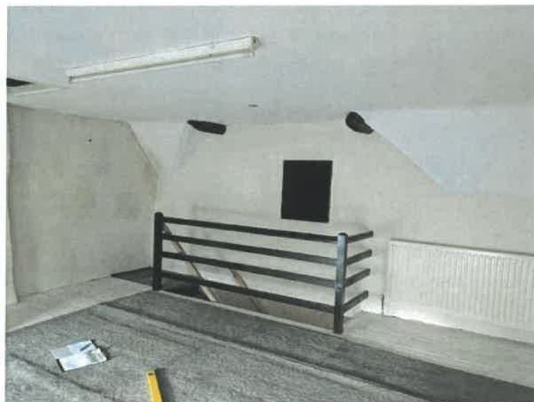
Figure 7.8.1: Western room ceilings and staining at valley connection
