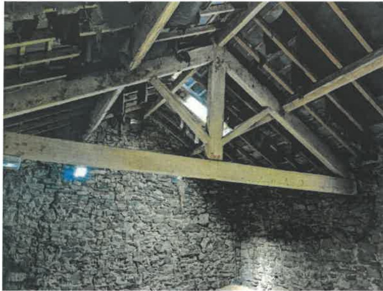
Figure 10.2.3: Northern gable with cracking to the side of the inwards bow
