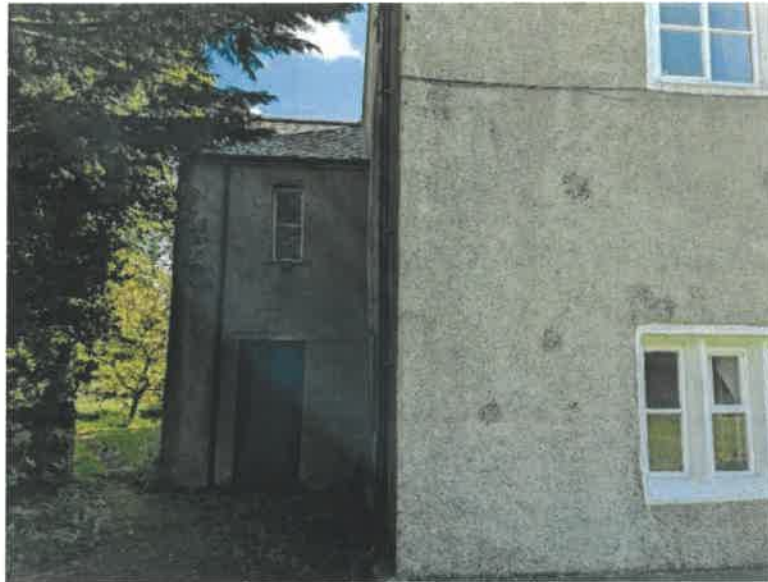
Figure 7.4.1: Bulge to the east wing wall
