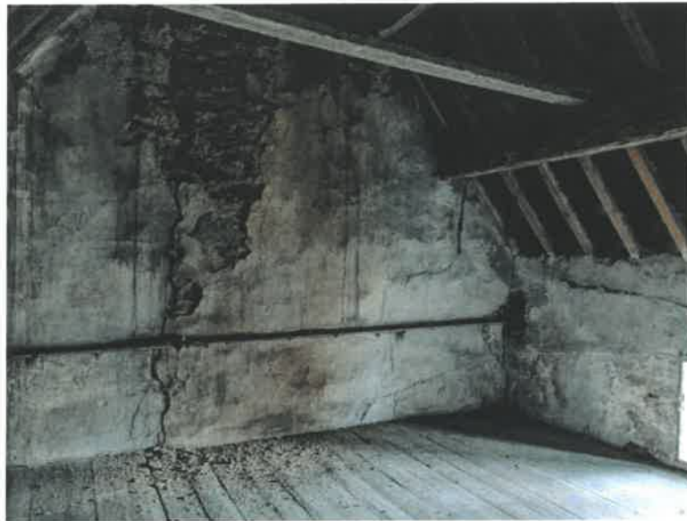
Figure 7.8.4: Eastern room water ingress below chimney and wall cracking
