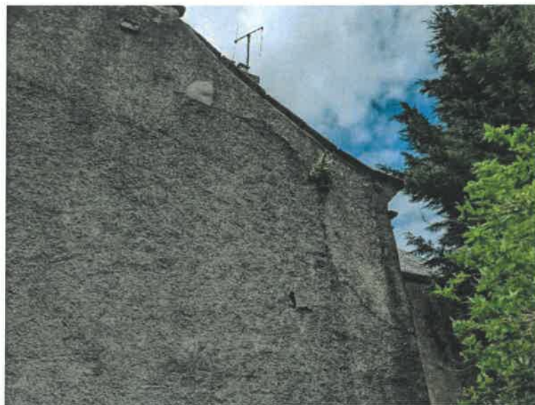
Figure 7.4.2: Cracked and spalled render to the cheese press gable
