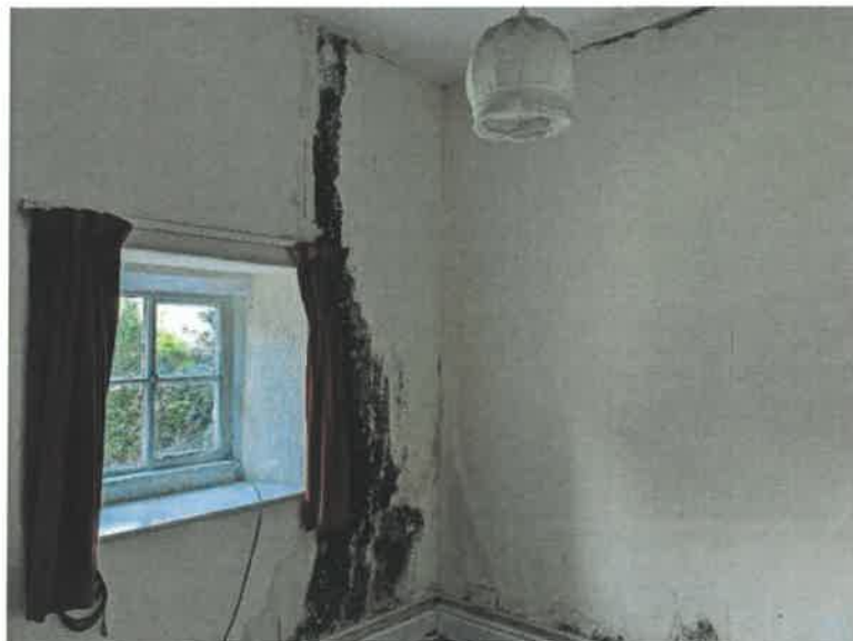
Figure 7.7.1: North east wing, first floor water ingress
