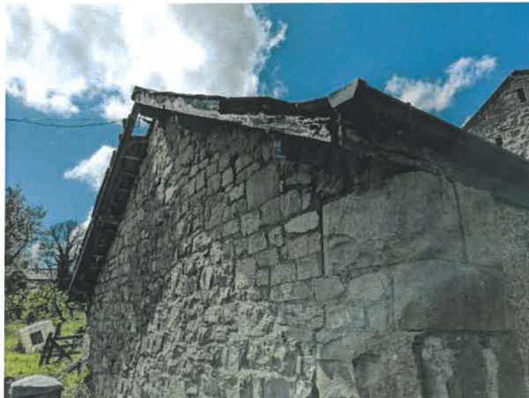
Figure 11.1.2: Deteriorated timber sections
