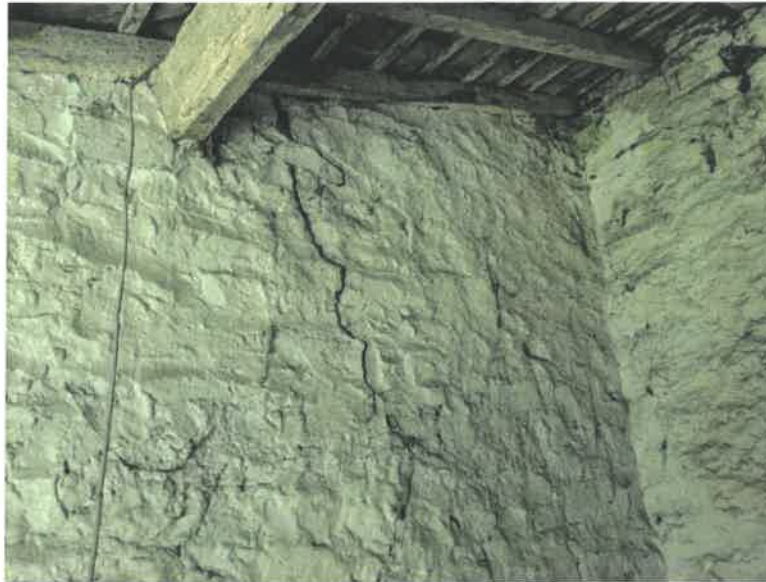
Figure 8.1.2: Cracking at purlin bearings
