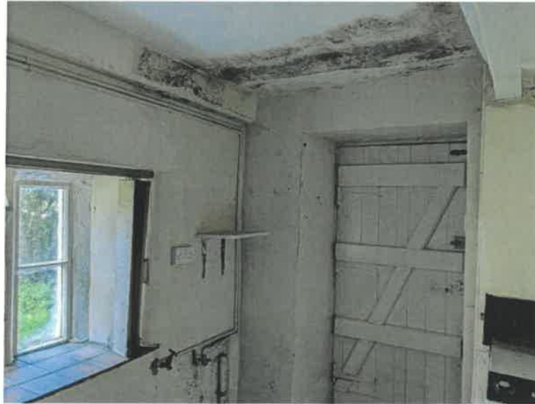
Figure 7.6.1: North east wing, ground floor bathroom water ingress
