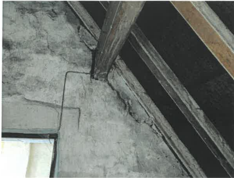
Figure 7.8.2: Eastern room cracking at purlin bearing
