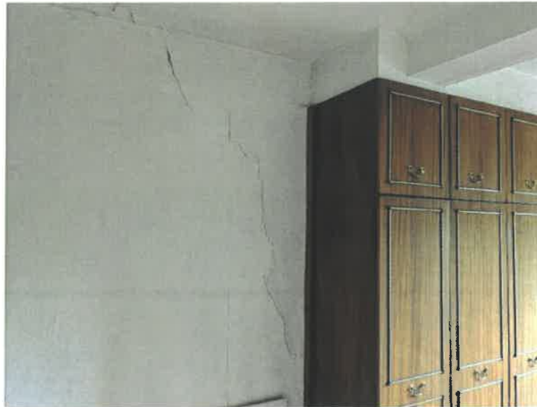
Figure 7.7.3: East gable wall cracking
