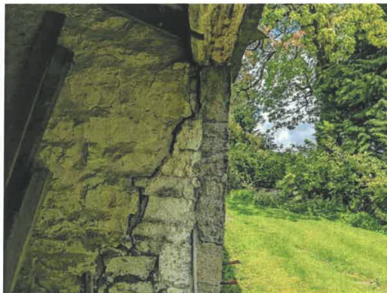
Figure 8.1.3: Wall settlement / cracking to front side
