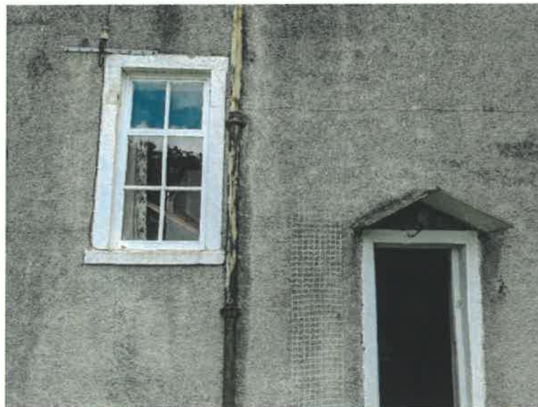
Figure 7.3.3: Render cracking between door and window
