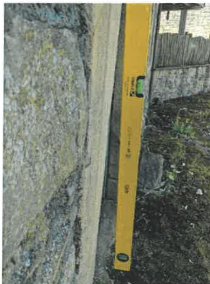
Figure 10.1.2: Severe lean to the centre of the front elevation walls
