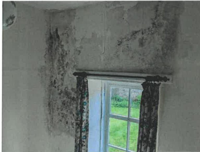
Figure 7.6.3: North east wing, water ingress at half landing level
