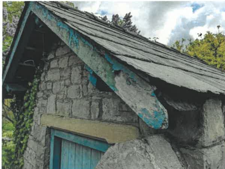
Figure 9.1.2: Deteriorated timber sections
