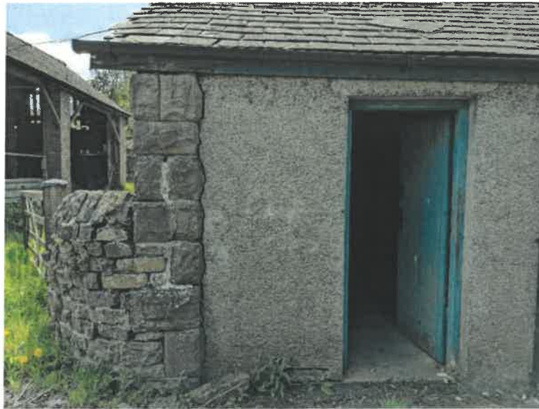
Figure 11.1.3: Wall / render cracking to corner quoin stones
