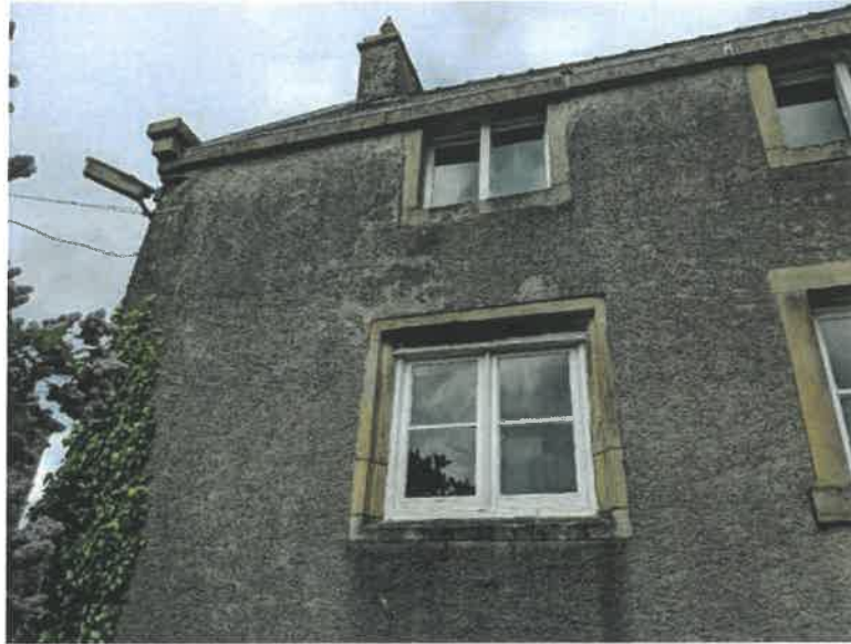
Figure 7.1.2: Render cracking between windows
