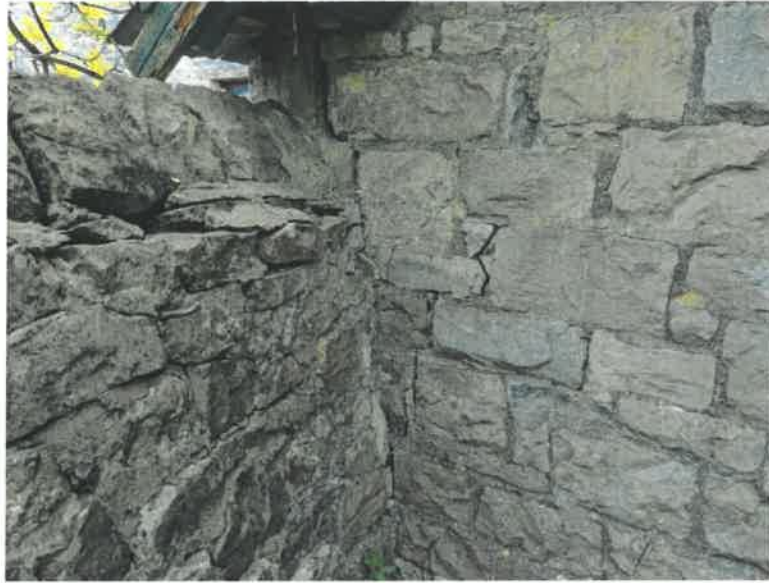
Figure 9.1.1: Coal store rear wall cracking
