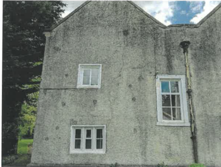
Figure 7.3.4: Large vertical crack to the eastern wing
