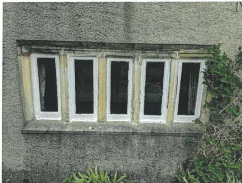
Figure 7.1.3: 5-panel window with heavily weathered stone surrounds
