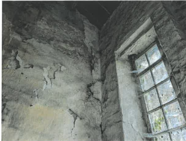
Figure 7.5.2: Cheese press south east wall corner with lack of tie in
