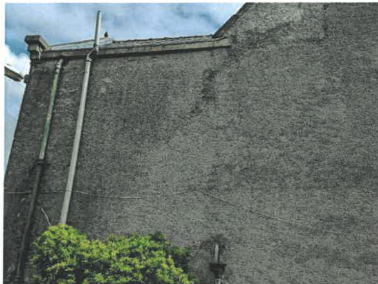
Figure 7.2.2: Vertical cracking in the render at wall / roof junctions
