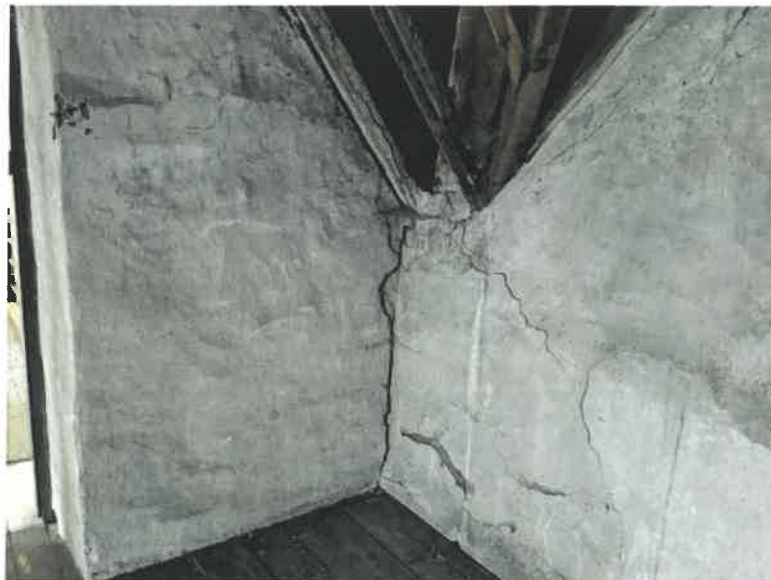
Figure 7.8.3: Eastern room wall corner separation
