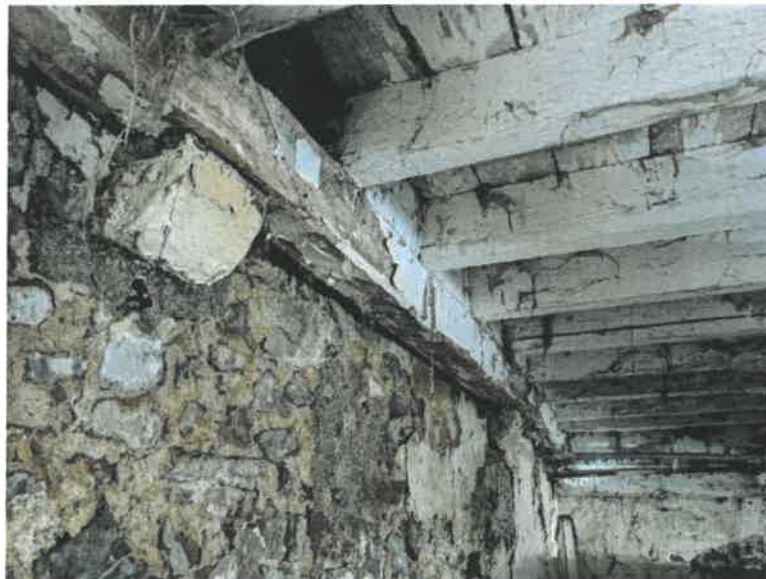
Figure 10.2.2: Front elevation wall corbel stones separated from the floor structure
