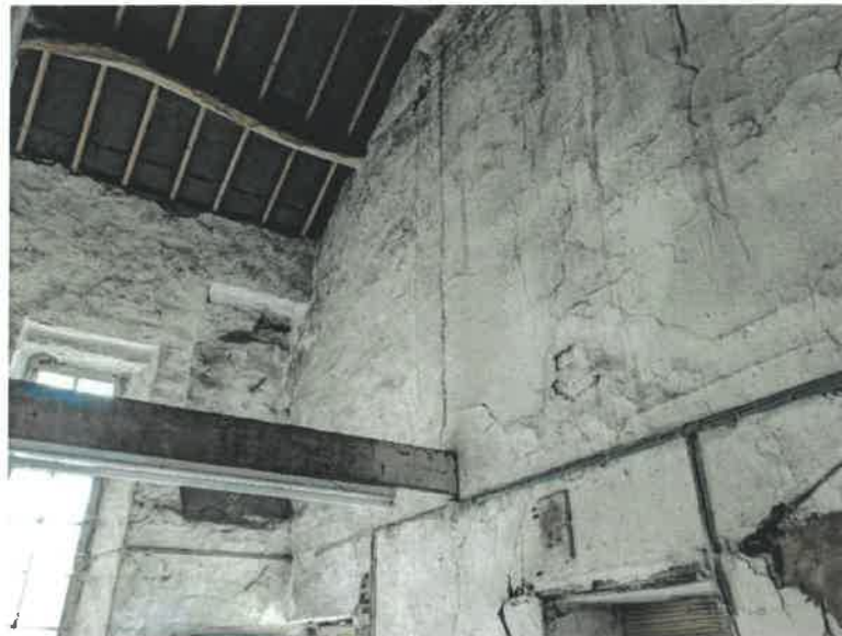
Figure 7.5.3: Cheese press to farmhouse wall vertical cracking
