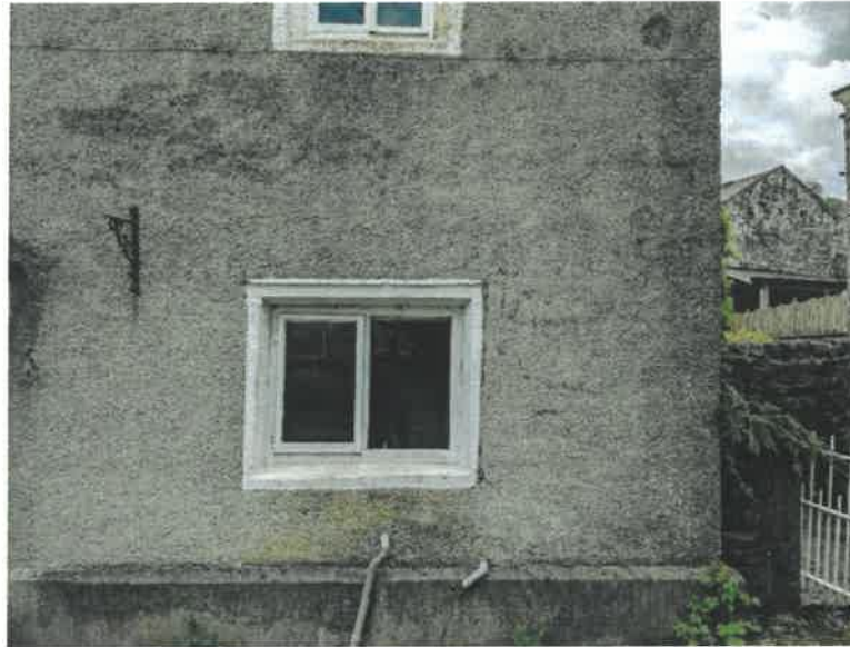
Figure 7.3.2: Render cracking between windows
