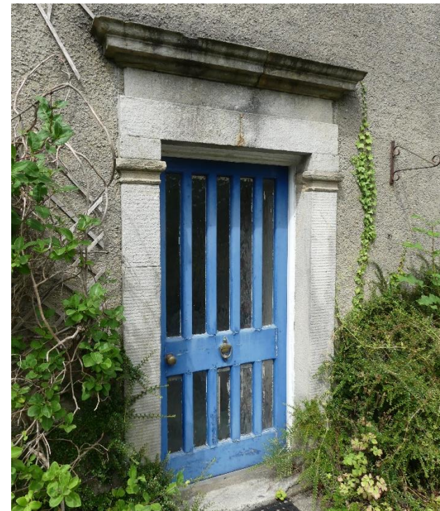
Figure 3.2: The principal door is framed with simple, chisel marked pilasters, a modest capital detail and entablature
