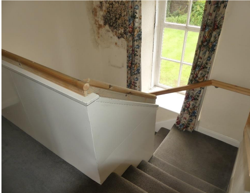
Figure 3.12: The staircase remains in situ, although the balusters have been boxed-in, and a new handrail installed
