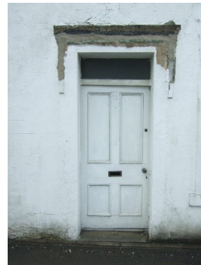
Picture 7 - Original front door with hood missing
