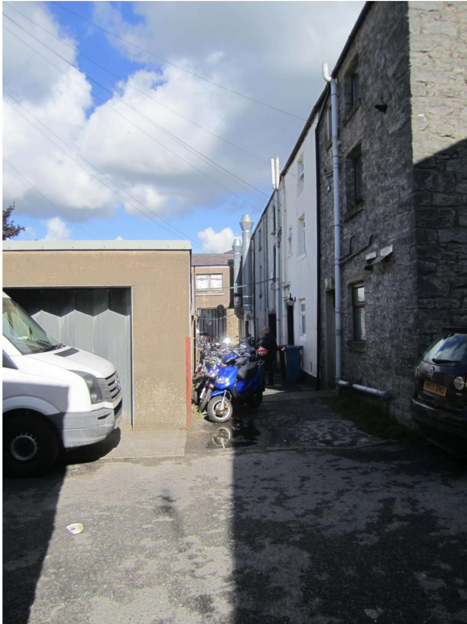
3 Extraction equipment at the rear of 48 and 50 Whalley Road
