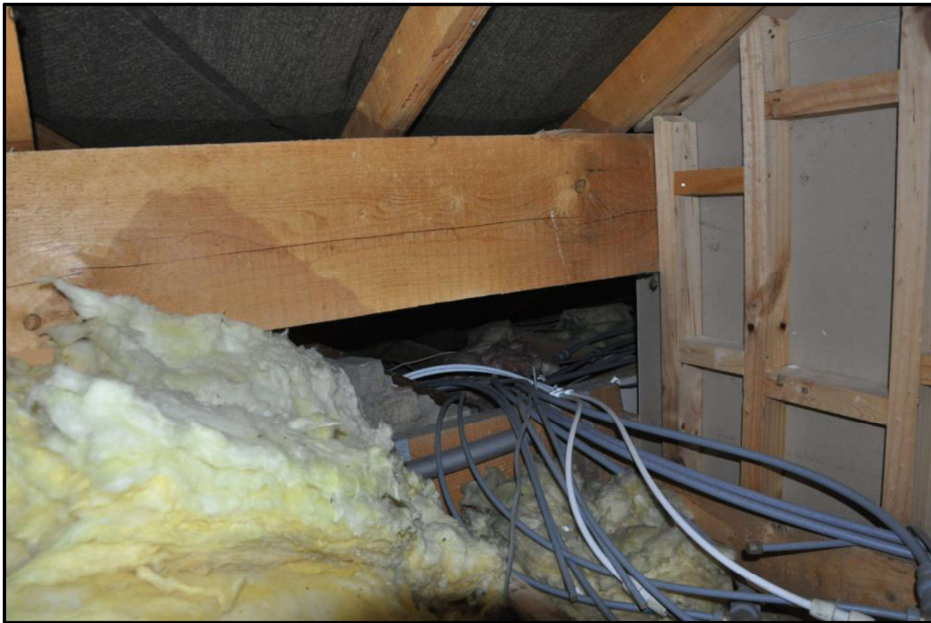
View of roof void above eaves showing intact bitumastic liner and deep rock wool
