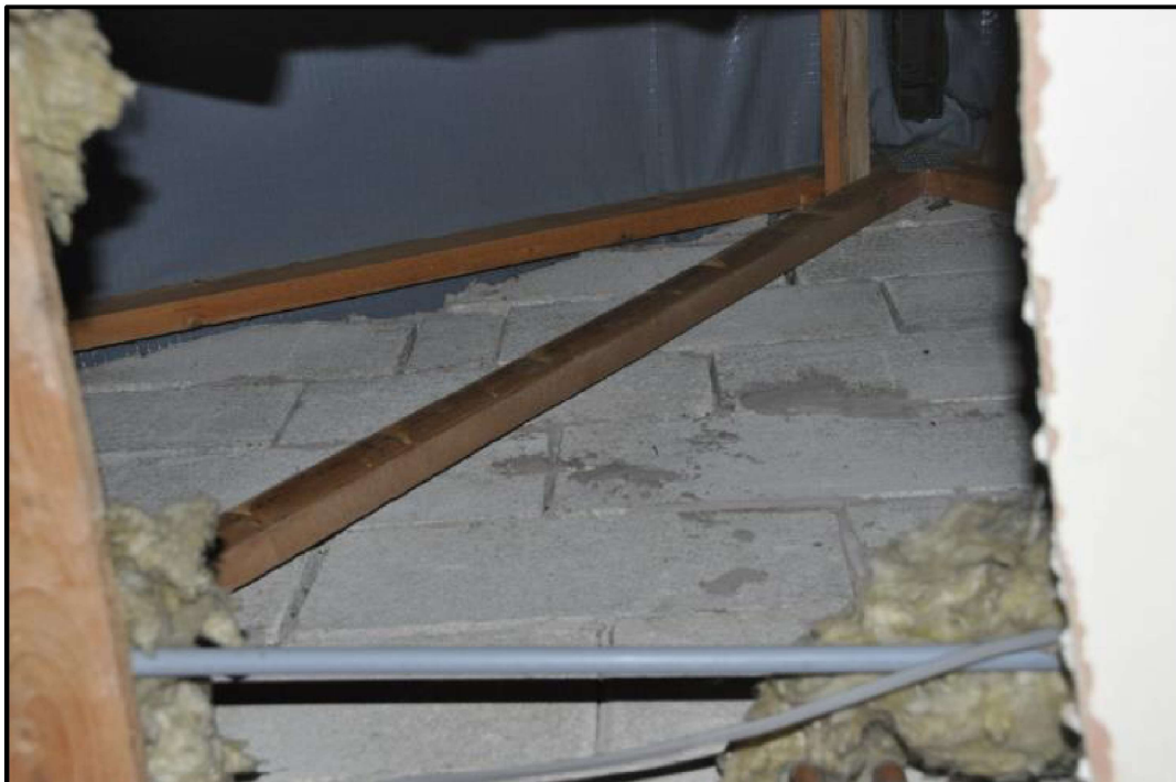
View of void above garage showing plastic roof membrane, rock wool and block walls
