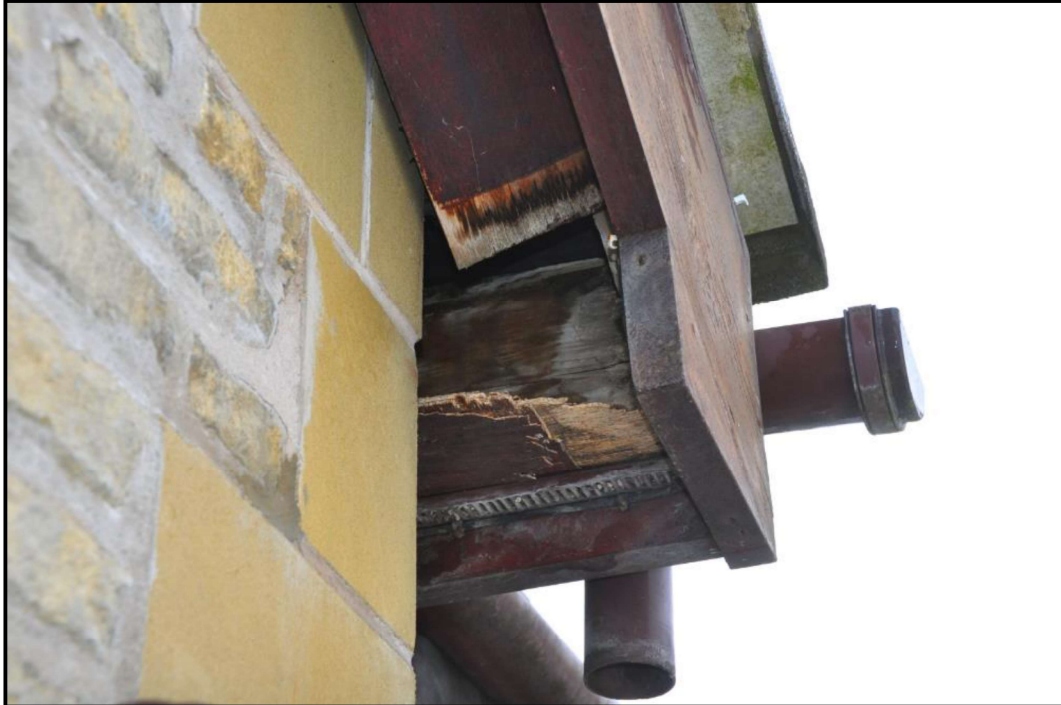
Example of damaged soffit. Gap is suitable for access by nesting birds
