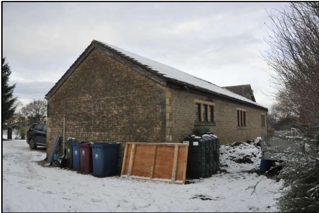
View of south gable of garage, small gaps with some potential for use by bats and birds behind gable soffits
