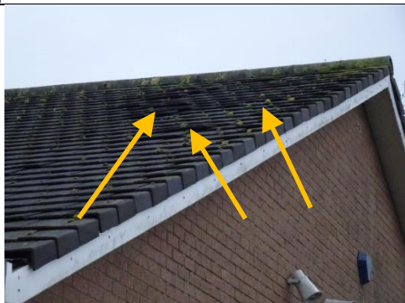
Area of lifted and dislodged tiles
