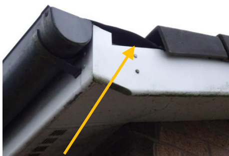
Gap at lower end of dry verge on north-west corner of roof.
