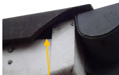
Gap at lower end of dry verge on north-east corner of roof.
