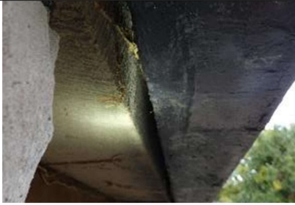
PLATE 9: Gap between wall and beam above the door along the south facing eaves. Gap is approx. 1.5cm wide and 10cm deep and filled with cobwebs.
