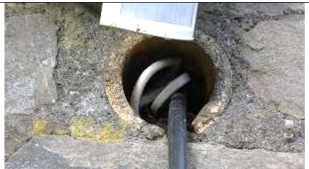
PLATE 8: Terracotta drainpipe ducting under the security light, filled with electrical cable.
