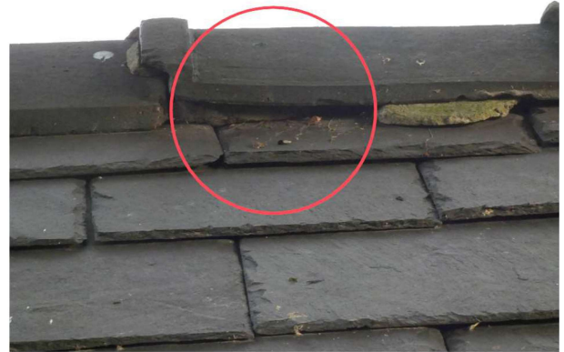
PLATE 10: North facing gap under concrete ridge tile at western end of roof with missing pointing, building B1. 1cm gap x 10cm.
