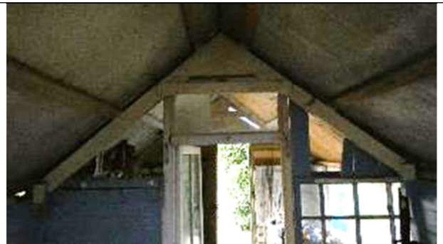
PLATE 22: Looking north-west along the ridgeline of the pitched roof shed. No signs of use were observed during the inspection.
