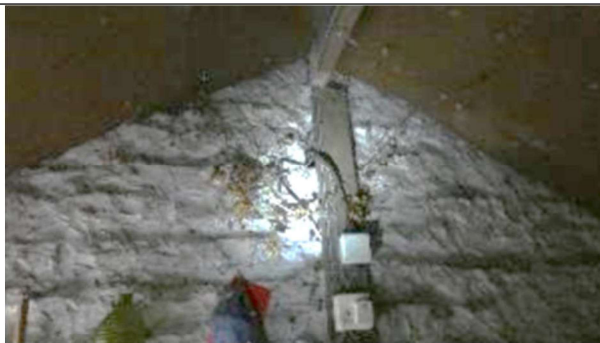
PLATE 13: B1 internal west facing gable end. Clean with light covering of cobwebs. No signs to indicate use by bats.
