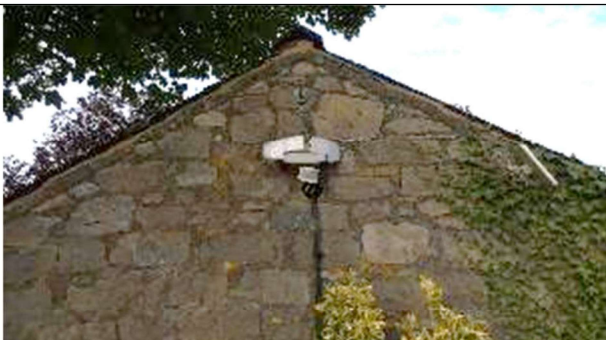
PLATE 7: West facing gable end. Ridge tile with missing dry verge pointing. Cable ducting pipe under a solar powered motion activated security light.
