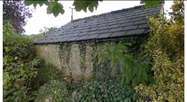
PLATE 4: North facing aspect by Downham Road. Tight fitting eaves few at base of pitched roof, minor ivy cover on wall. Ridge tile at western end with small gap ( )
