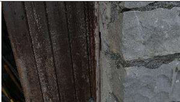
PLATE 11: Ca. <10mm gap, 1m above ground on right side of the south facing door.
