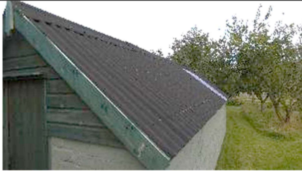
PLATE 17: B2, recently fitted, west facing black bitumen corrugated roof sheet covered roof, with matching ridge material. All materials were tight fitting.
