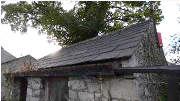
PLATE 15: South facing pitched roof from eastern end. Tiles tight fitting and gable end well pointed.
