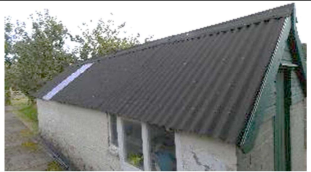
PLATE 18: B2, recently fitted, east facing black bitumen corrugated roof sheet covered roof, with matching ridge material.
