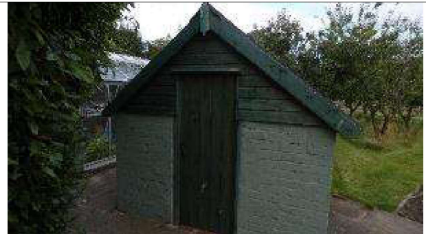
PLATE 16: North facing entrance to B2 of brick built shed. Cladding and gable end
