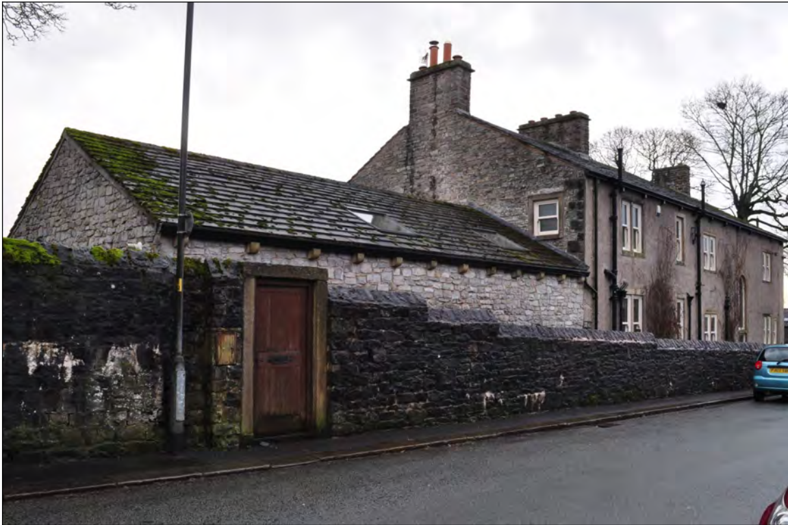
Photo 1: Boundary wall on Downham Road, reduced in height. Rear of Fir Tree House to right.
