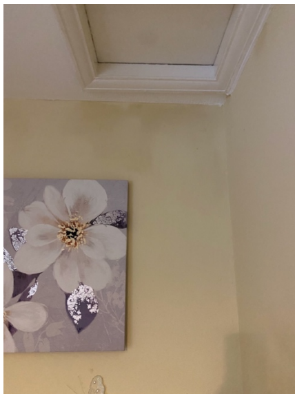
Photograph 3: Rear bedroom gable/ chimney breast inner wall at ceiling junction
