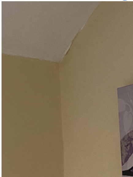
Photograph 1: Rear bedroom gable/ external elevation at ceiling junction
