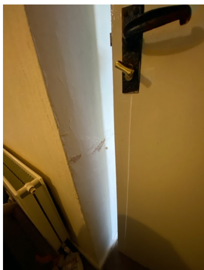
Photograph 6: View onto front door reveal There is evidence of chalking to plaster and paint finish
