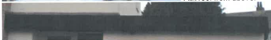
Boarded fascia to garage
