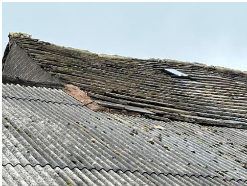
Photograph 3: Example of missing, lifted, broken and slipped tiles; gaps beneath ridge tiles; gaps surrounding skylights; and gaps beneath the lowest row of roof tiles.
