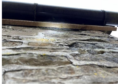
Photograph 7: Example of narrow gap, ranging from 0 cm to approximately 3 cm, between the timber fascia board and the stone elevation.
