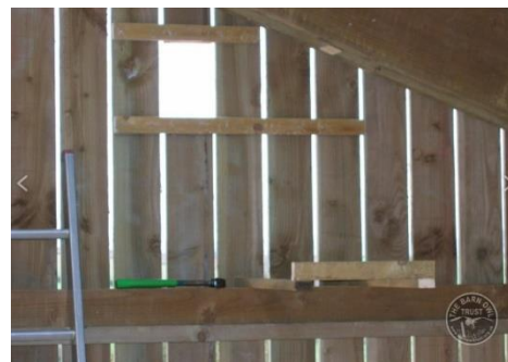
Photograph 20: Opening created for barn owls (with clear view of nest box)
