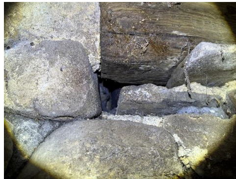
Photograph 14: Example of cracks and crevices present throughout the internal elevations.
