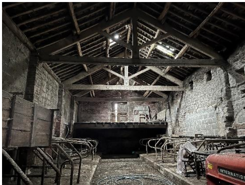
Photograph 13: View of the internal space (central section), showing numerous areas of light ingress due to the state of the roof and skylights. Ledge on the first floor towards the west of the barn.
