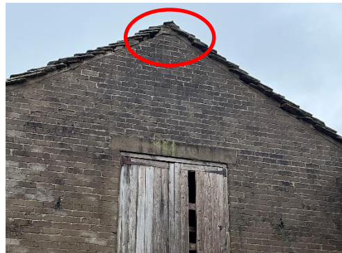
Photograph 4: Example of gaps between and beneath the edge tiles on the gable end. Loading door present on the second floor of the western elevation.
