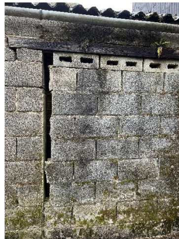
Photograph 9: Narrow gap within the breezeblocks.
