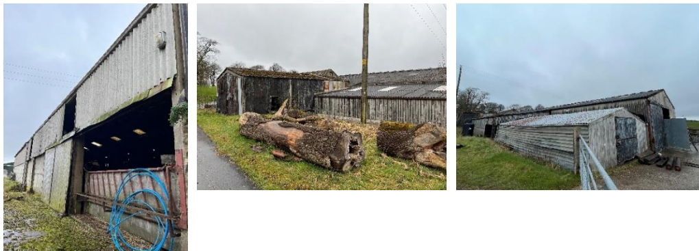
Photographs 10 - 12: External elevations of the eastern two-thirds of the barn which are constructed of large concrete blocks, corrugated sheets and timber cladding.
