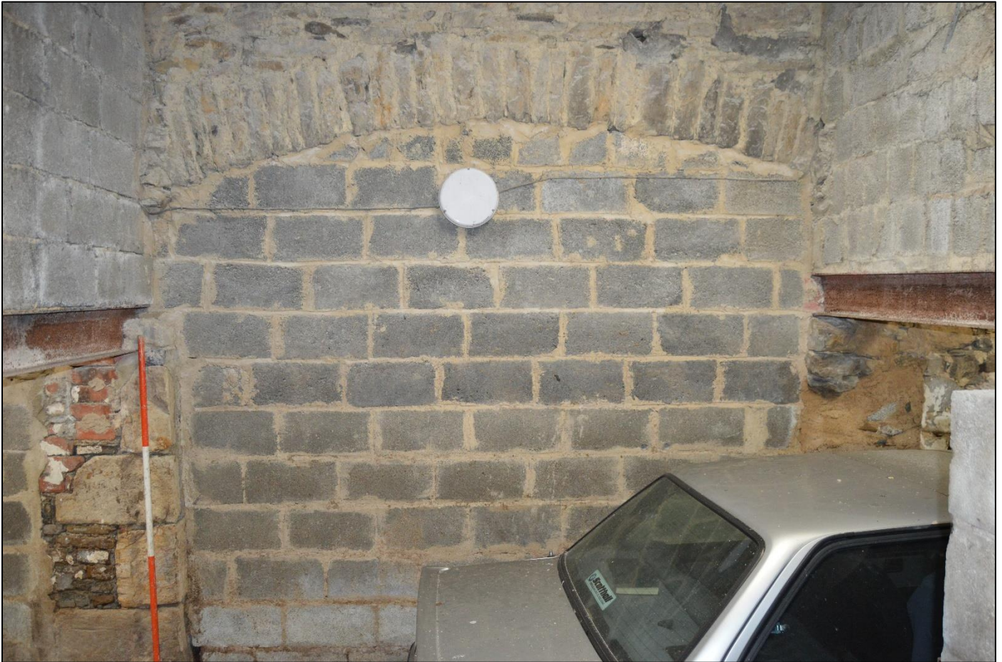
PL37: View of blocked opening with segmental arched head to the north elevation of the original barn.
