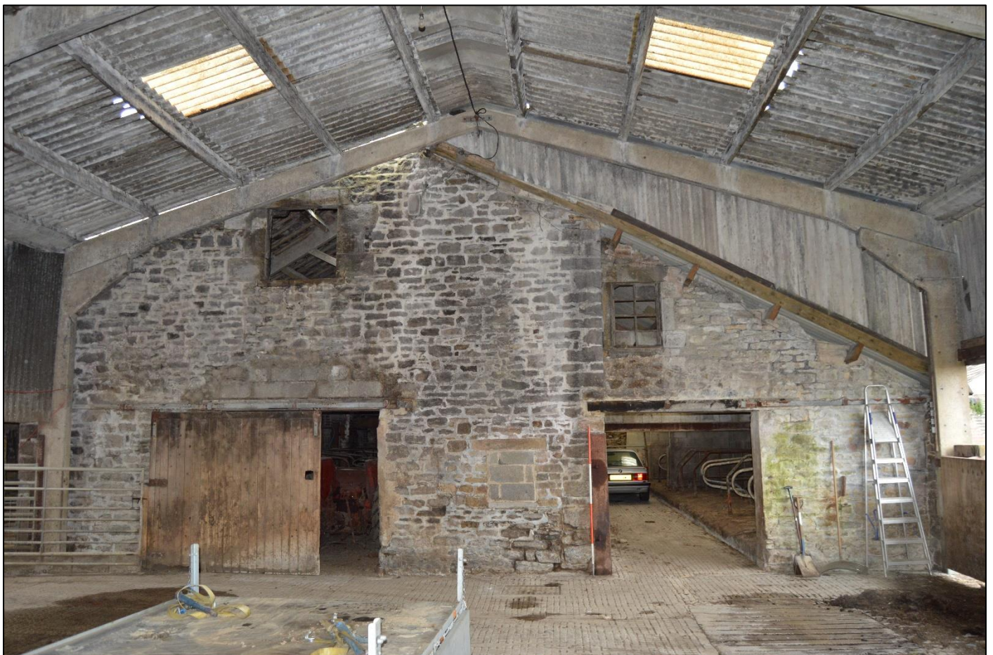
PL24: View of the east elevation of the barn and north outshut from within the modern farm buildings to the east.
