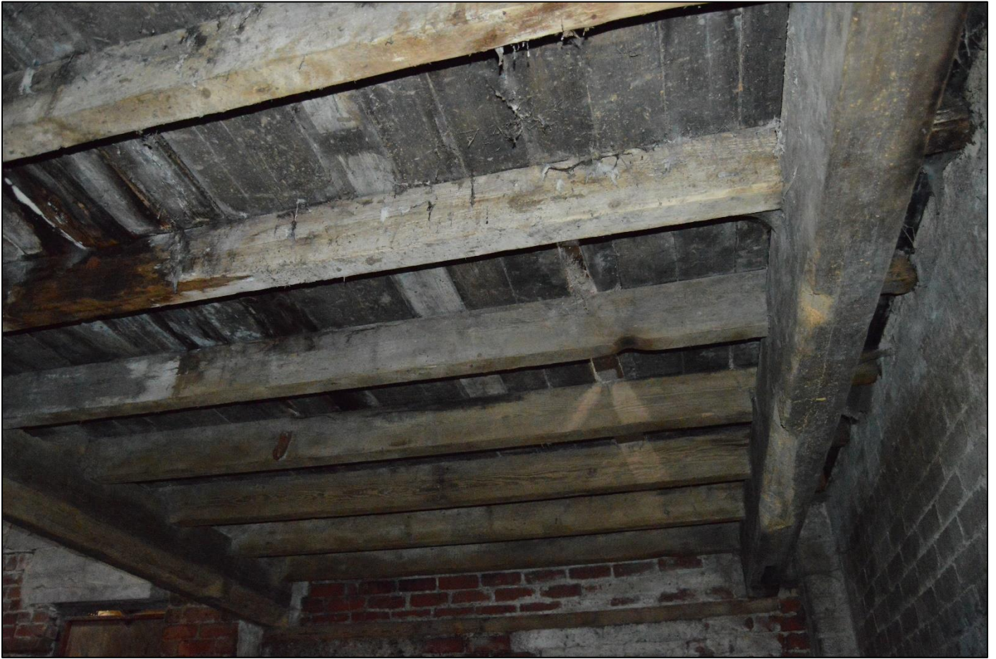
PL48: View of the underside of the hayloft to the west end of the original barn, viewed from the north.
