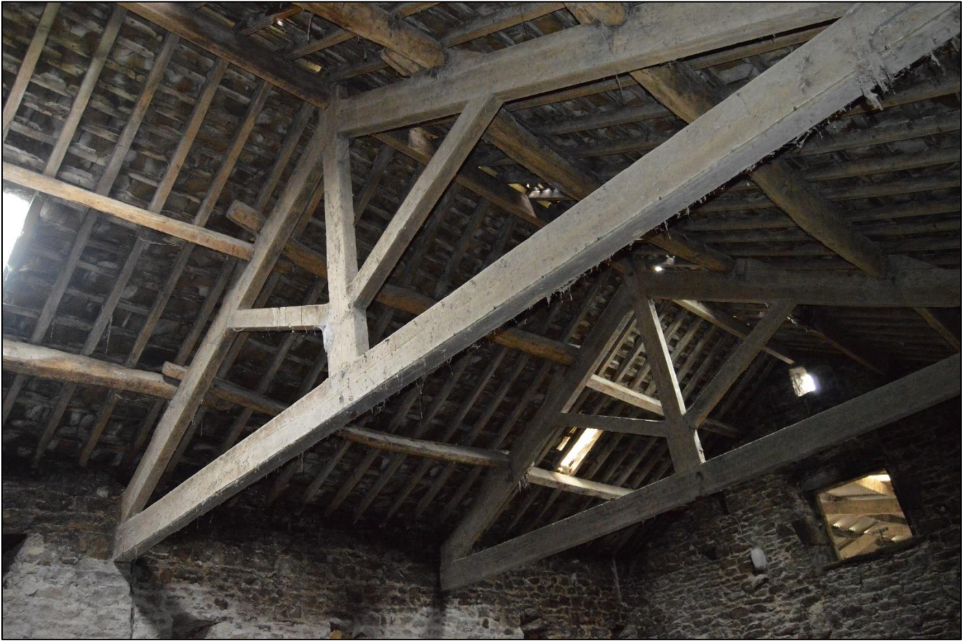
PL54: View of the roof timbers to the north roof slope of the original barn.
