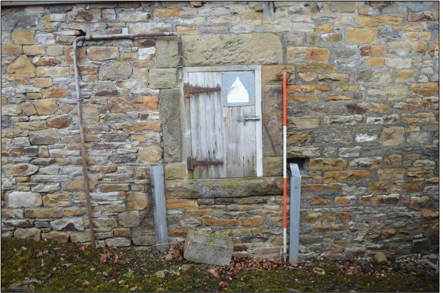
PL13: View of small access / window opening to the north elevation of the north outshut (blocked up internally).
