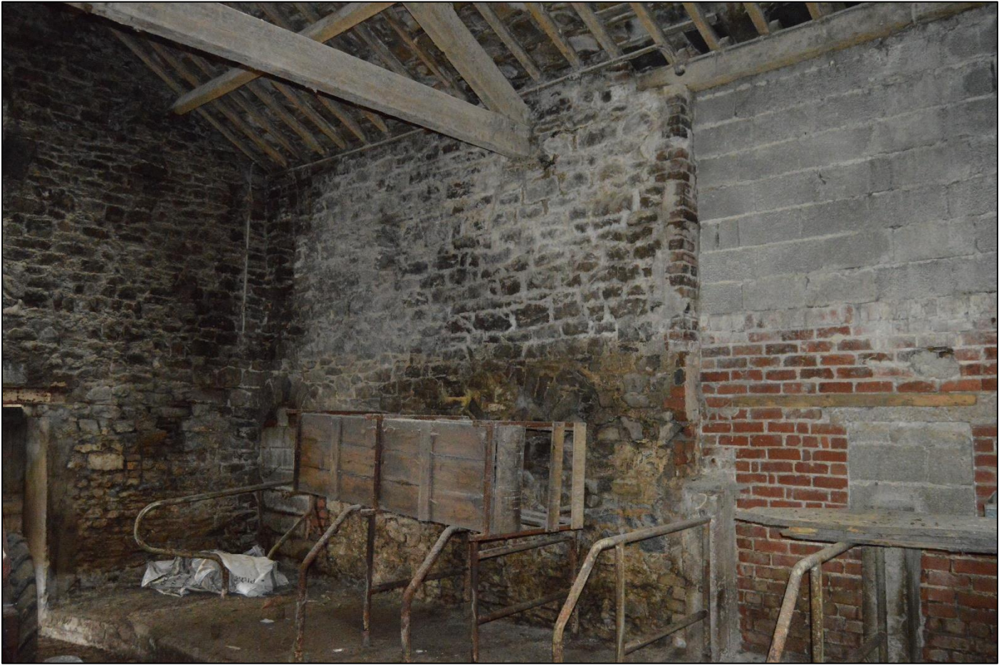
PL42: View of the east end of the south wall of the original barn.
