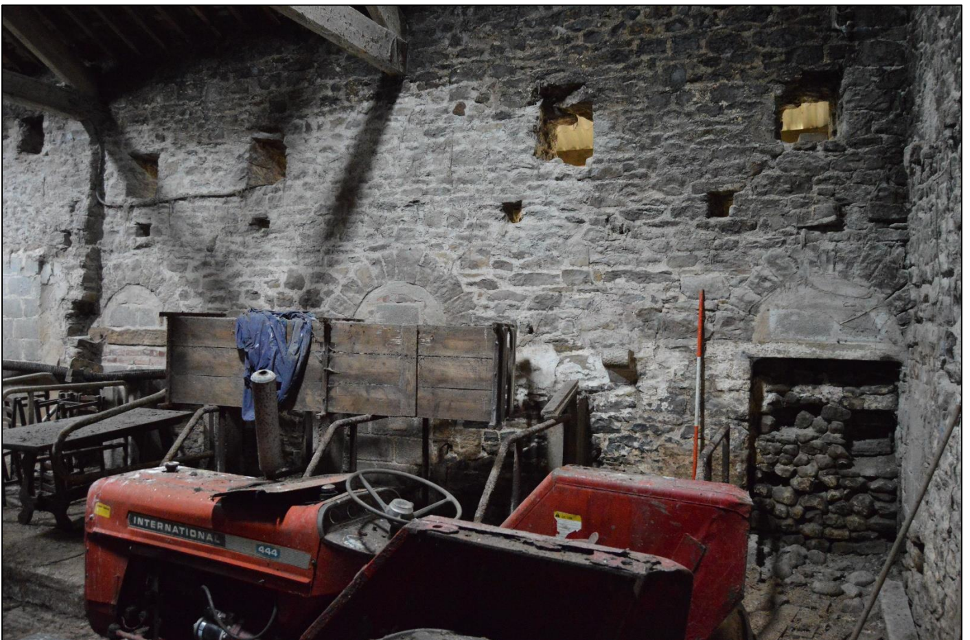
PL45: View of the blocked doorways to the north wall of the original barn.
