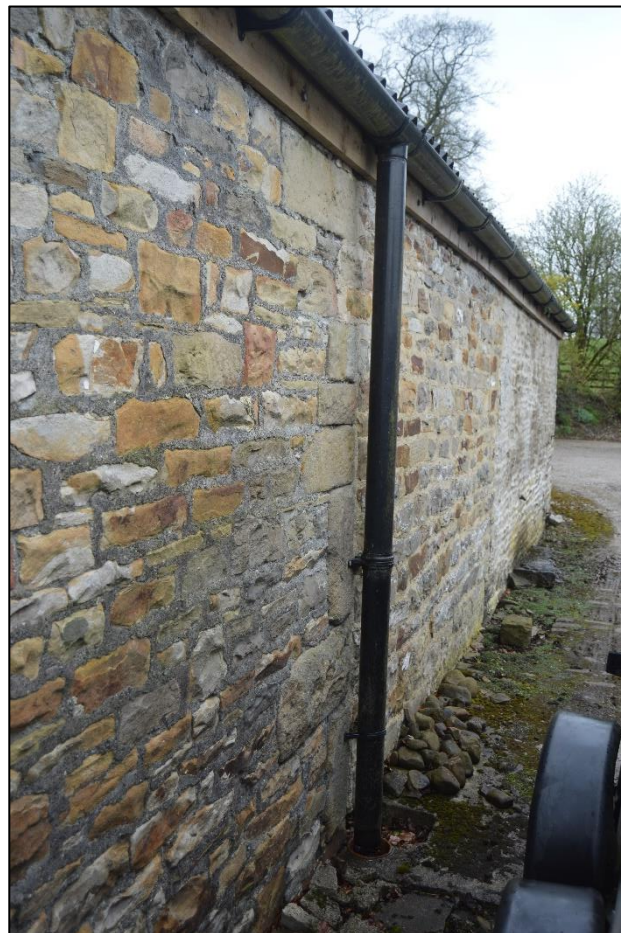
PL14: View of blocked up wall opening to the north elevation of the north outshut.
