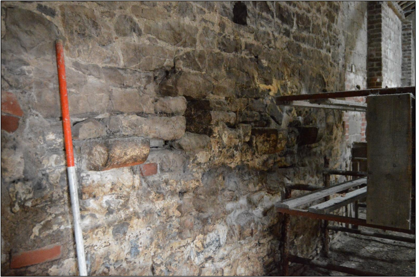
PL44: View of stone corbels to the east side of the south wall within the original barn.
