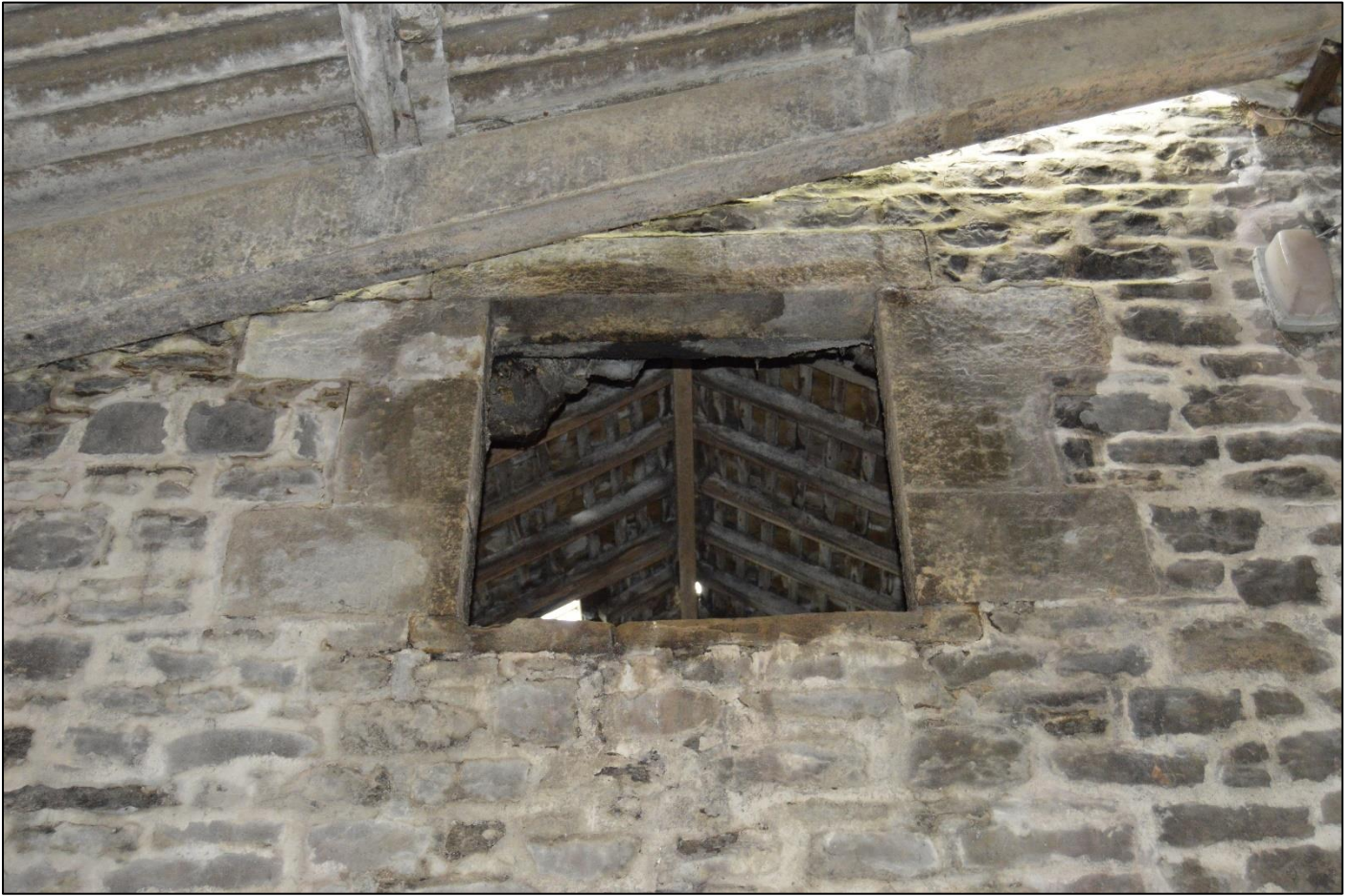
PL29: View of the forking hole at high level to the east gable end elevation.
