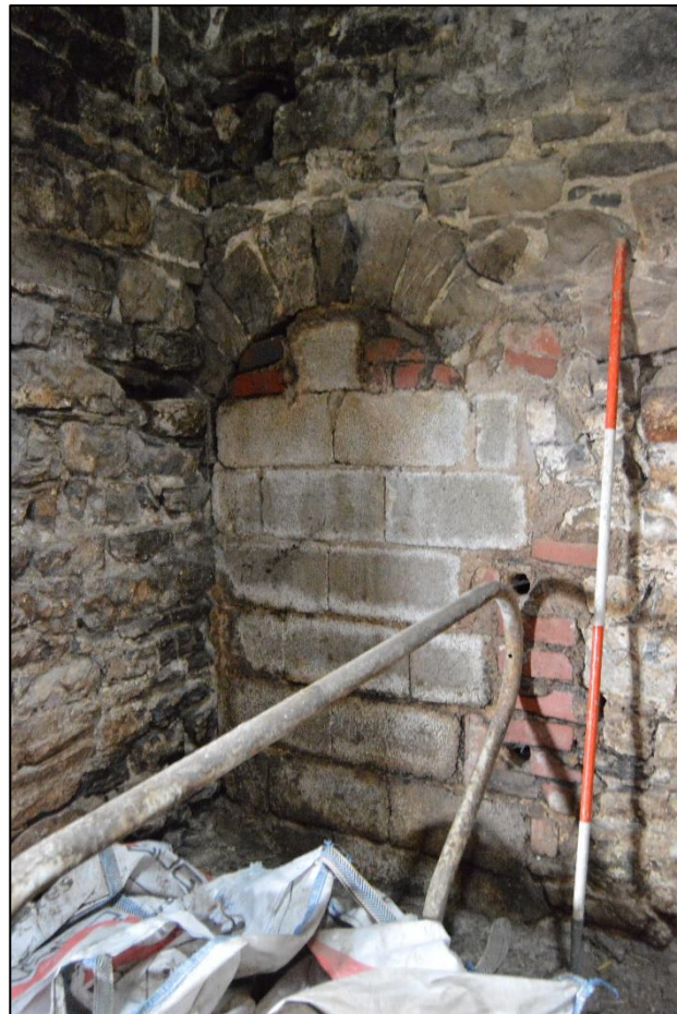
PL43: View of the blocked doorway to the south west corner of the barn.
