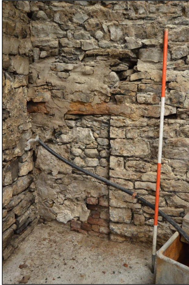
PL19: View of the blocked opening to the west end of the north outshut.
