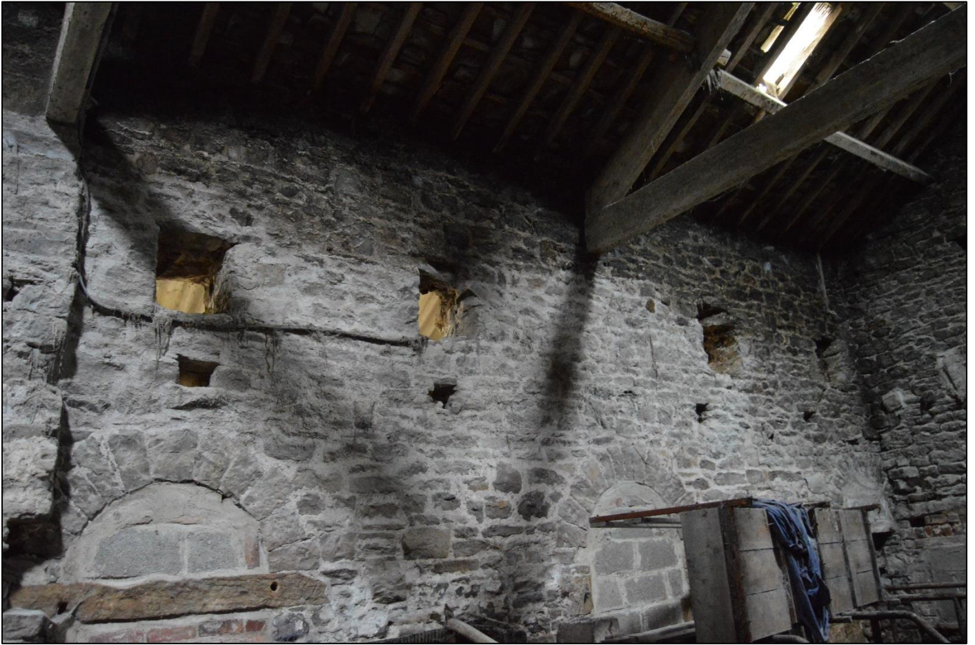
PL46: View of the 'breathers' to the north wall of the original barn.
