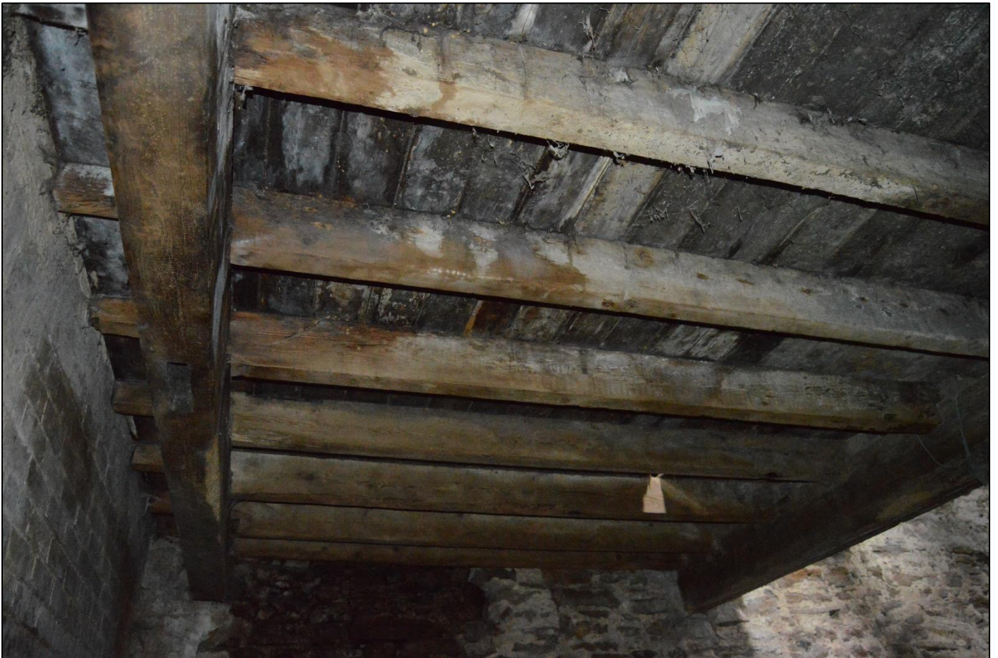
PL47: View of the underside of the hayloft to the west end of the original barn, viewed from the south.
