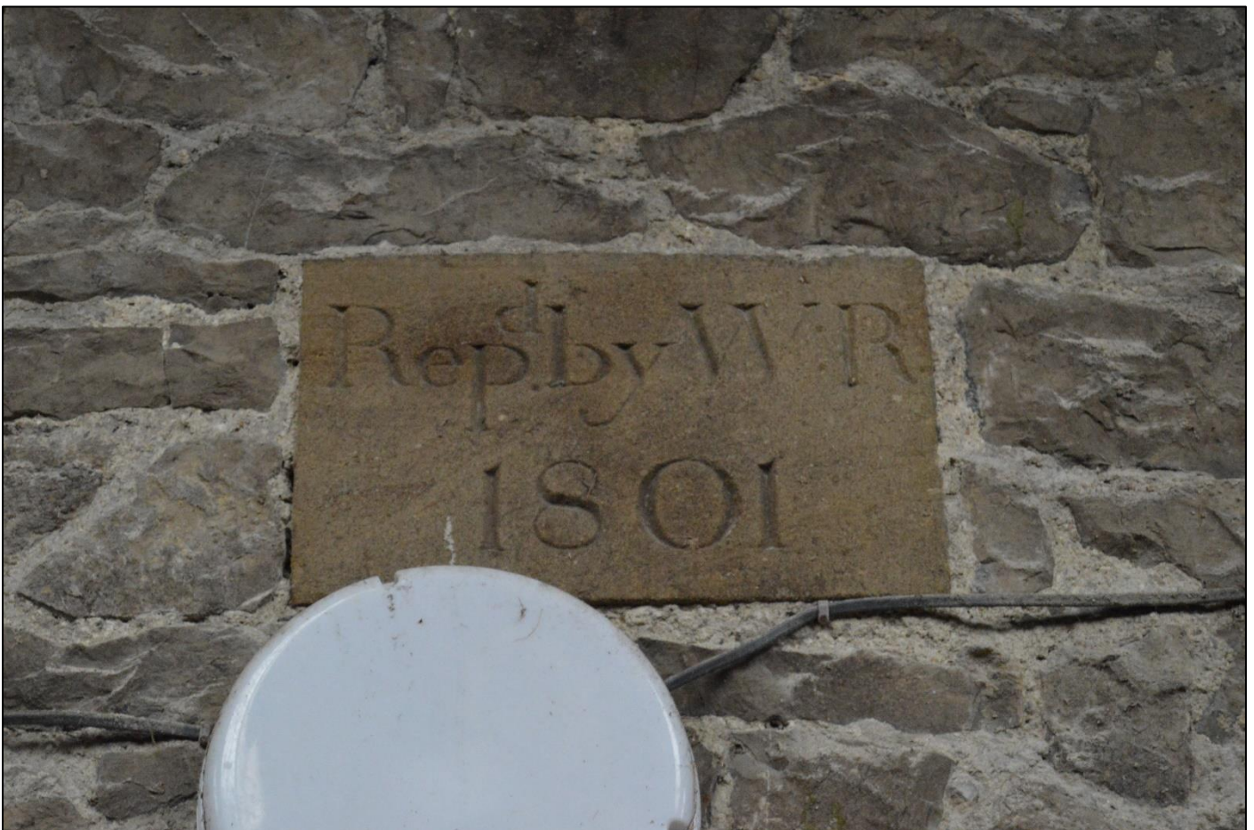
PL36: View of the datestone present to the north elevation of the original Barn inscribed 'Rep'd by W.R. 1801'.
