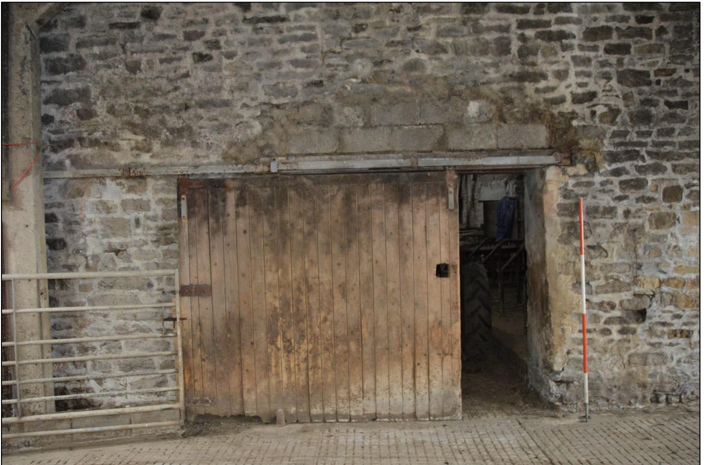
PL28: View of the formed sliding door opening to the east gable end of the original barn.
