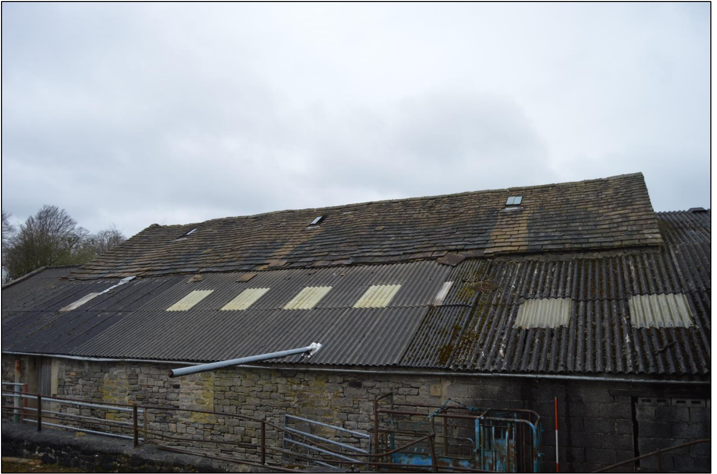
PL11: View of the stone flag roof covering to the south roof slope of the barn.
