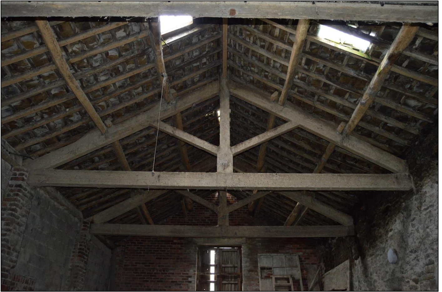
PL52: View of king post roof trusses over the west end of the original barn.
