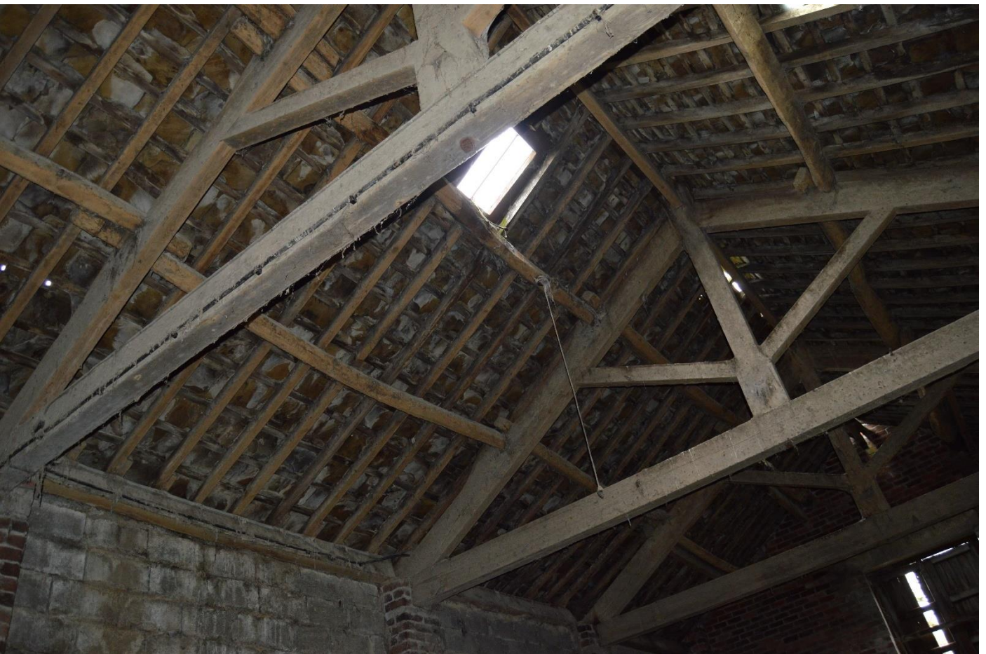
PL53: View of the roof timbers to the south roof slope of the original barn.
