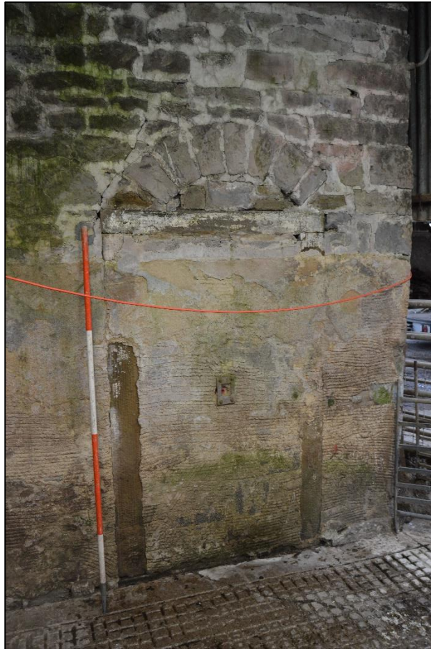
PL23: View of the blocked doorway to the south elevation of the original barn.
