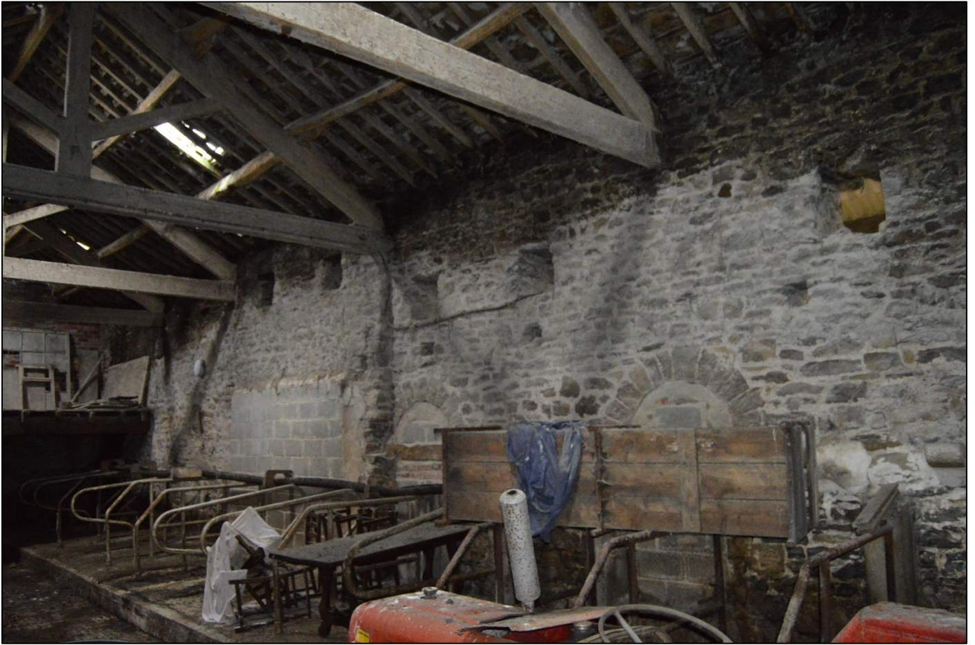
PL39: View of the north wall of the original barn from the south west.
