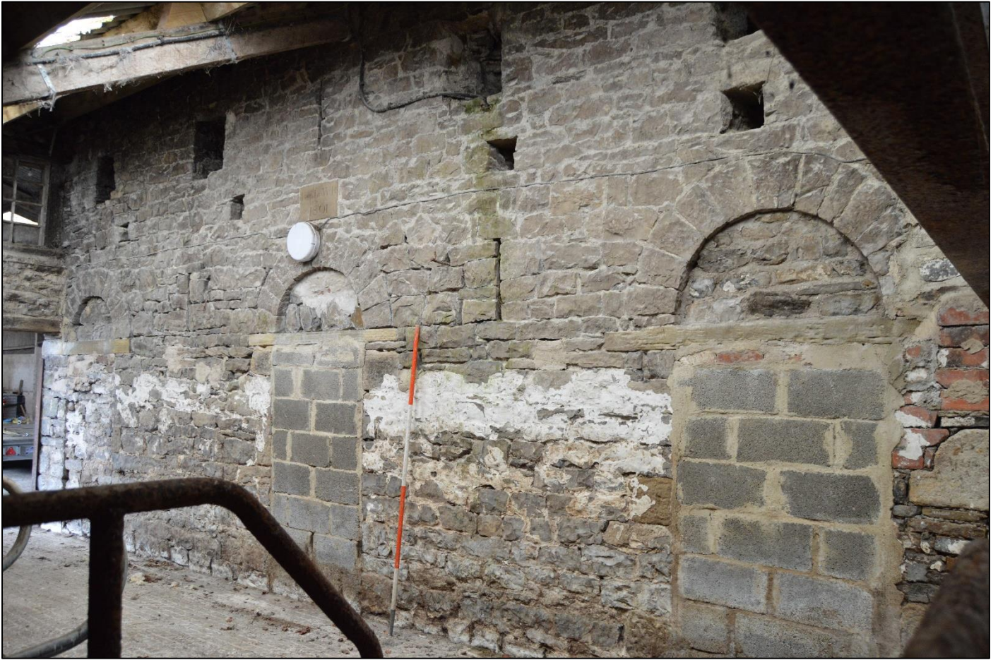
PL31: View of three blocked doorways, with segmental arched heads to the north elevation of the original barn.
