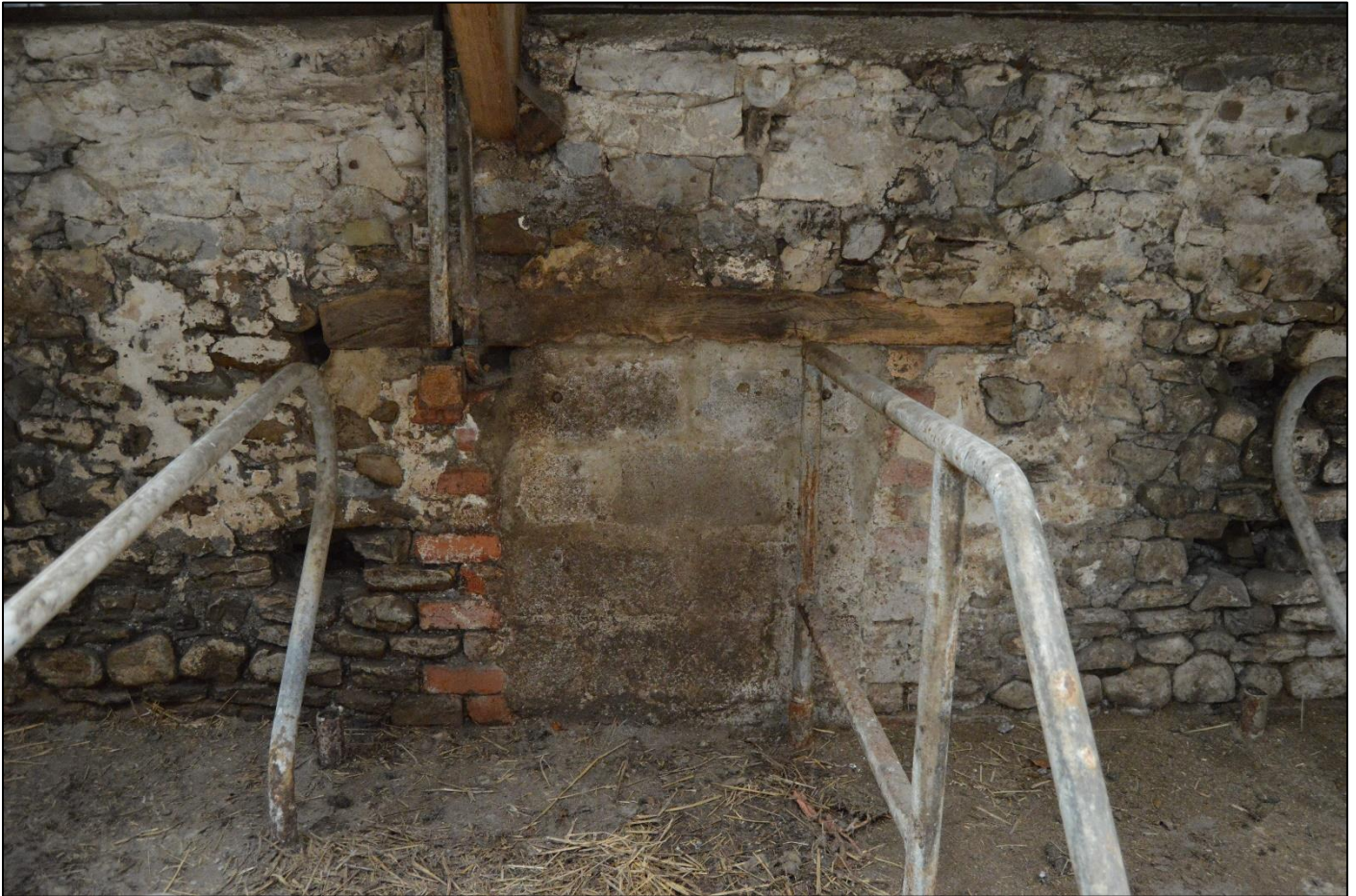
PL35: View of the blocked opening to the north elevation wall of the north outshut.
