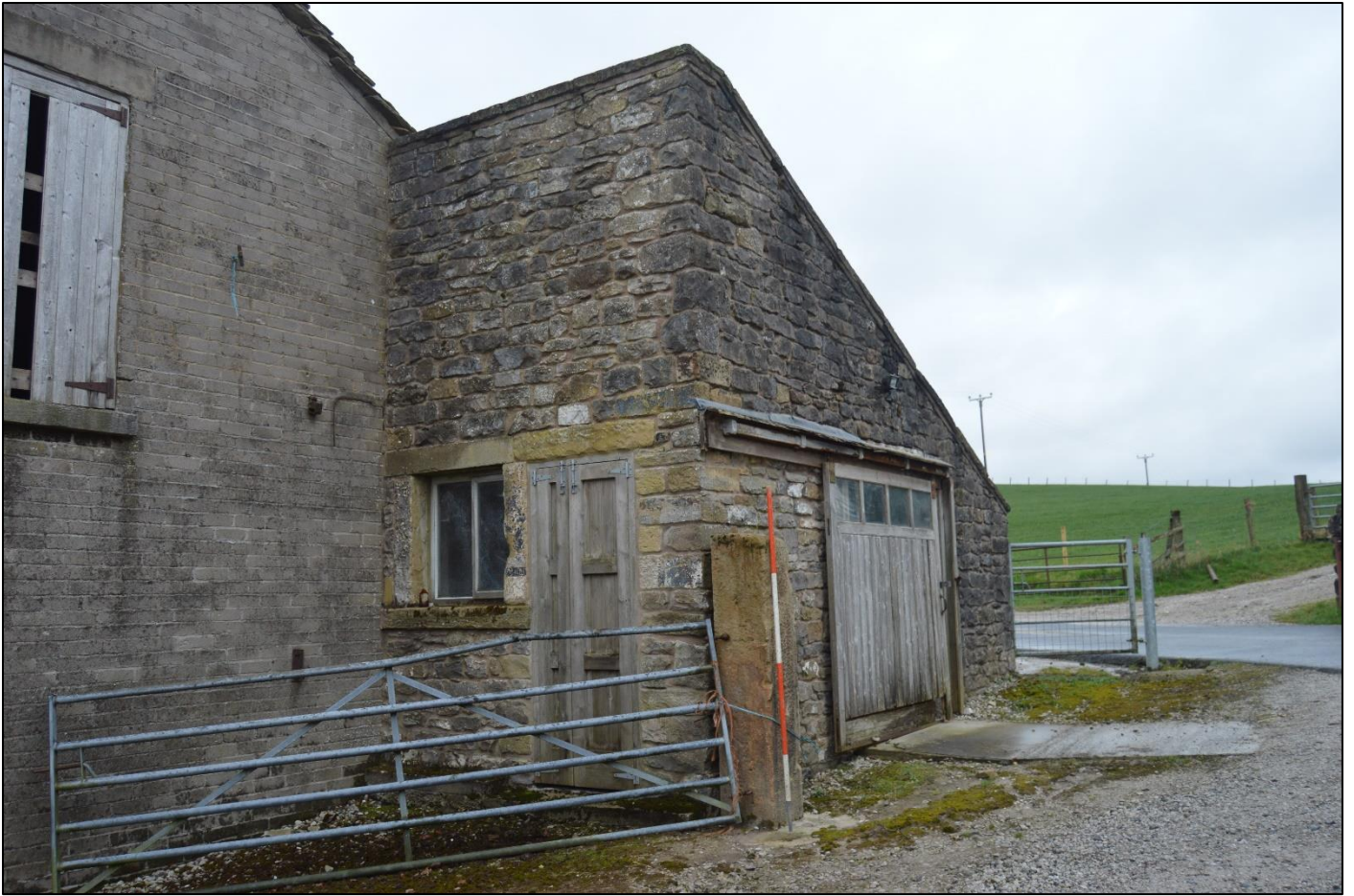
PL05: View of the extension to the south outshut from the north west.
