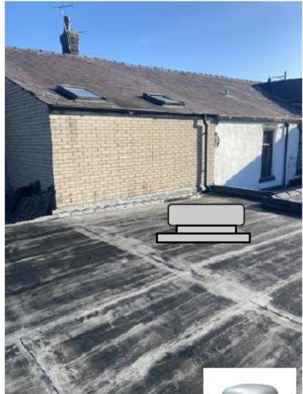
Air input cowl mounted on the roof as shown
