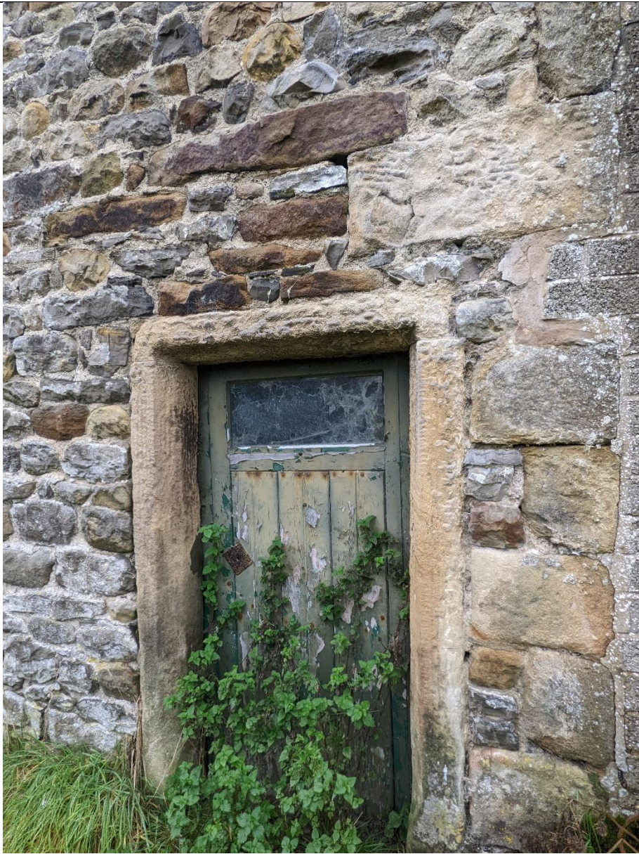
Gale wall, sandstone door surround is weathered, but not structurally significant. Blockwork to shipon block bonded into stone coins.
