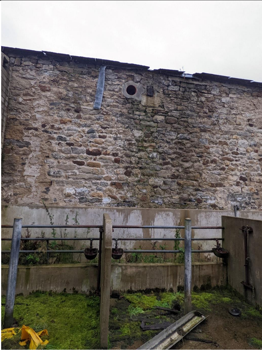
Rear elevation, missing tiles at eaves and gutters, allowing water to run down the wall. Pointing is in reasonable condition.
