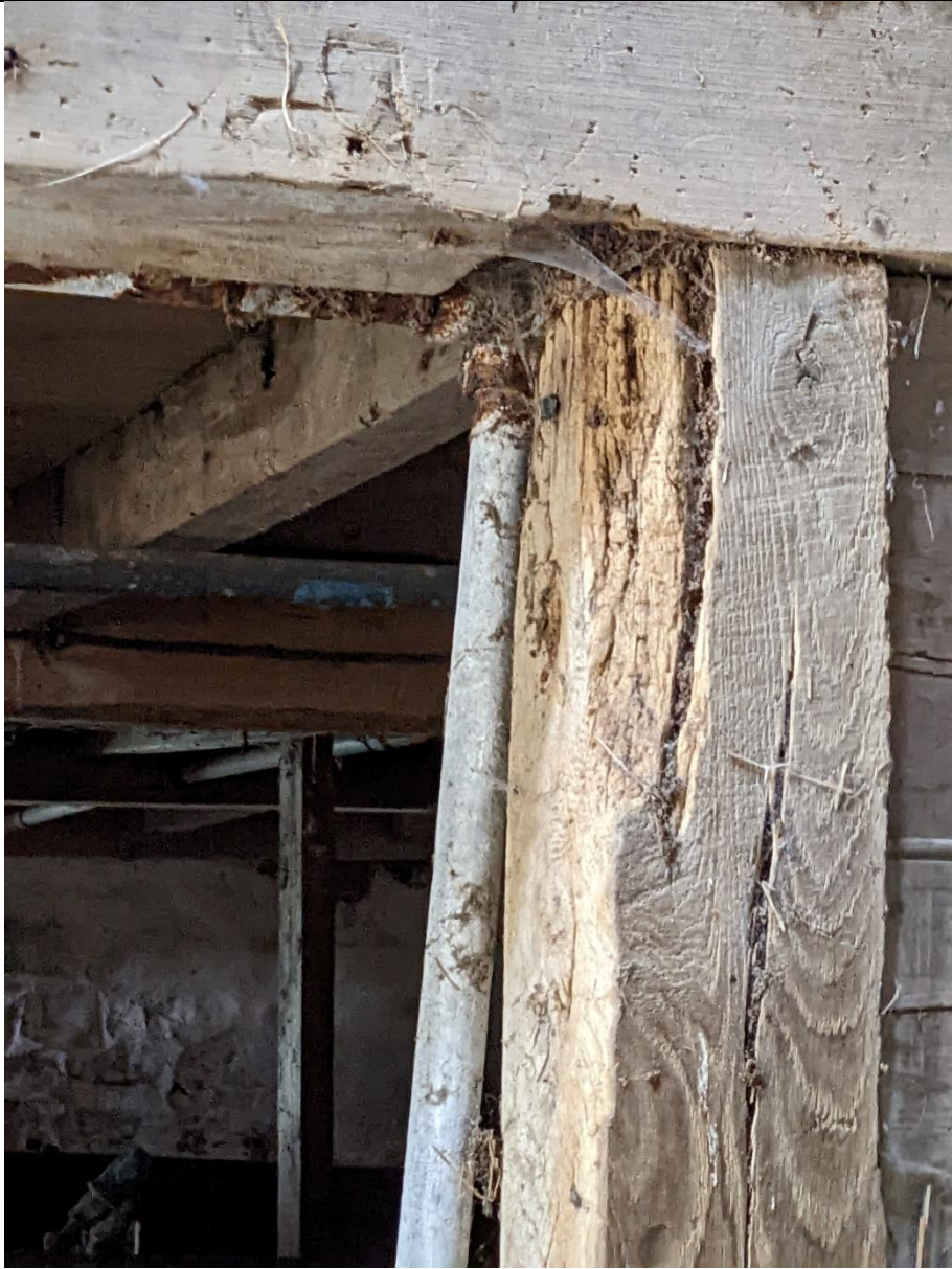
Woodwork affected timber in stalls
