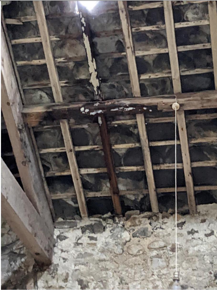
Suspected rot in purlin and rafter due to water ingress.
