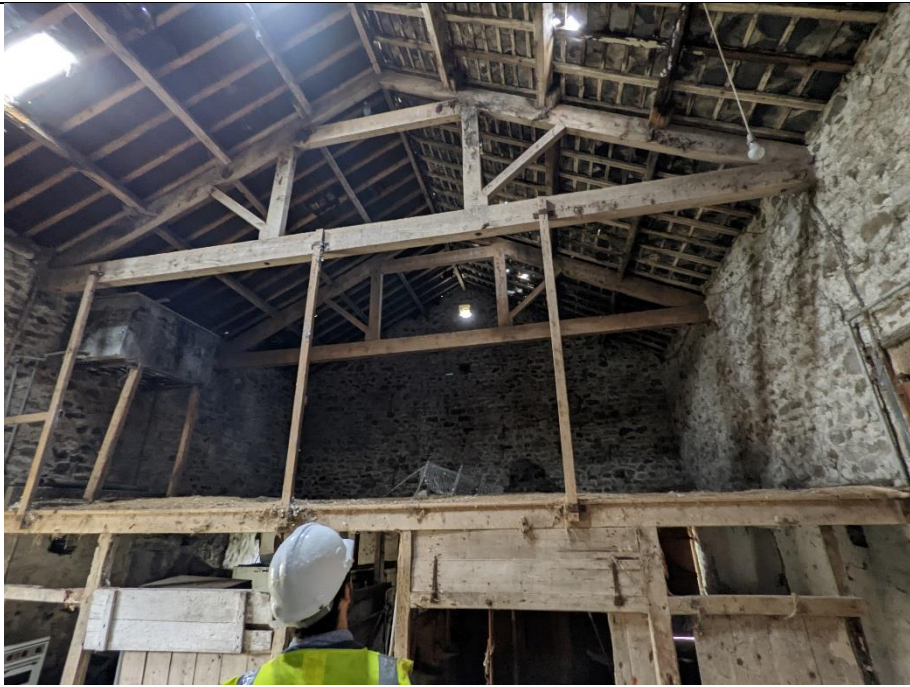
Interior view showing trusses, and hayloft. Note holes in roof.
