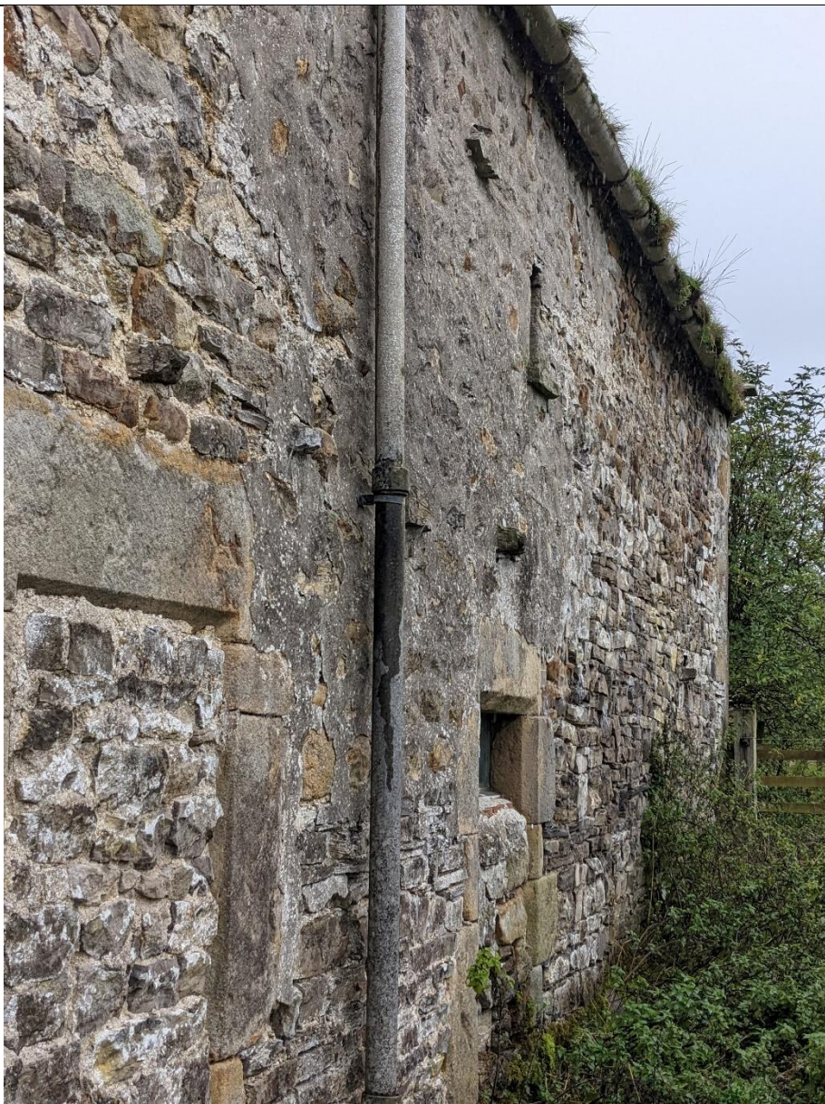
Rear elevation- vegetaion in gutters to be cleared and downpipe repaired.
