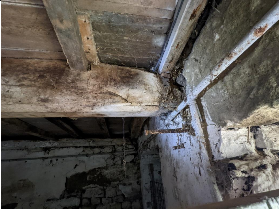
Timber beam supporting loft in left hand room, loss of section from rot at bearing in front wall.
