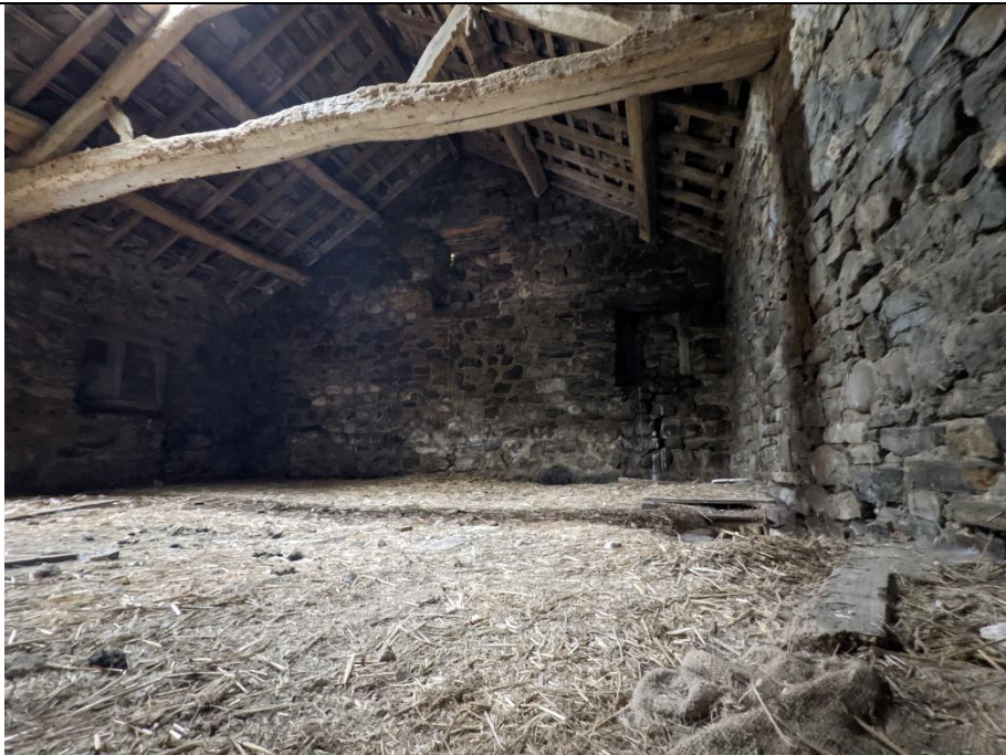
View into loft from hatch. Floor is uneven. Roof appears intact. Rustic truss appears affected by woodworm. Floor is uneven. Not entered, due to condition of timbers viewed from below.
