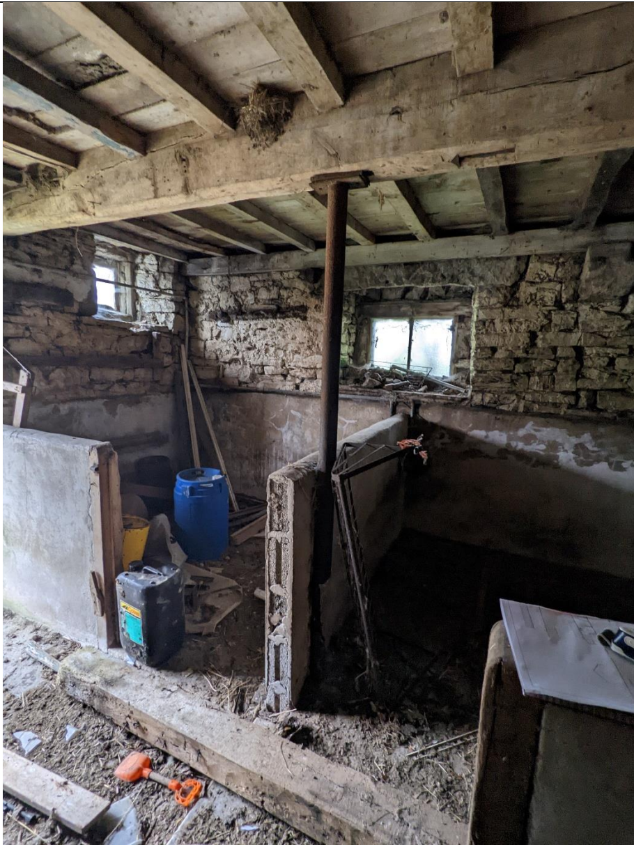
Steel prop installed under timber beam. Note bottom 1/3 rd of prop is missing due to corrosion..
