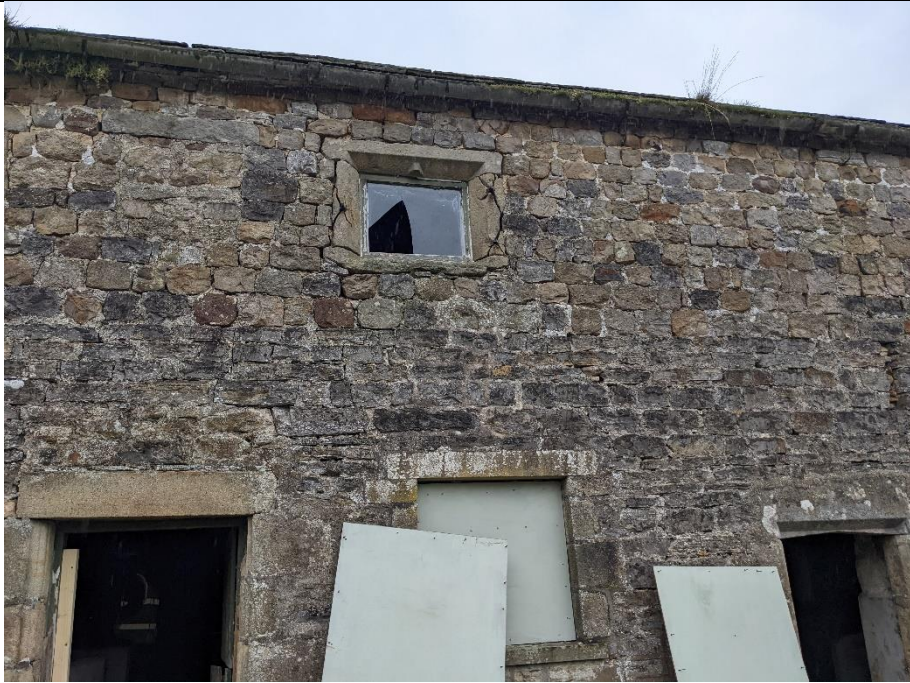
Front elevation, broken stone jambs to first floor window
