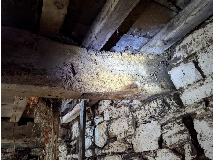
Timber Beam supporting loft in left hand room. Affected by woodworm. Loss of effective section to be confirmed.
