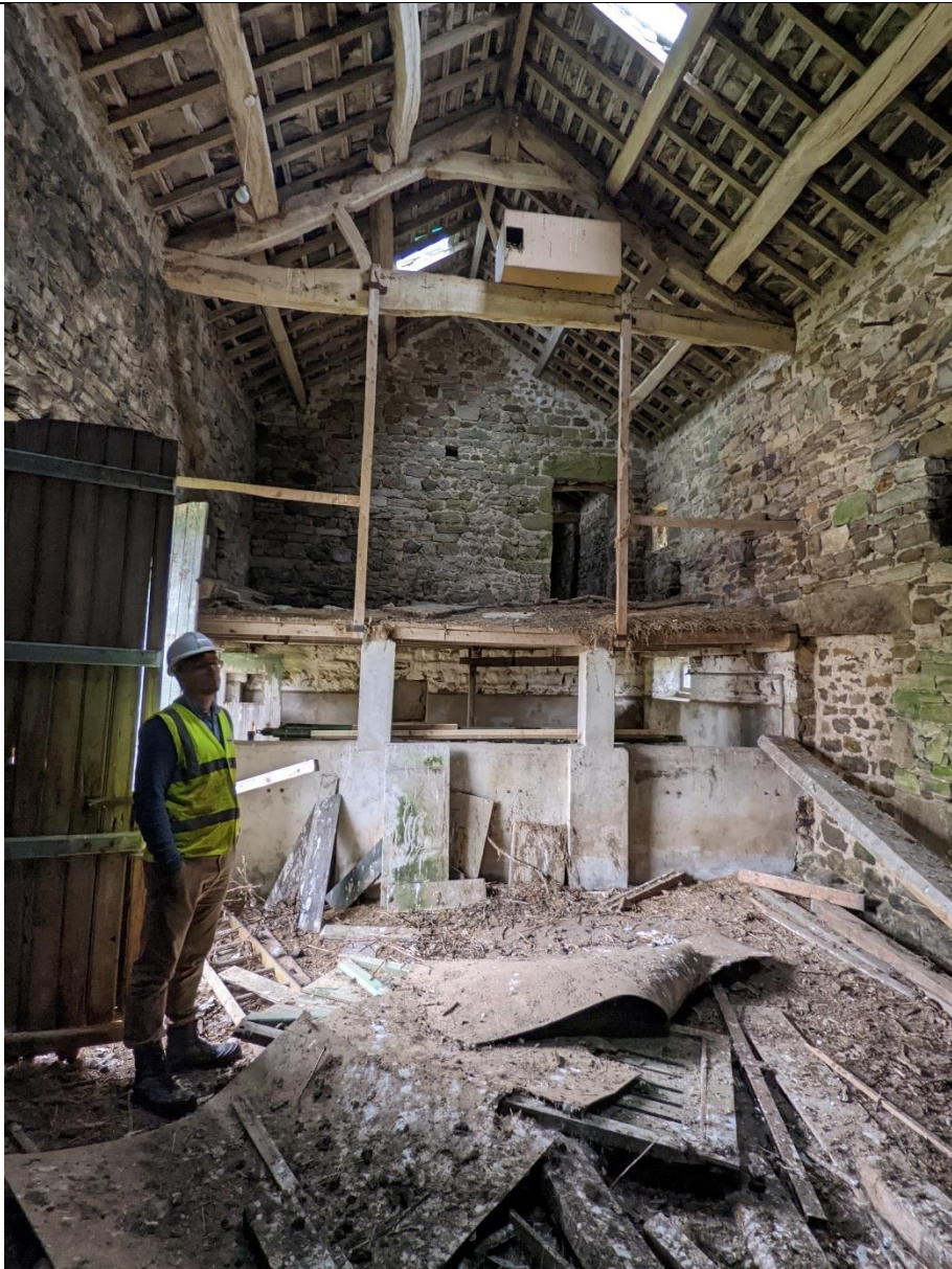
View back to the loft in the main barn. Some purlins seem original hewn beams. Walls reasonably plumb.
