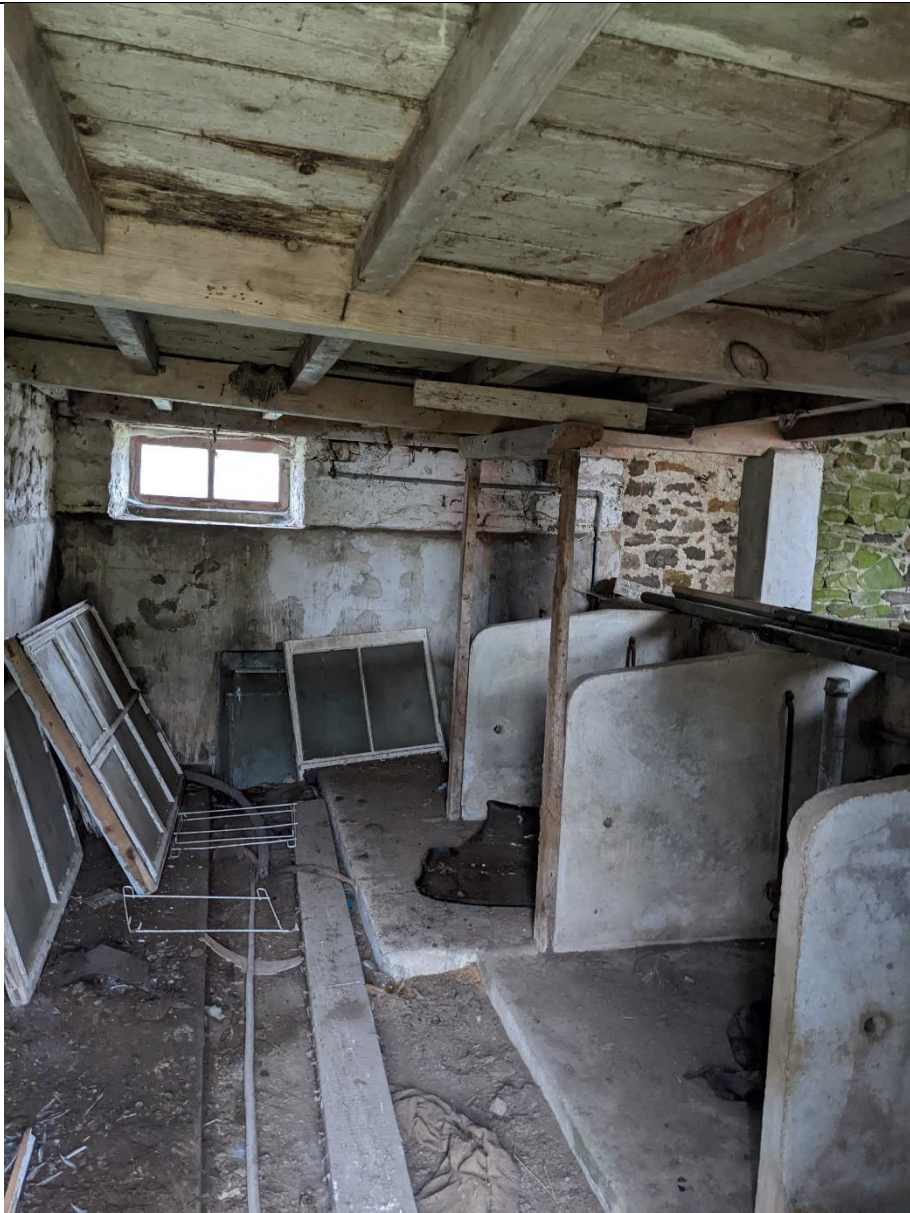
View into stalls in middle portion of barn. Timbers to loft over appear in reasonable condition, not original.
