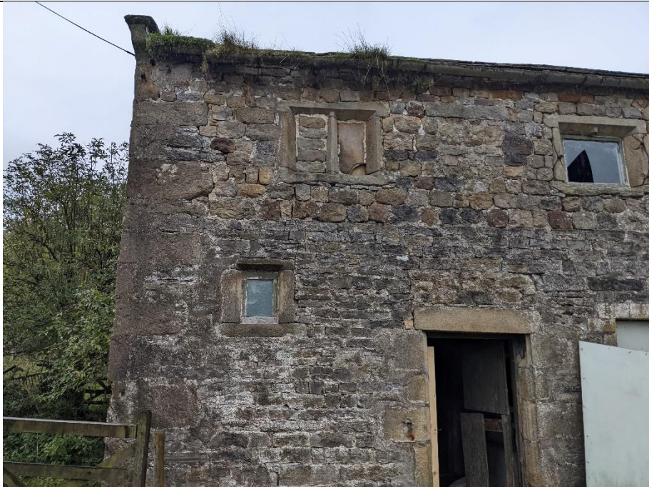
Front elevation, left. Infilled window to first floor, vegetation in gutter.
