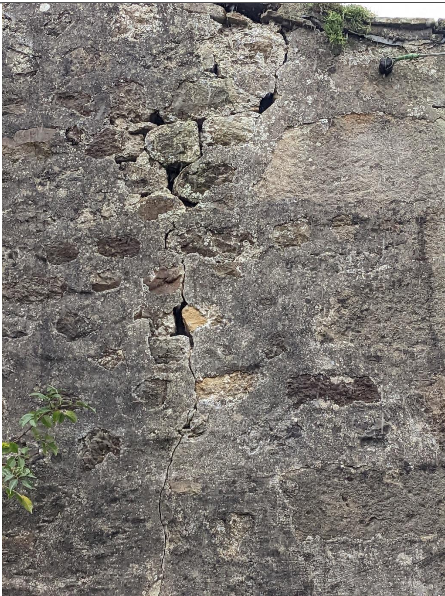
Crack in west gable at verge near south kneeler stone.
