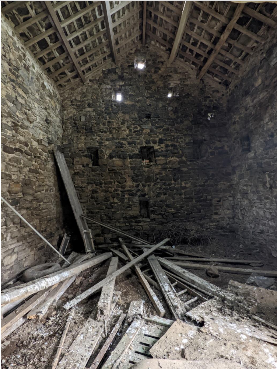
View in main barn. Roof timbers appear in reasonable condition. Top of walls appear to have been recently re-pointed, possibly at the time of ree-roofing. No sarking felt.
