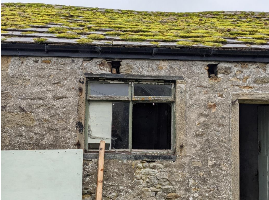
Close up on front window with timber lintel, which may be considered for replacement
