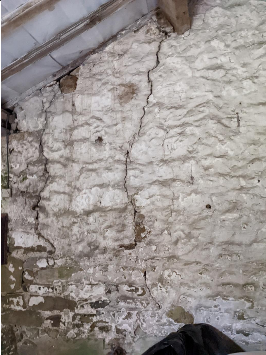
Internal wall, vertical cracks emanating from purlin bearings
