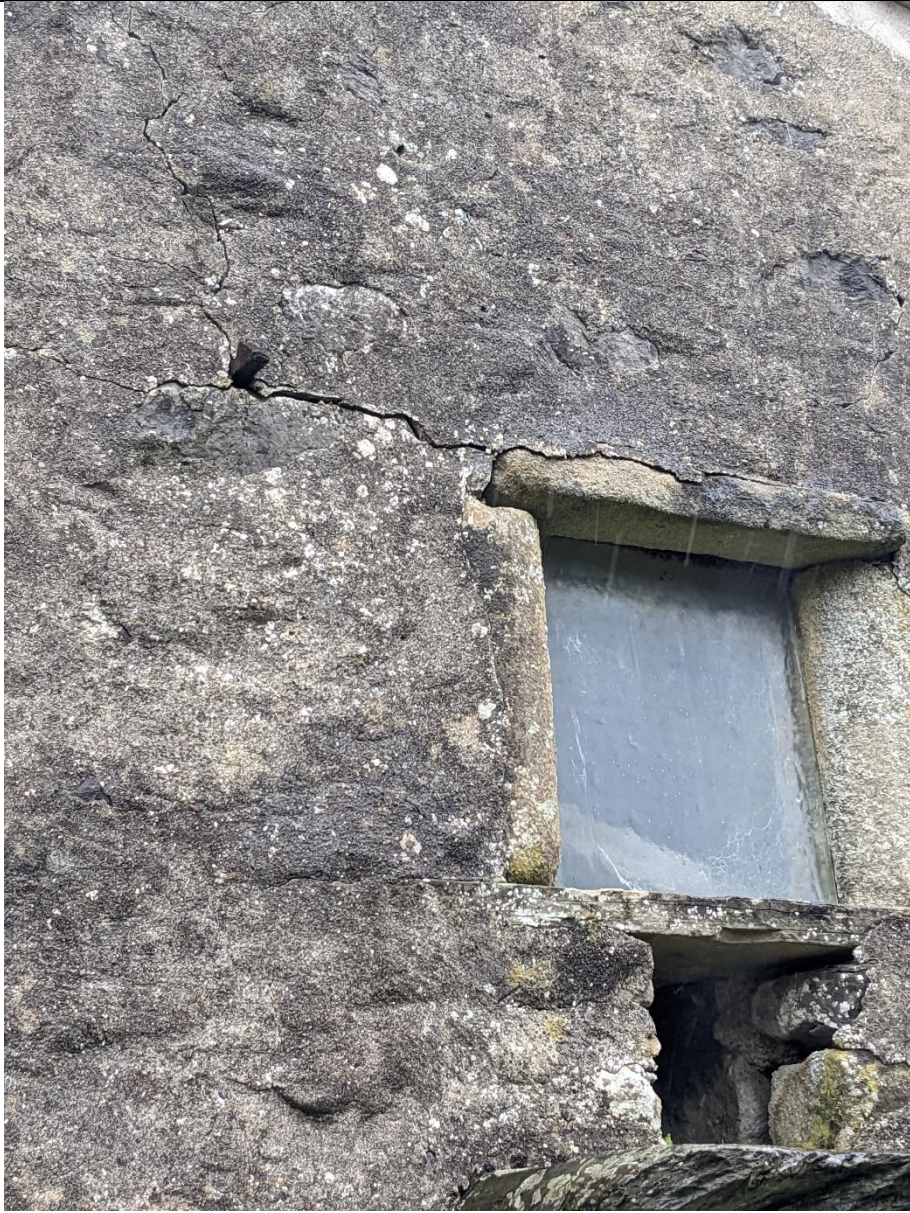
Crack in RH gable wall between stone lintel and masonry wall.
