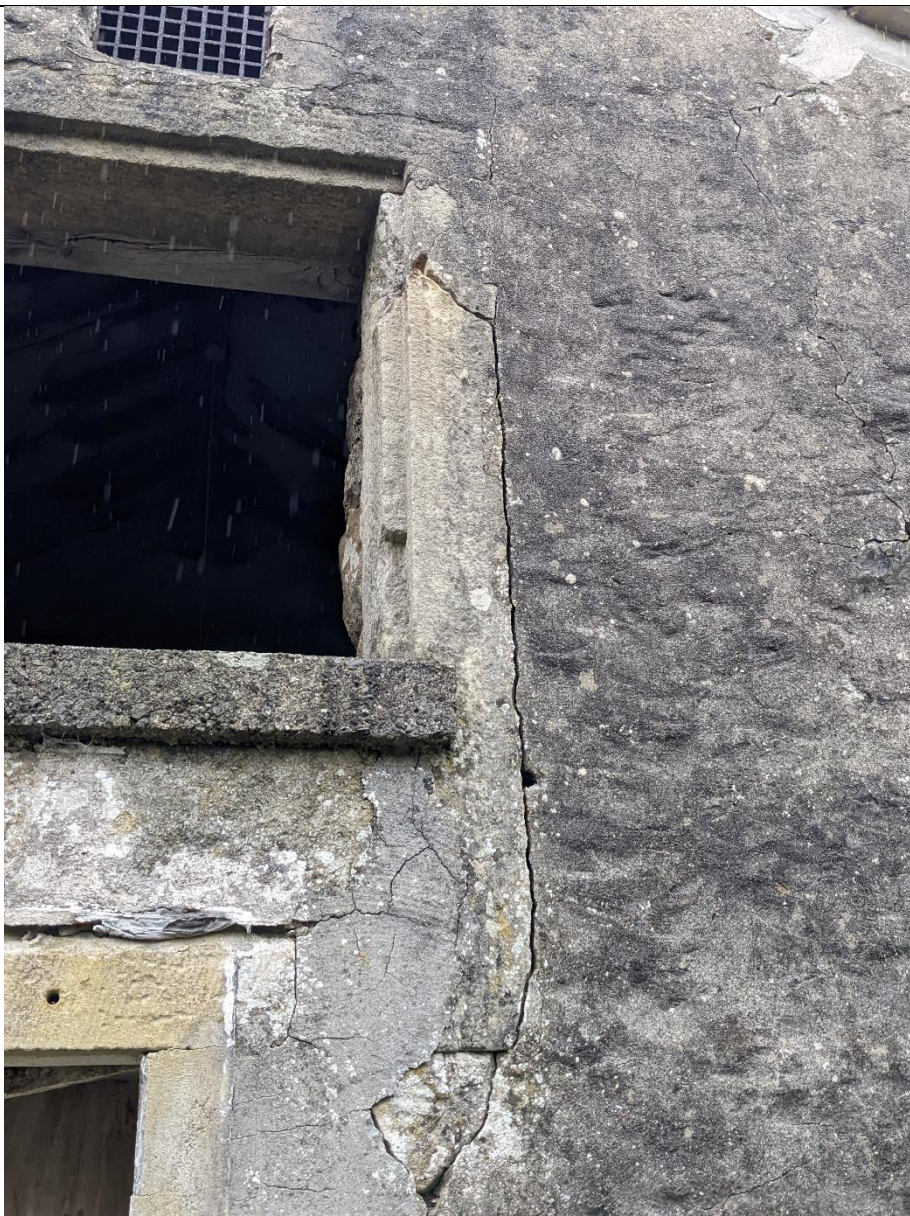
Crack in right hand gable between RH stone jamb and masonry.
