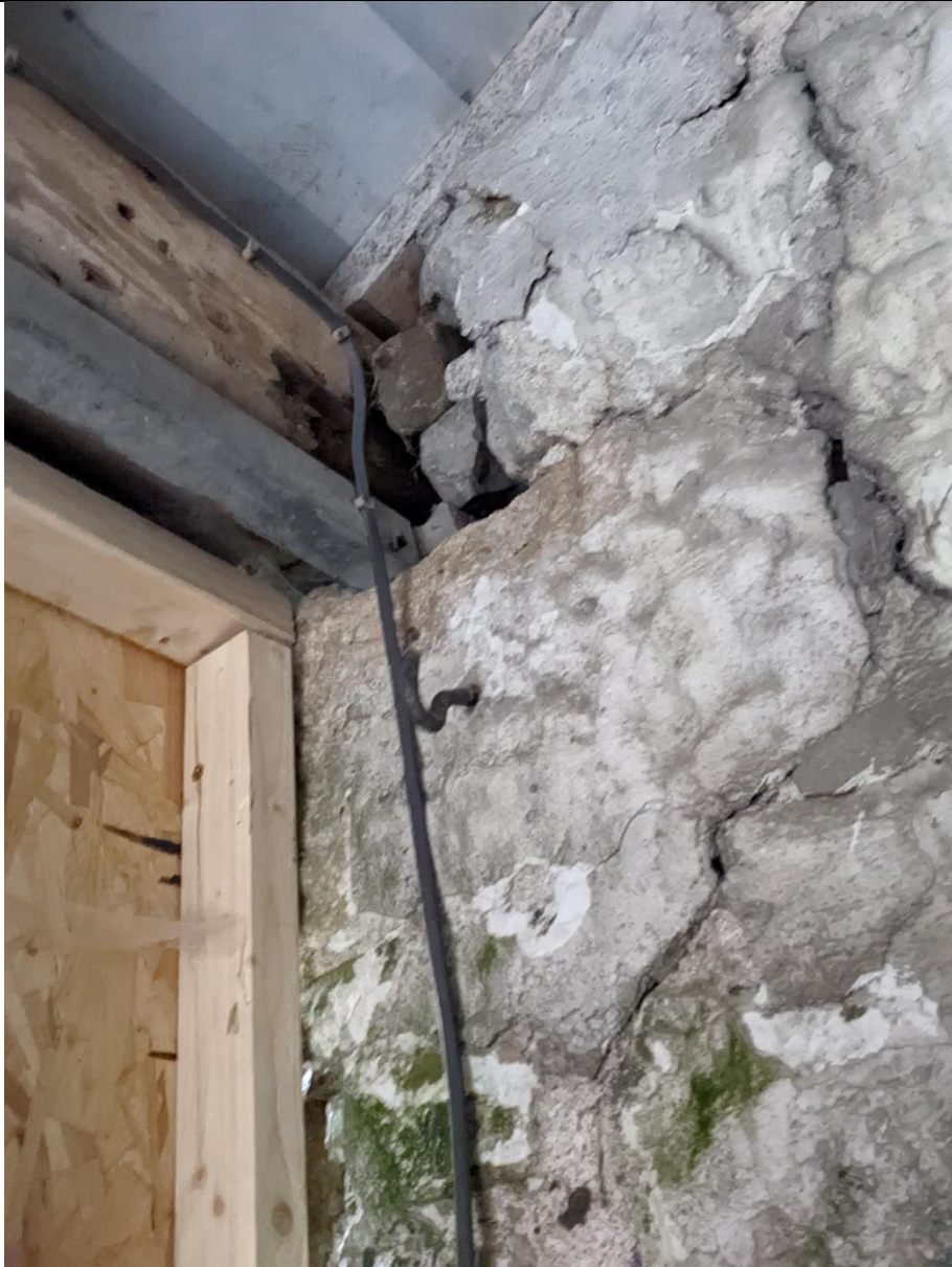
Detail on end of timber lintel at left hand side of wide opening, with timber infill
