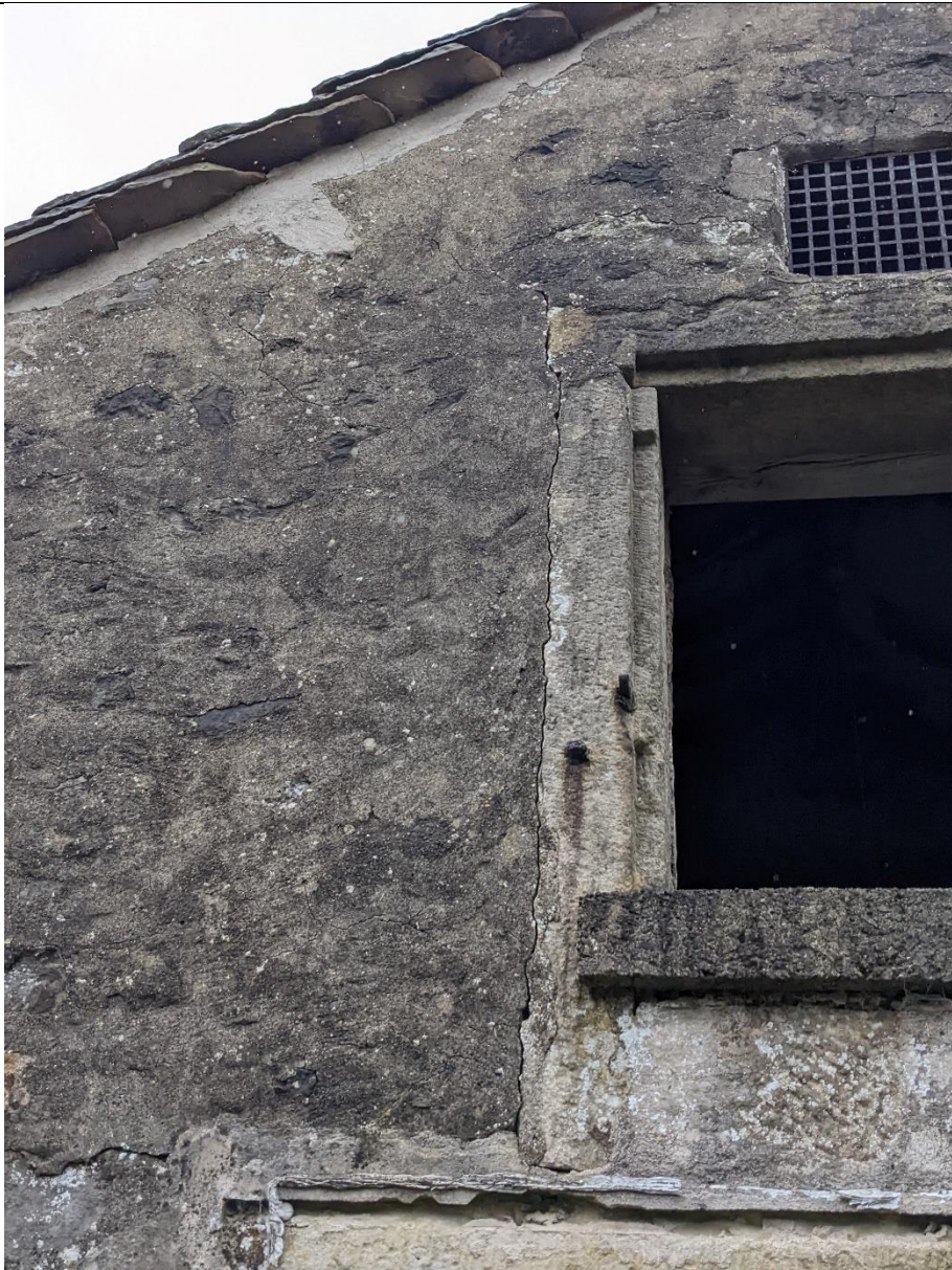
Crack in right hand gable between LH stone jamb and masonry.
