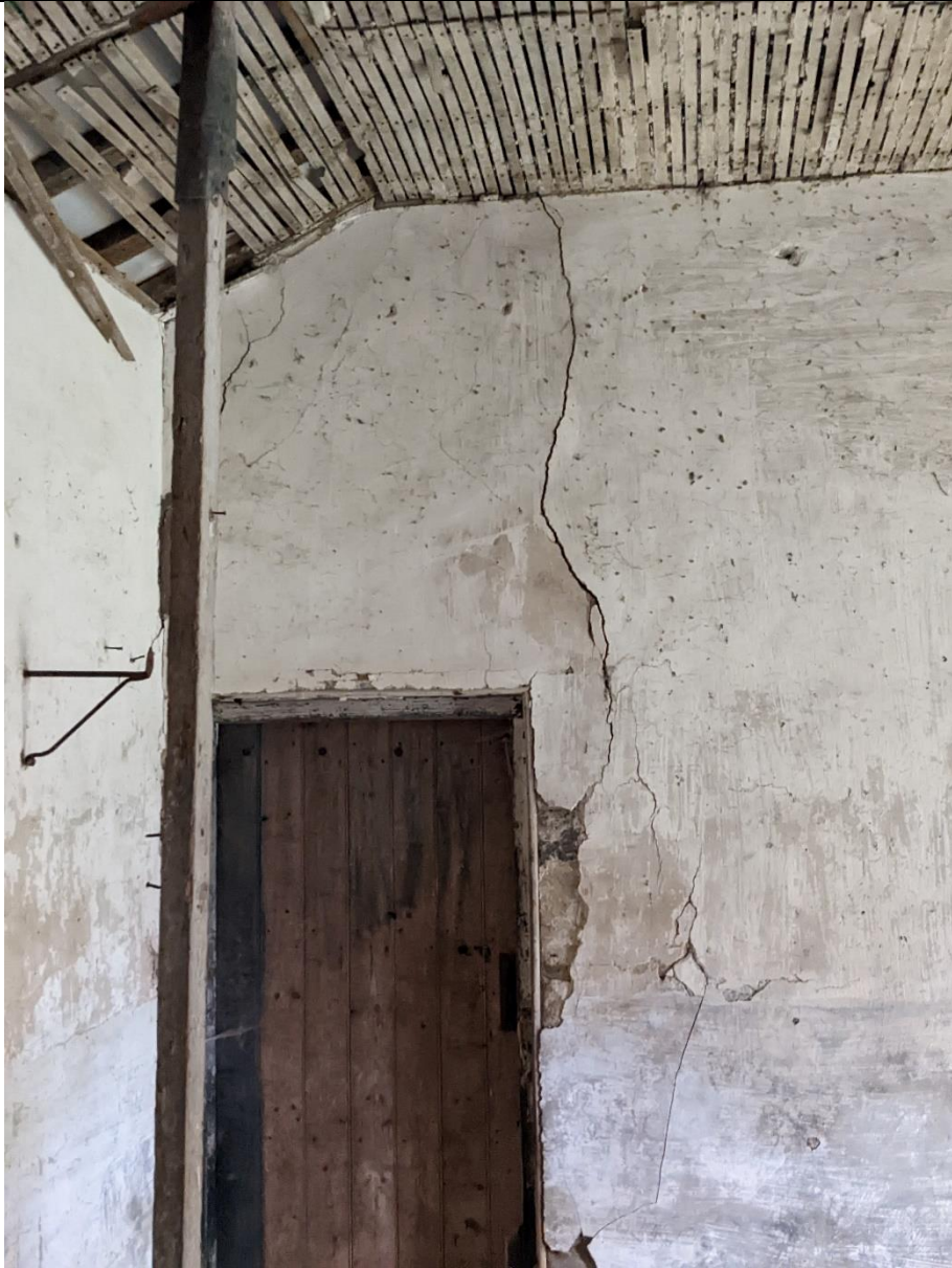
Interior view showing crack in cross wall, emanating from purlin bearing
