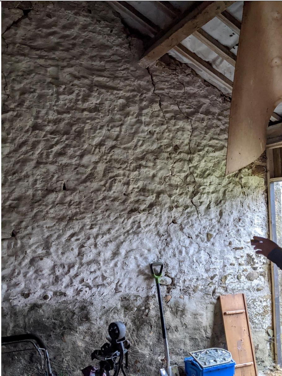
Vertical cracks in cross wall to front, emanating from purlin bearings
