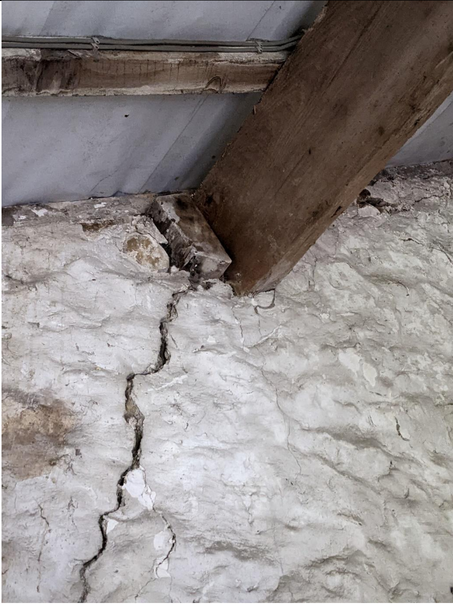
Close up on purlin bearing, showin vistige of old purlin cut end.
