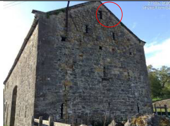
Photograph 4: Ventilation slots and holes in the south eastern gable of Barn 2. Circled is the location of the roost entrance where 6 soprano pipistrelle bats emerged.
