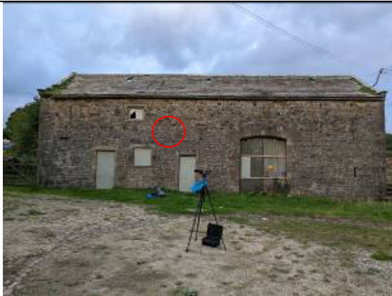
Photograph 3: South western elevation of Barn 2, highlighting the gaps in the stone work above the infilled ventilation slot where one bat emerged.
