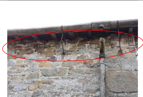
Photograph 2: Example of gaps in mortar work between the stones and access beneath the eaves (circled).
