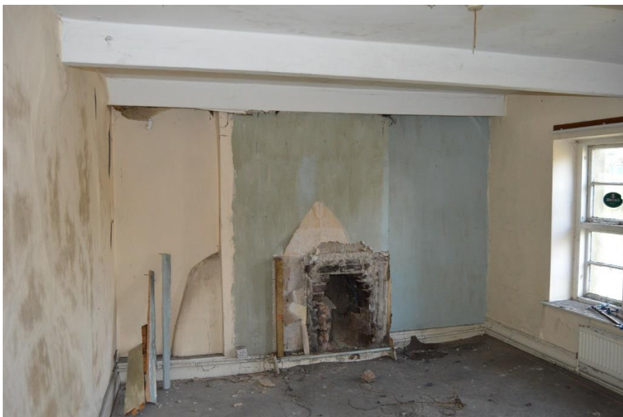
Bedroom 4– No surround present, to be retained and concealed.
