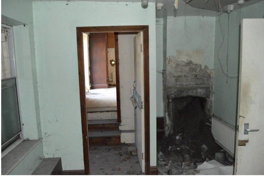
Master Ensuite - No surround present, to be retained and concealed.
