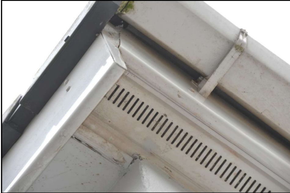
Image showing example of sealed soffit with no potential access for use by birds or bats
