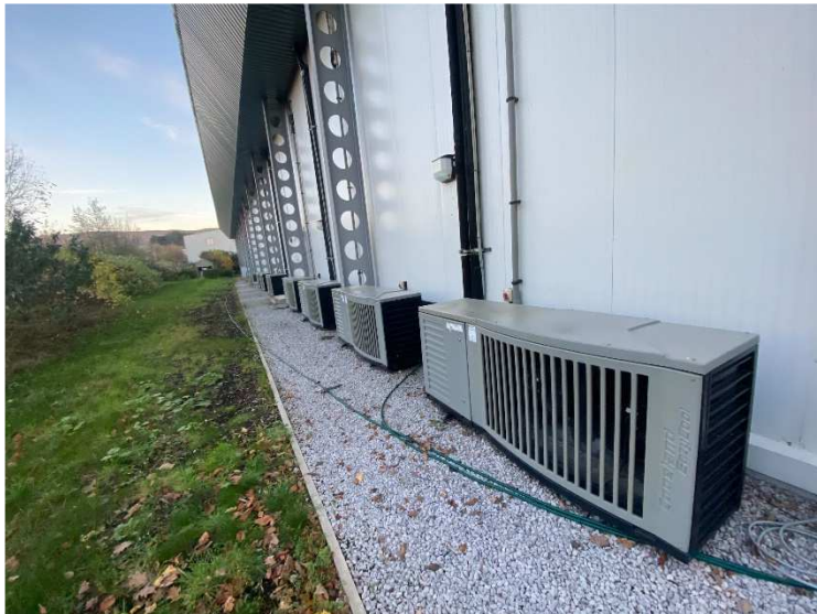
Fixed Plant Items
