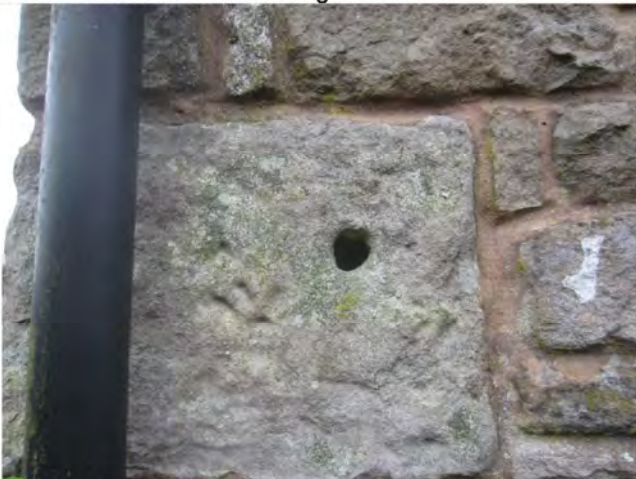
Photo 23: Hole in the western elevation of Building 5
