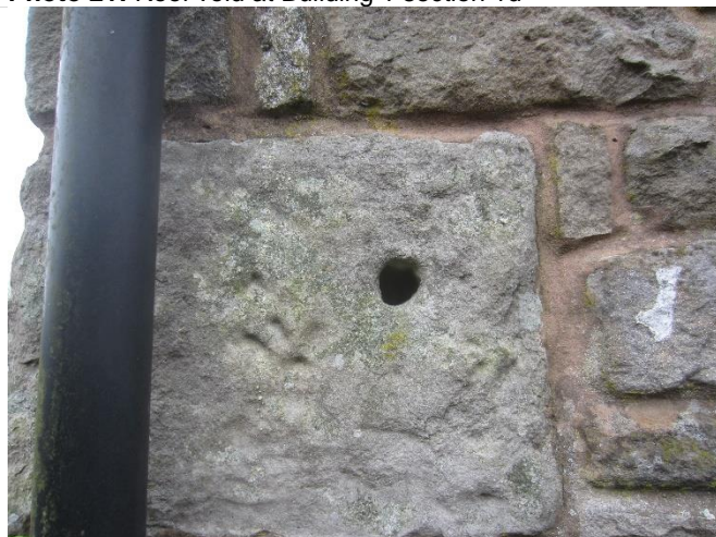
Photo 23: Hole in the western elevation of Building 5
