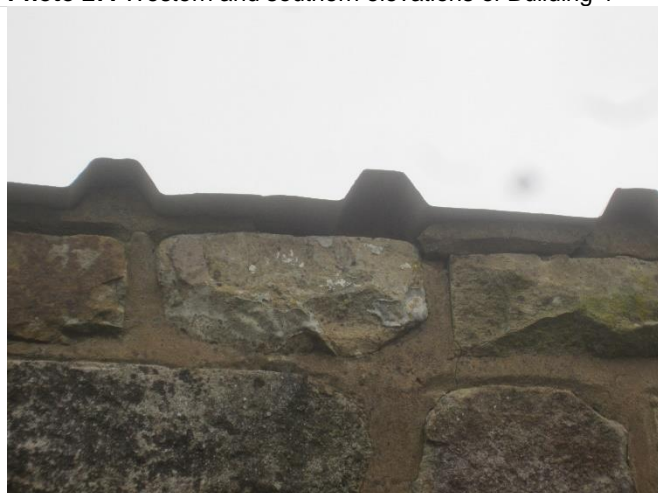
Photo 29: Gaps at the roof line of Building 4; inspected with endoscope
