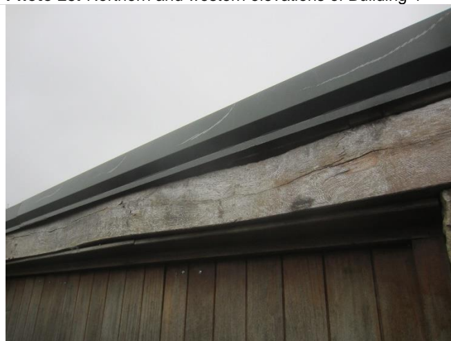
Photo 30: Gap in timber above garage door at Building 4; inspected with endoscope
